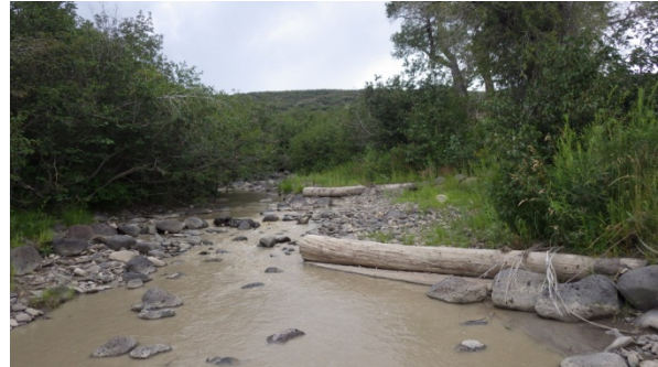
Figure 54: Log vanes at low flow providing bank stabilization and channel narrowing 2 years after construction (Milk Creek, Colorado).
