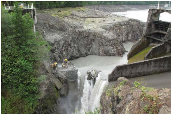
Figure 70: Removal of the lower portion of Glines Canyon Dam, Washington, 7/1/2012 (photo courtesy of the National Park Service).
