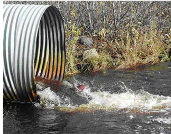
Figure 46: Culvert outlet drop, with Coho.
