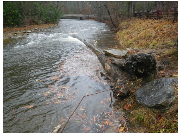
Figure 55: Log J-hook vane providing bank stabilization and pool scour 4 years after construction (Pisgah National Forest, North Carolina; photo credit: Brady Dodd).
