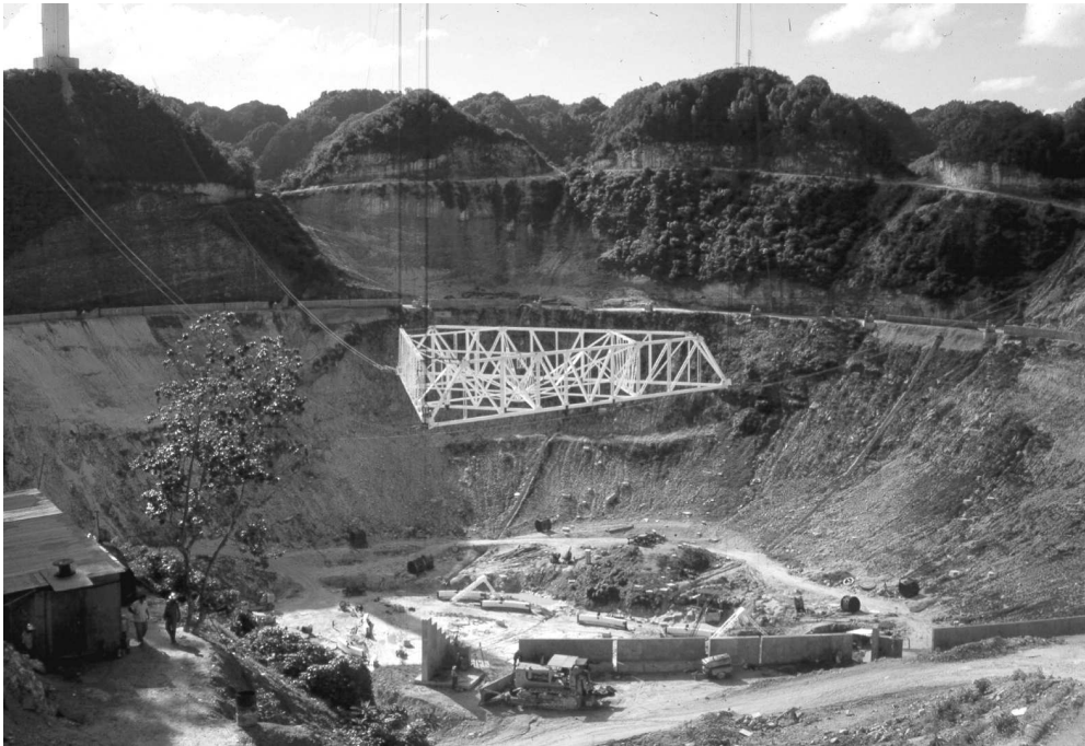
Figure 5. The triangular platform was raised with pulleys attached to auxiliary cables strung between the three towers.
