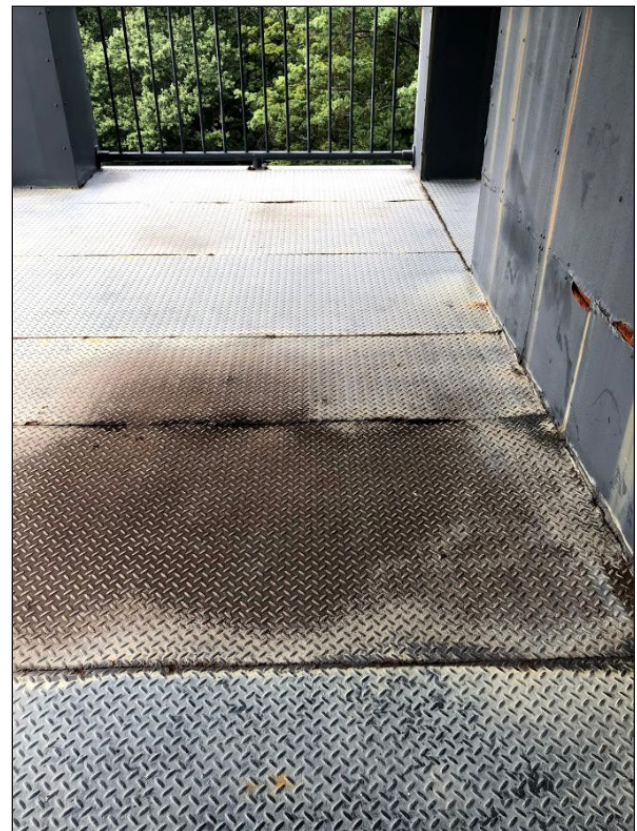
Figure 37. Rust staining at steel seams on observation deck floor, photo by author
