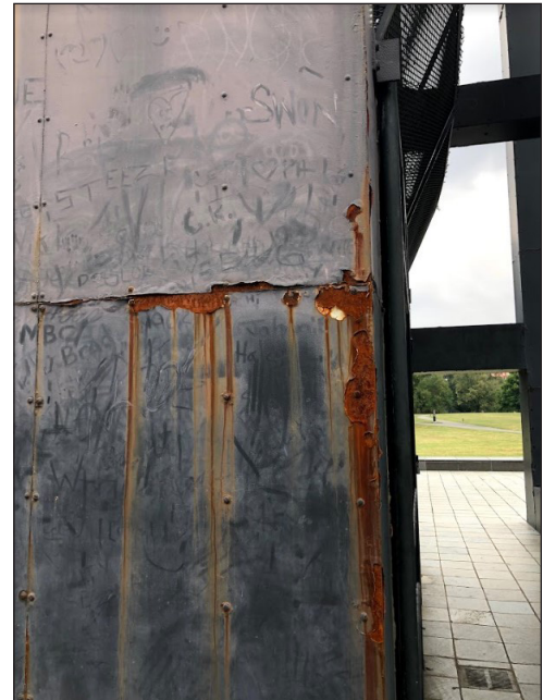
Figure 52. Corrosion along panel edge
