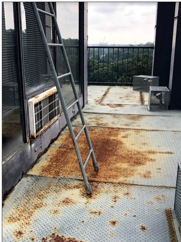
Figure 72. Rust staining to flooring due to moisture from AC unit (2019), photo by author
