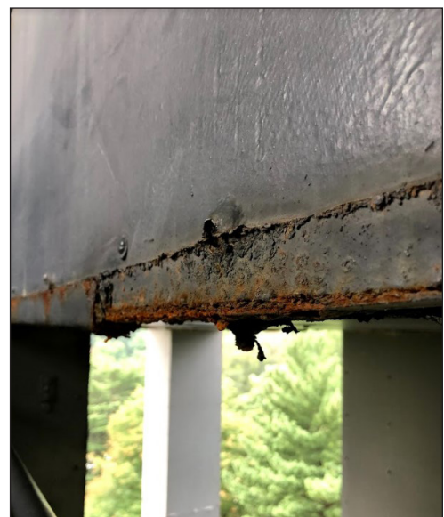
Figure 54. Corrosion underneath panel
