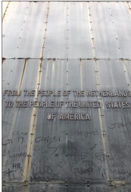
Figure 51. Rust staining along panels
