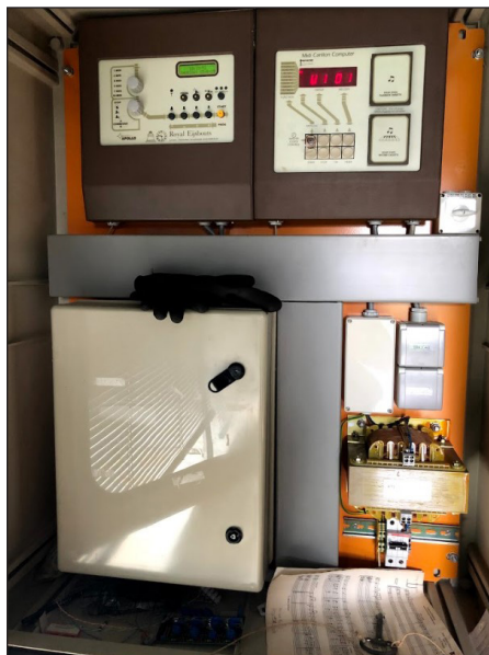
Figure 74. Electrical Panel in Clavier Playing Chamber (2019), photo by author
