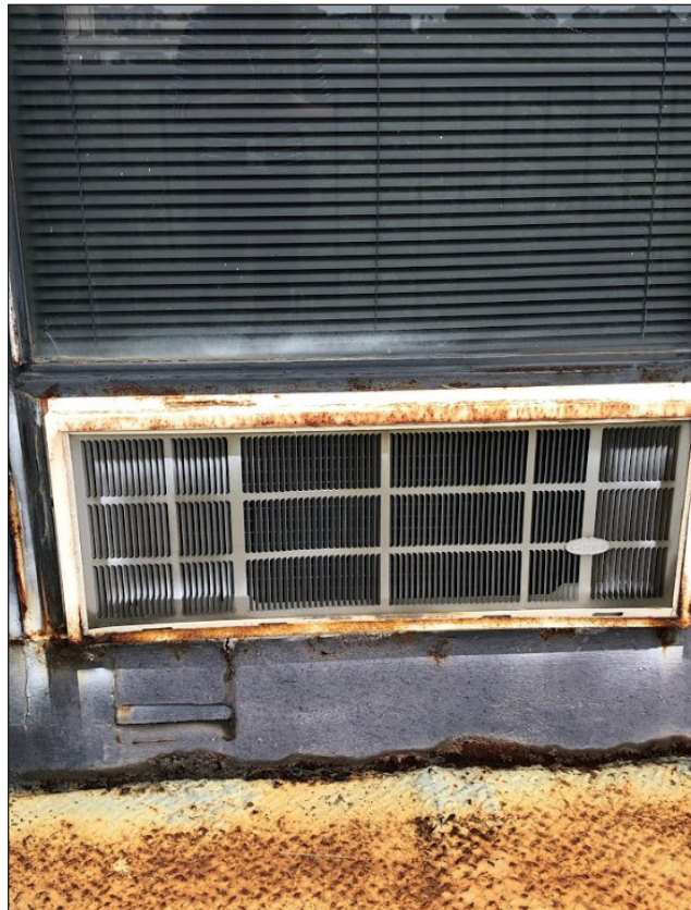
Figure 73. Rust staining under the exterior of the AC unit (2019), photo by author
