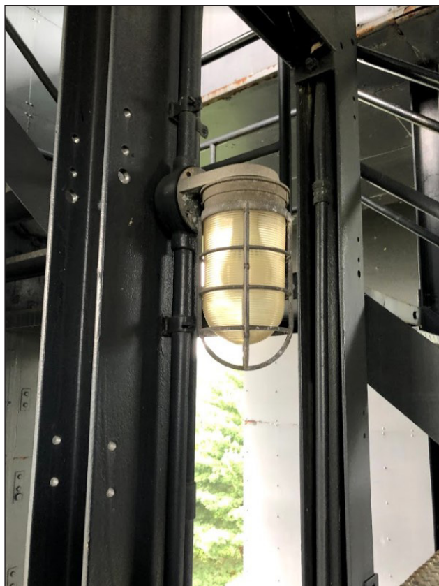
Figure 76. Light fixture in interior stairwell (2019), photo by author
