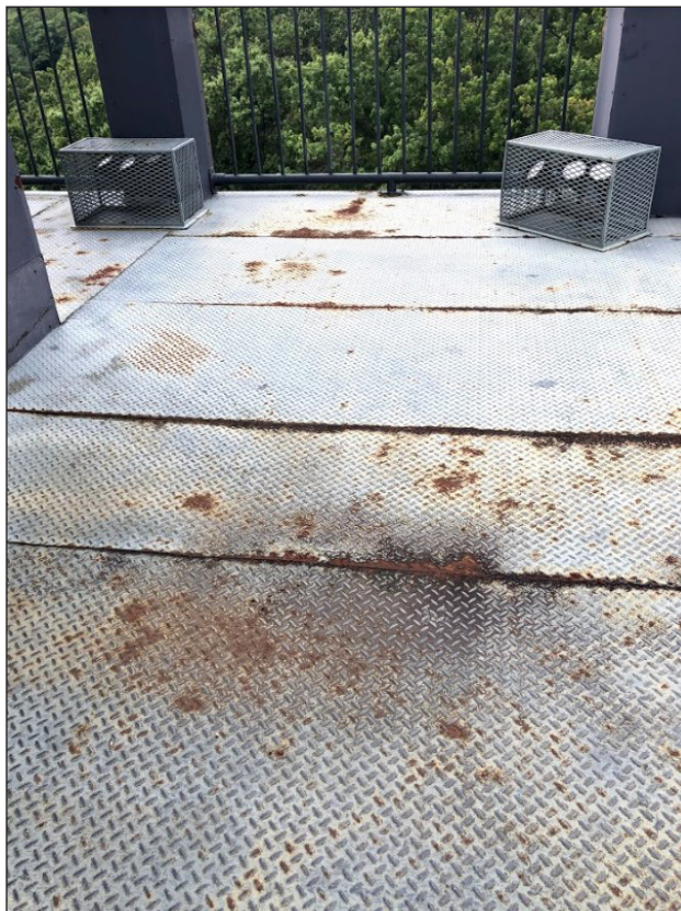
Figure 36. Rust staining at steel seams on observation deck floor, photo by author
