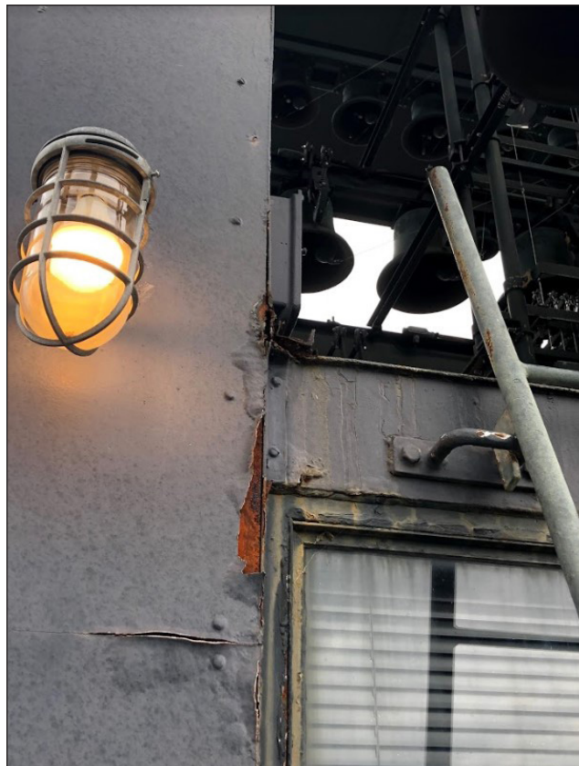
Figure 77. Functioning light fixture on the exterior of the clavier playing chamber on the second observation deck (2019), photo by author
