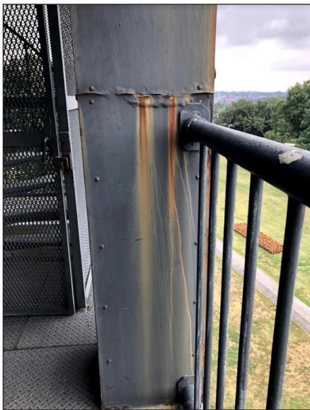
Figure 49. Rust staining on steel column
