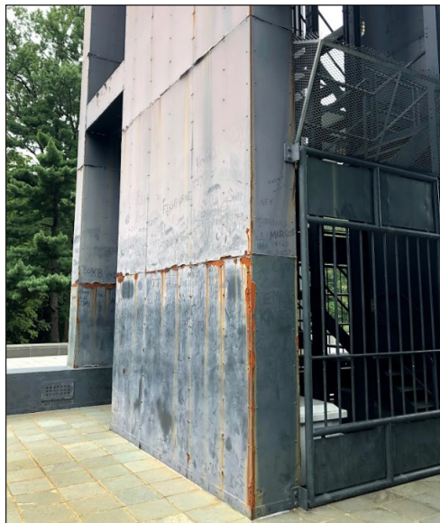
Figure 50. Corrosion along steel edges
