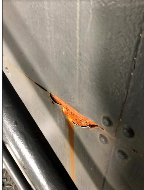
Figure 48. Rust on Steel Panels
