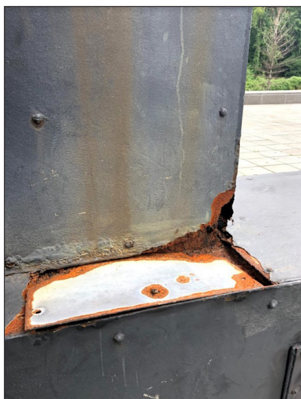
Figure 53. Corrosion along steel beam corner
