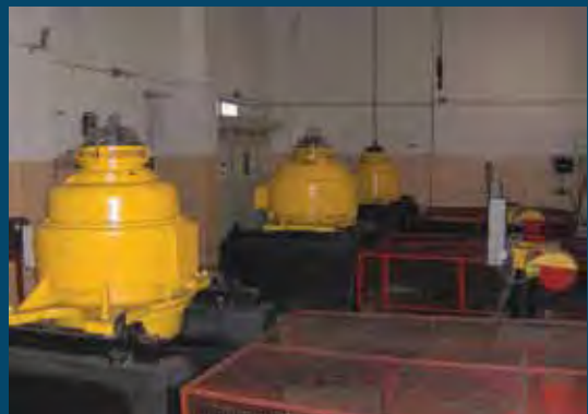
HE pastate Inside powerhouse
