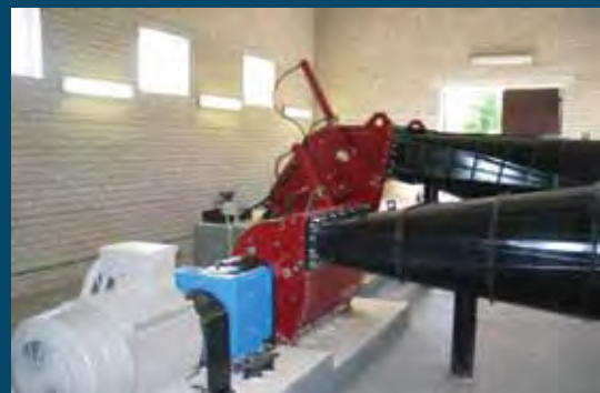
HE pastate Inside powerhouse
