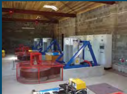
HE pastate Inside powerhouse
