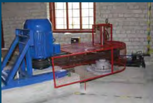
HE pastate Inside powerhouse
