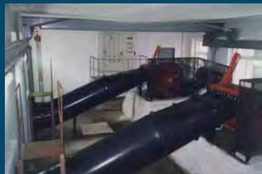
HE pastate Inside powerhouse
