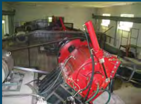
HE pastate Inside powerhouse
