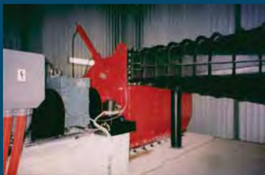
HE pastate Inside powerhouse
