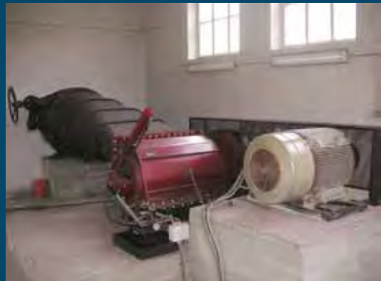
HE pastate Inside powerhouse
