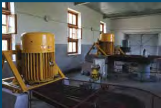
HE pastate Inside powerhouse
