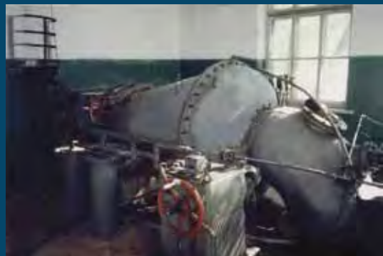
HE pastate Inside powerhouse
