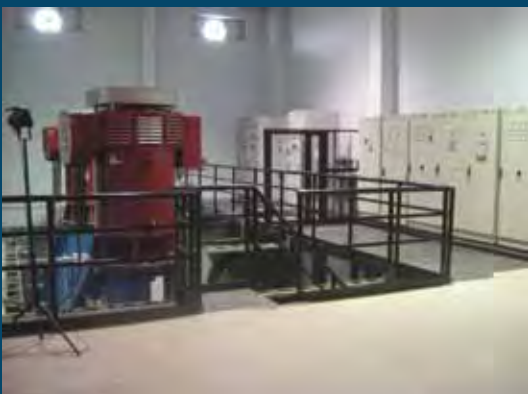
HE pastate Inside powerhouse
