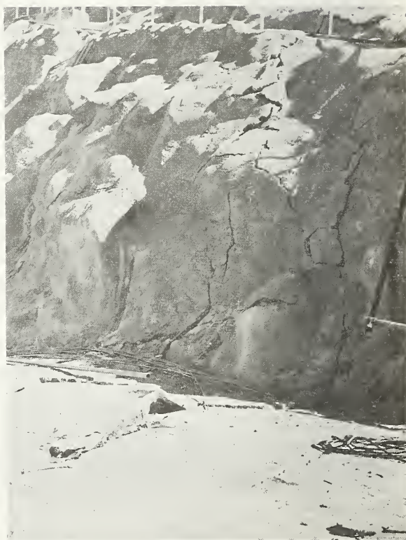
Figure 8.28 Cracks in gunite, left abutment downstream of Pacoima Dam.
