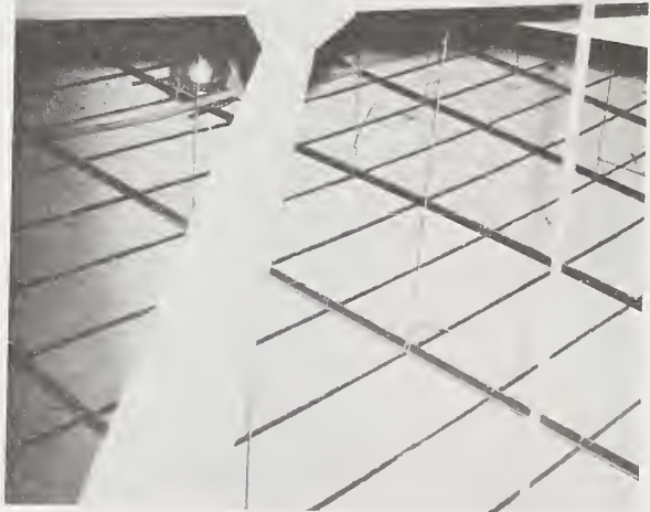
Figure 6.21 Buckled 5 x 3 angle brace, San Fernando High School.
