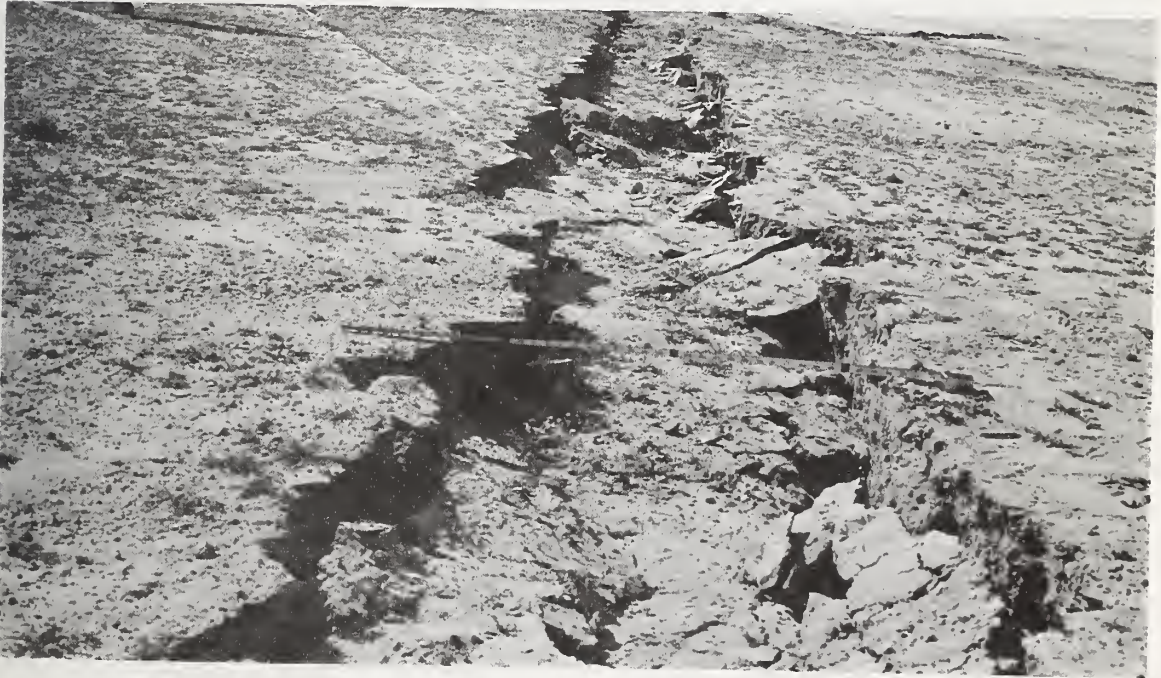
Figure 7.38 Ground cave-in (2-ft wide) near the damaged road slabs shown in figure 7.35.
