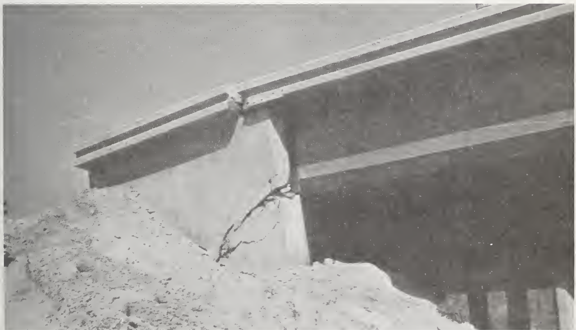
Figure 7.29 Typical abutment damage.
