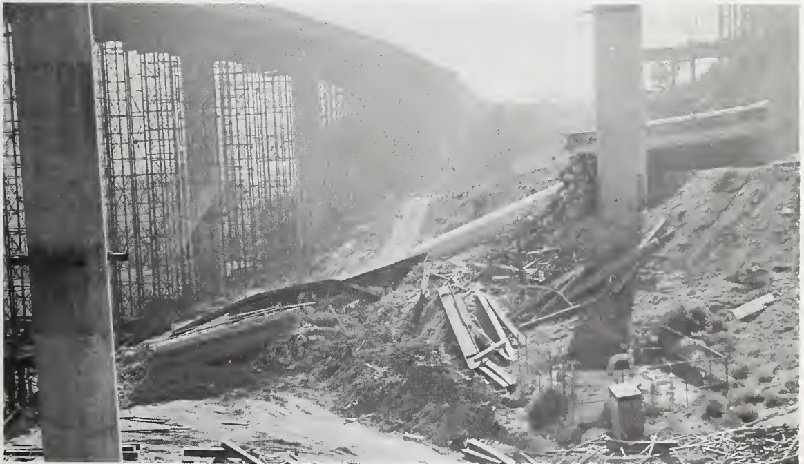
Figure 7.7 Debris from the South Connector Overcrossing.
