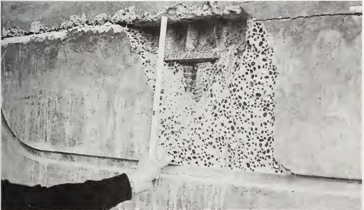
Figure 5.177 Damage to the exterior surface of the concrete wall along the construction joint.
