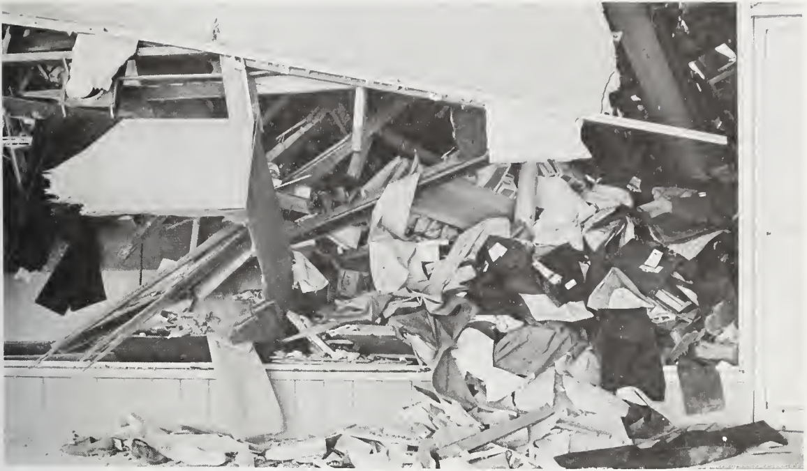
Figure 5.140 The wall of the building shown in figure 5.139 fell through the roof of this building.
