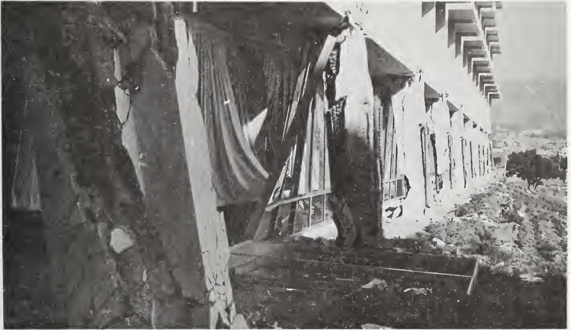
Figure 5.26 South row of first story columns, in Wing D; note the lack of ties on the corner bars which have broken out of the columns.
