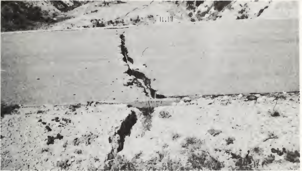
Figure 8.30 Looking northwesterly toward basin showing crack in the pavement and a 2-inch vertical displacement of paved crest of dam (Stetson Debris Basin).
