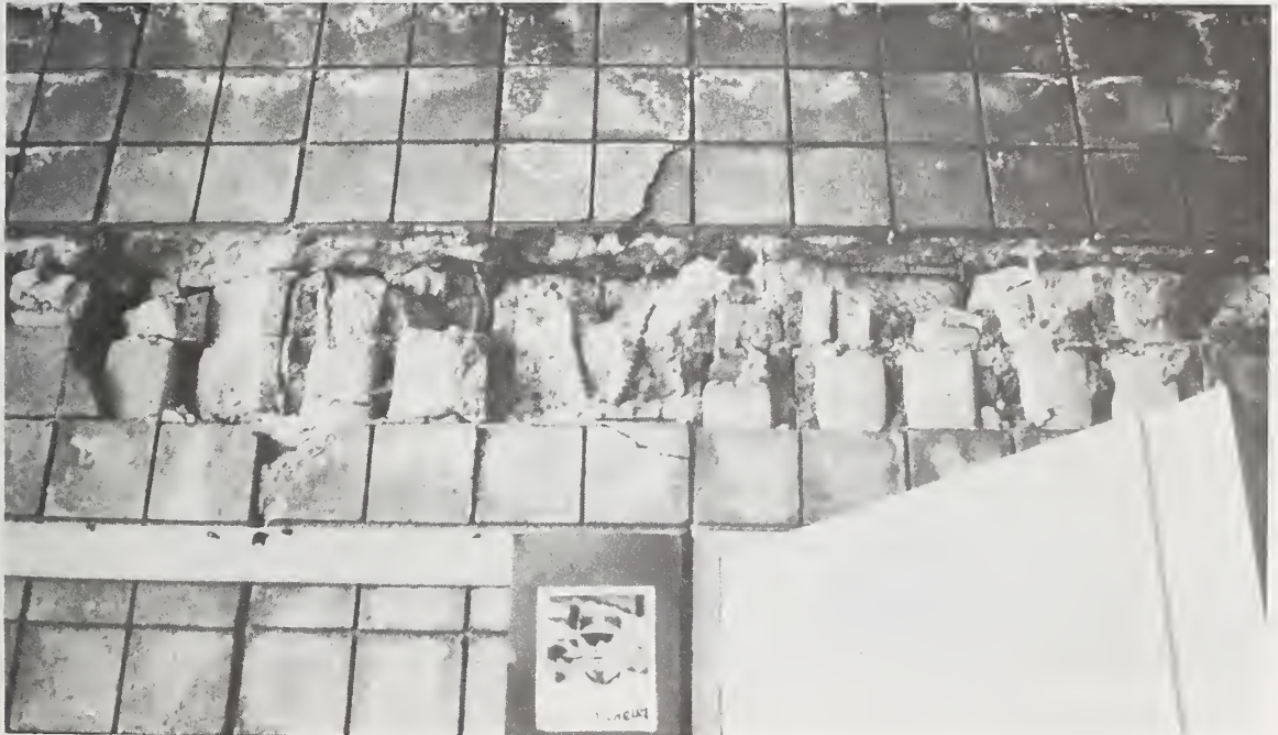
Figure 6.50 Damage to wall at change in roof elevation (interior), Los Angeles County Juvenile Facility.
