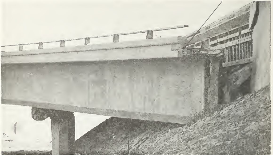
Figure 7.22 Abutment and pier damage at the western end of the Northwest Connector Overcrossing.
