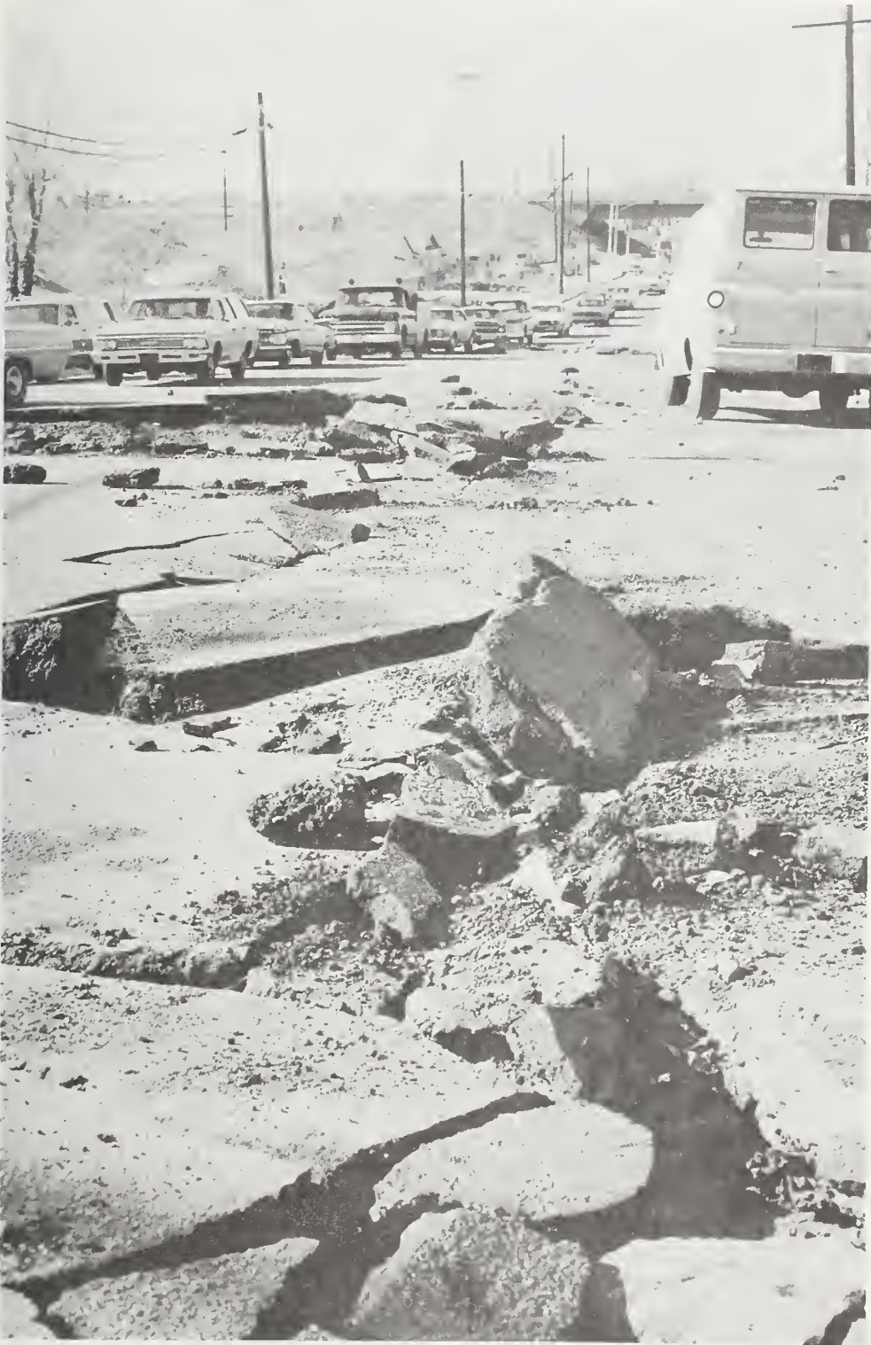
Figure 7.43 Buckled street in Sylmar near Harding Elementary School. (Los Angeles Times Photo.)
