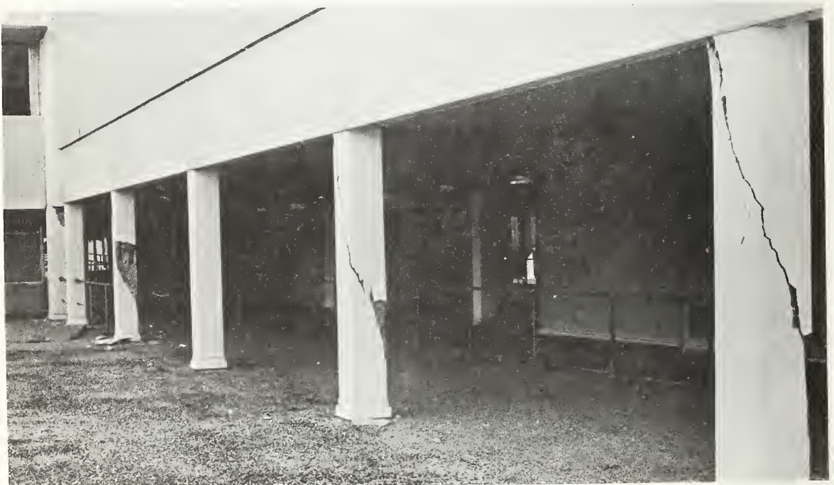
Figure 5.74 Torsional cracking of second-story columns in the north wing.
