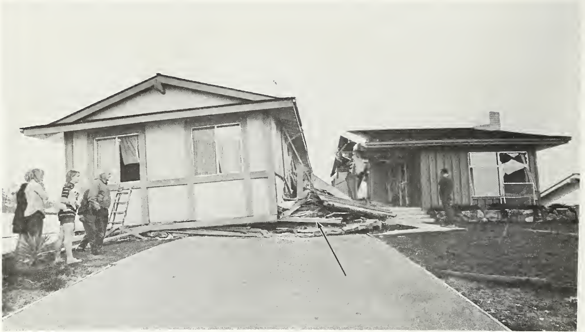
Figure 5.162 Split-level residence, Sylmar. Note crushed car (arrow). (Los Angeles Times Photo).
