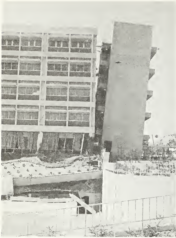
Figure 5.34 Tipped stair tower at the end of Wing C. This is the only stair tower that did not topple. This stair tower is supported directly on the foundation; whereas, the other three towers were supported on the ground-story columns.
