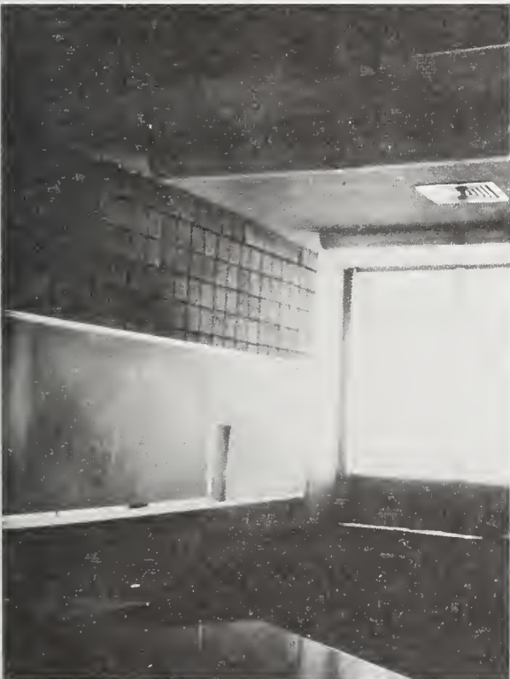
Figure 6.45 Displacement of concrete block at top of transverse partition, Los Angeles County Juvenile Facility.
