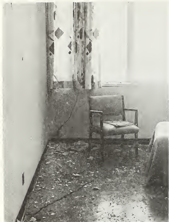
Figure 5.67 Damaged northwest corner room on the third floor. Note shear wall, floor, and spandrel cracking.
