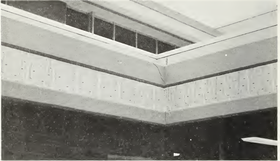
Figure 5.88 Cracking in exterior roof beams of the Mental Health Center.
