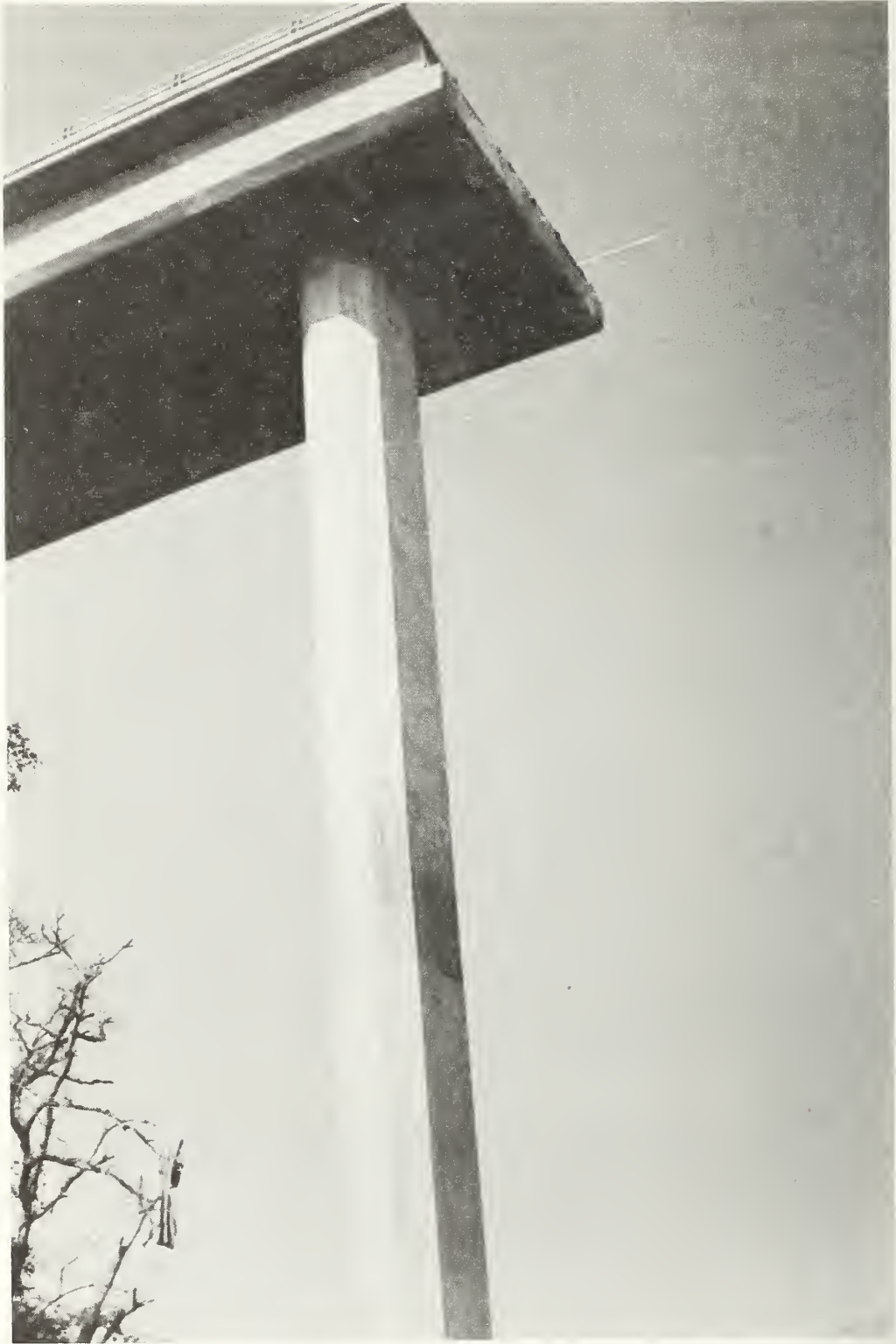
Figure 7.5 Post-failure view of Pier 5 and hinge seat.
