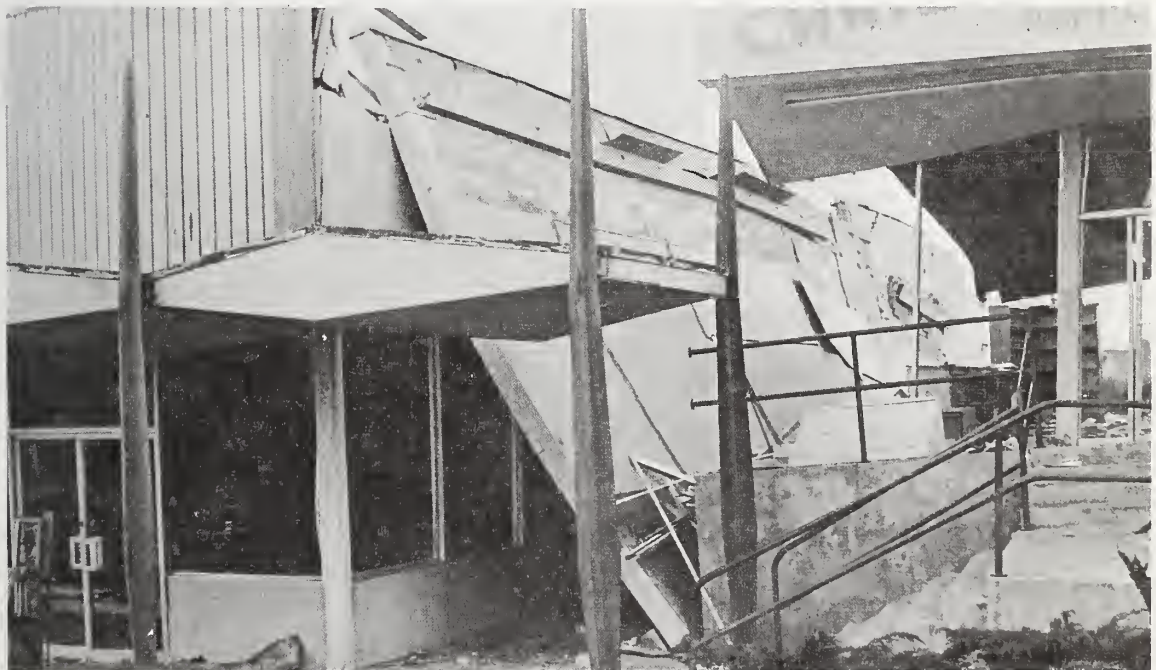
Figure 5.133 Collapsed side wall of a small store in the shopping center.
