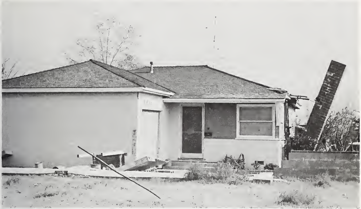
Figure 5.164 Leaning reinforced brick masonry chimney.
