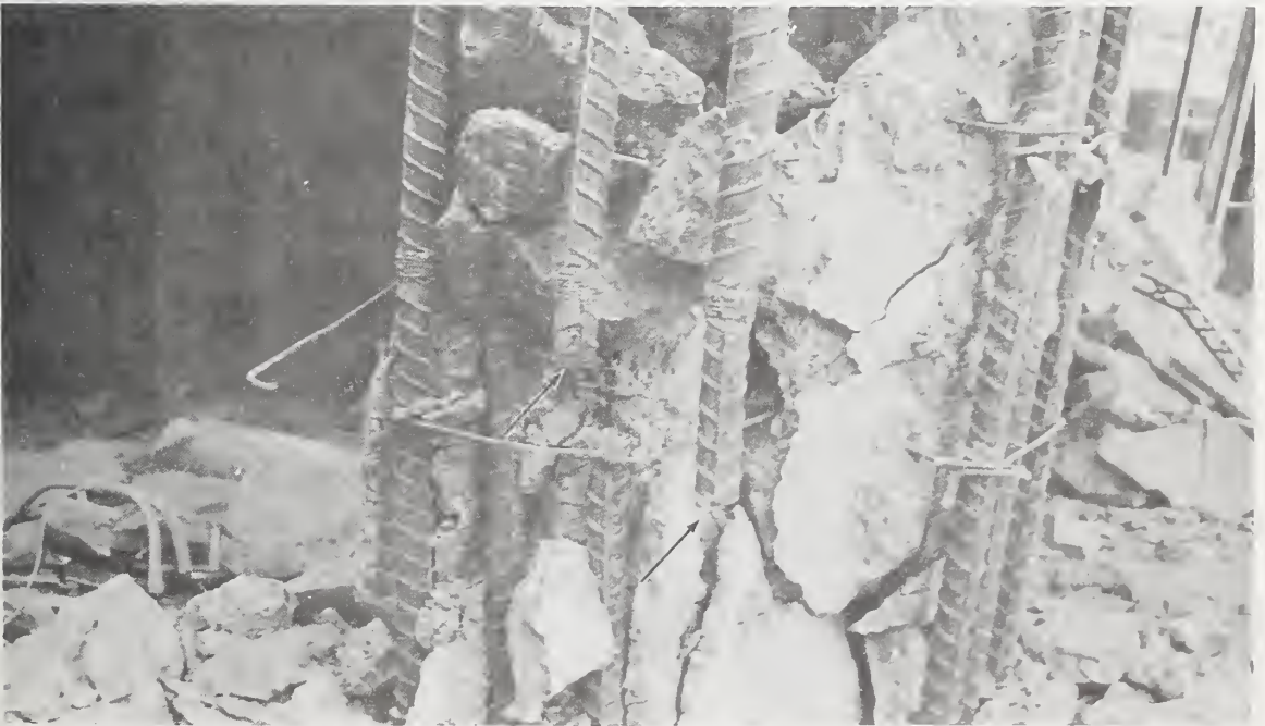
Figure 5.21 Close-up view of the first story column in the northeast corner of Wing B. Note the two fractured main reinforcing bars (arrows) and broken ties.
