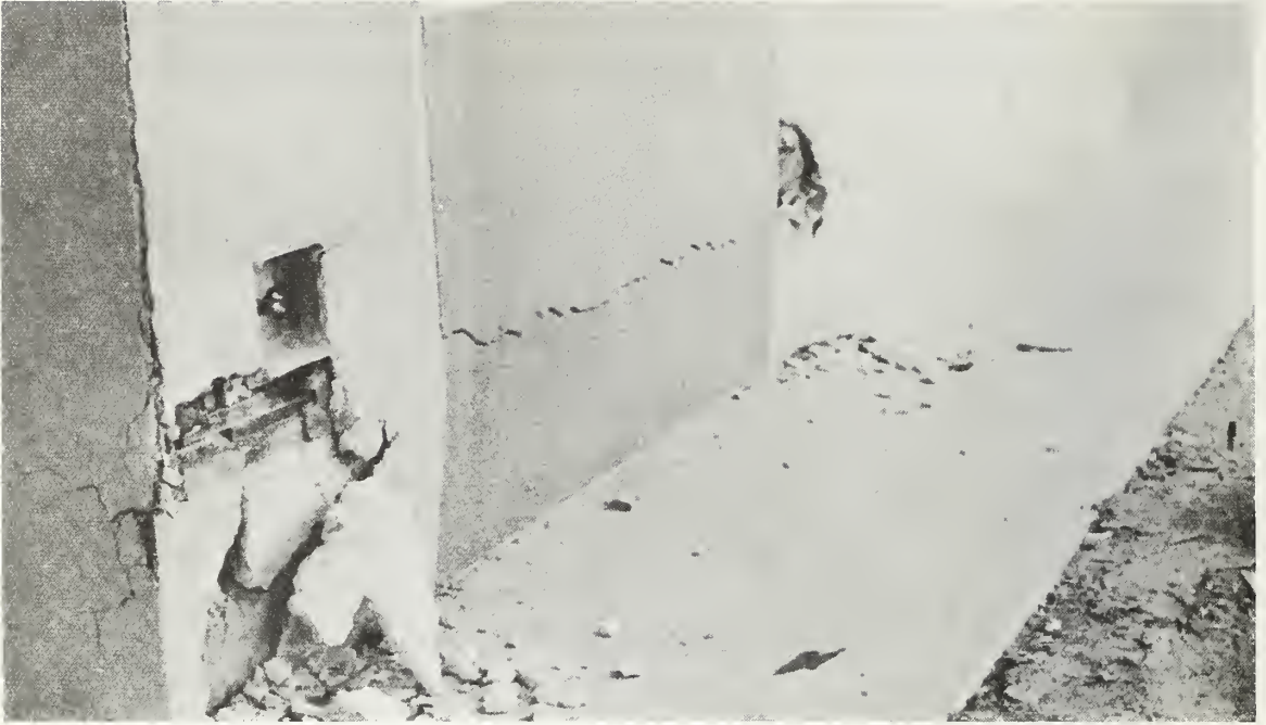
Figure 6.12 Displaced bearing wall, Van Gogh Street School.
