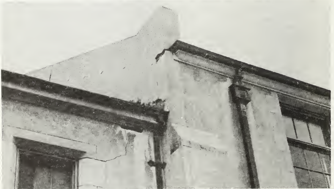
Figure 6.5 Brick walls sustained serious cracking, Morningside School Building #2.
