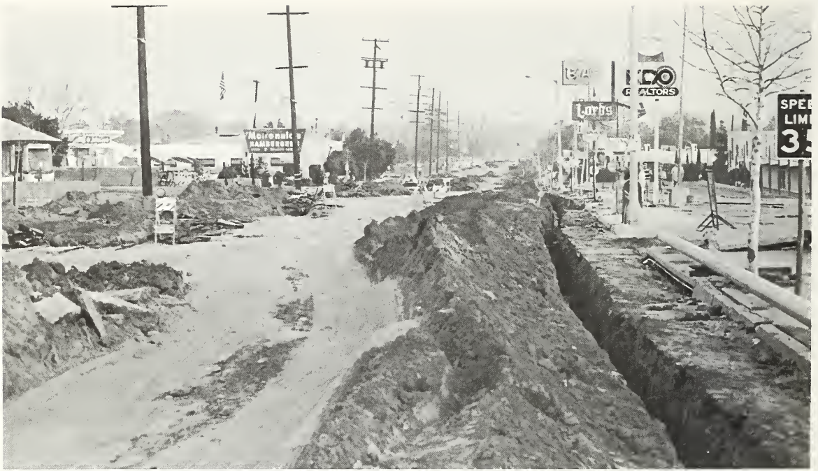
Figure 7.39 Broken gas, water, and sewer lines being repaired near intersection of Hubbard Avenue and Glenoaks Boulevard, San Fernando.
