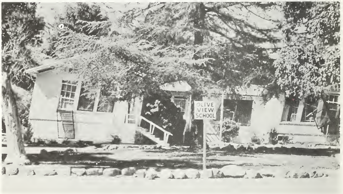
Figure 5.40b Severely damaged pre-1933 wood-frame structure at the old section of the Olive View Medical Center.
