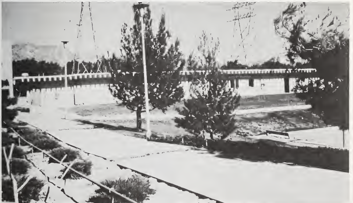
Figure 6.41 West wall of girls' school, Los Angeles County Juvenile Facility. Note displacement at left (north) end of building and severe ground rupture (see figure 6.48).
