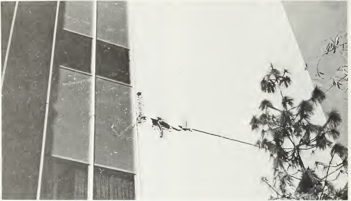
Figure 5.104 Buckled vertical reinforcement in southeast shear wall.
