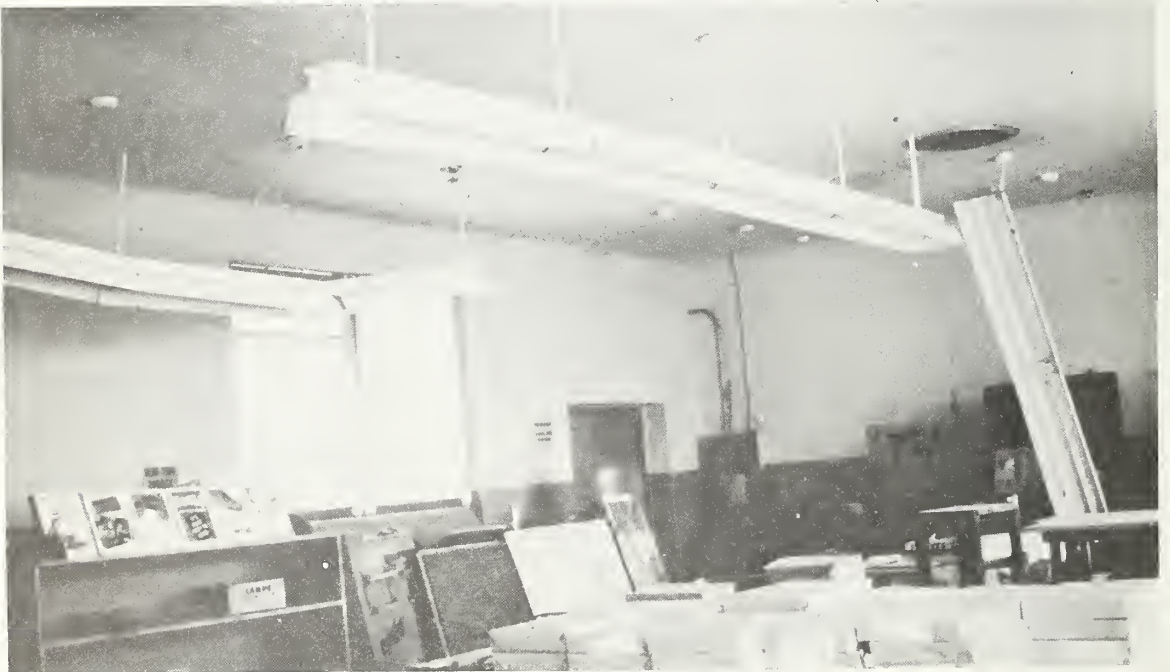
Figure 6.60 Stem mounted lighting fixtures were severely damaged, Camp Karl Holton.
