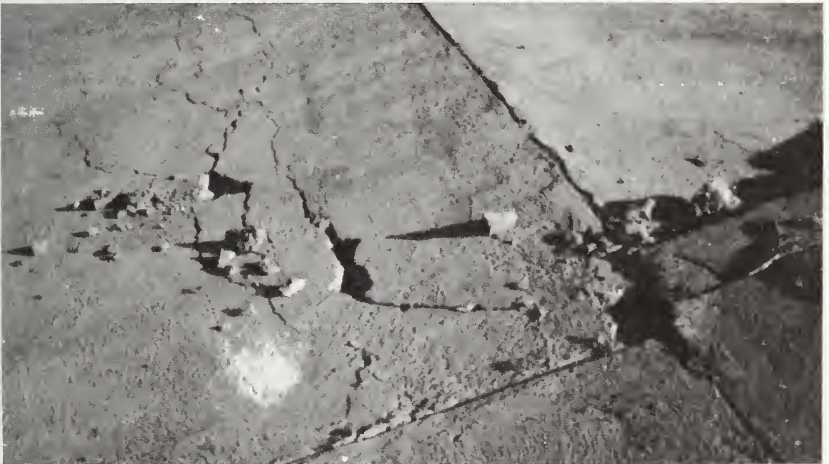
Figure 8.31 Looking easterly showing damage to facing slab; Stetson Debris Basin.
