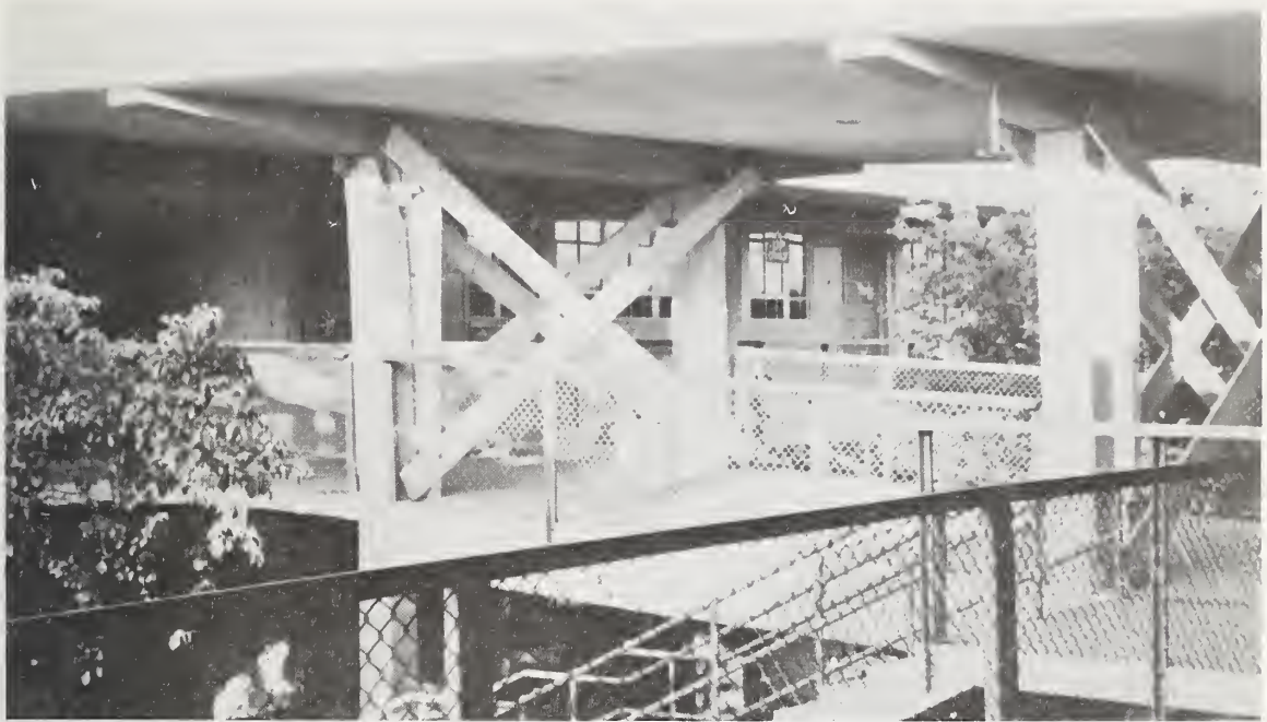
Figure 6.22 Fractured concrete at second-story covered arcade columns, Patrick Henry Jr. High School.
