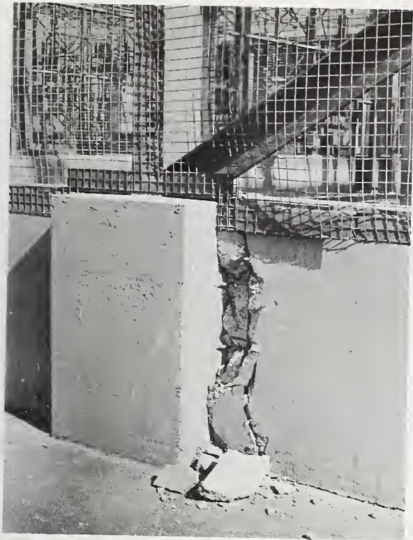
Figure 8.12 Concrete spalling at one of the joints between a column pedestal and an enclosure wall surrounding the electrical transformer yard.
