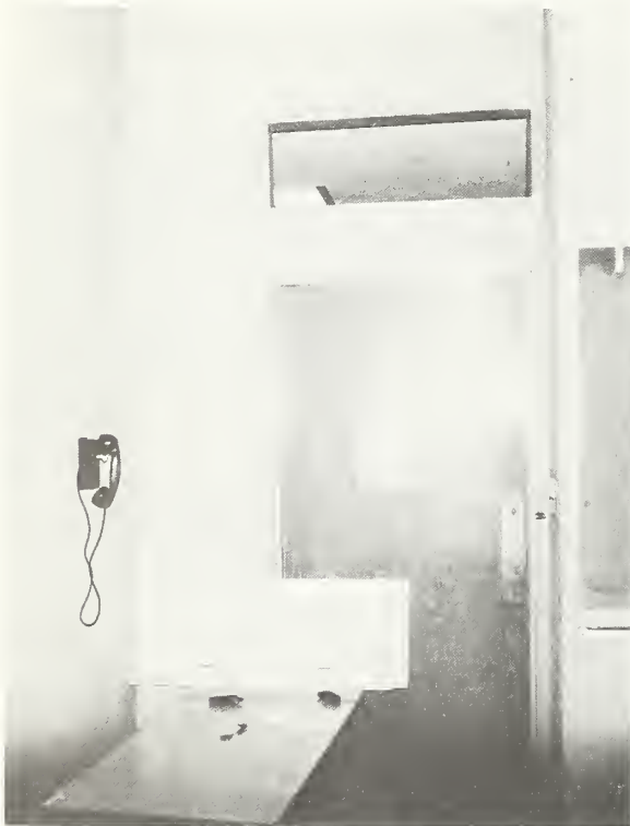
Figure 6.33 Ventilating louvers pulled loose from corridor wall above classroom doors (louver placed on table for photo), Crescenta Valley High School.
