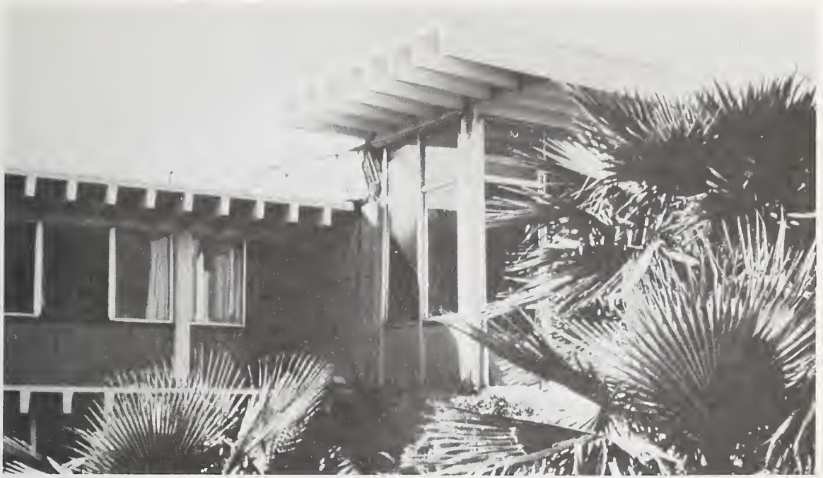
Figure 6.49 Damage to wall at change in roof elevation (exterior), Los Angeles County Juvenile Facility.
