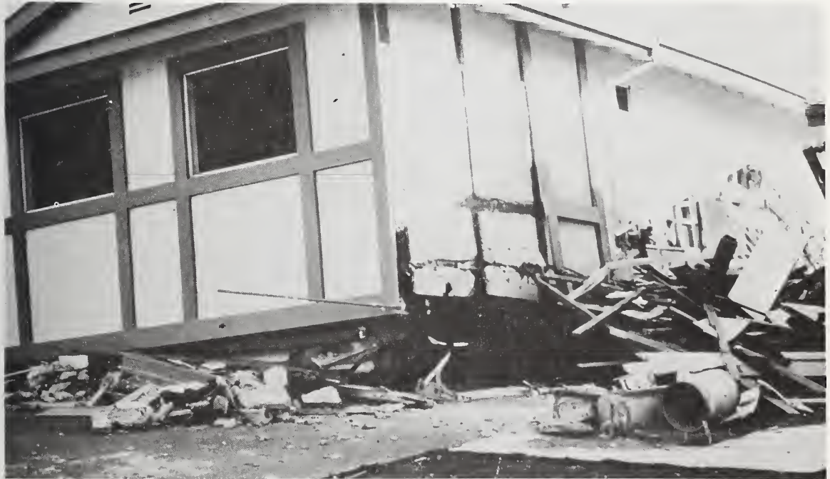
Figure 5.157 Collapsed split-level residence at Fenton Avenue and Tyler Street.
