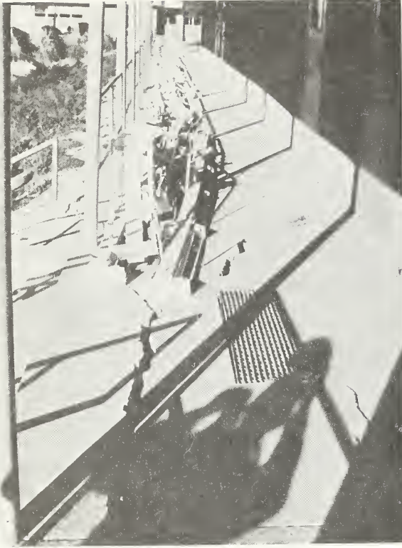
Figure 6.59 Arcade pipe columns were displaced at base where slab on grade pulled apart, Camp Karl Holton. (Damaged lighting fixtures were removed from buildings and stored on walkway.)
