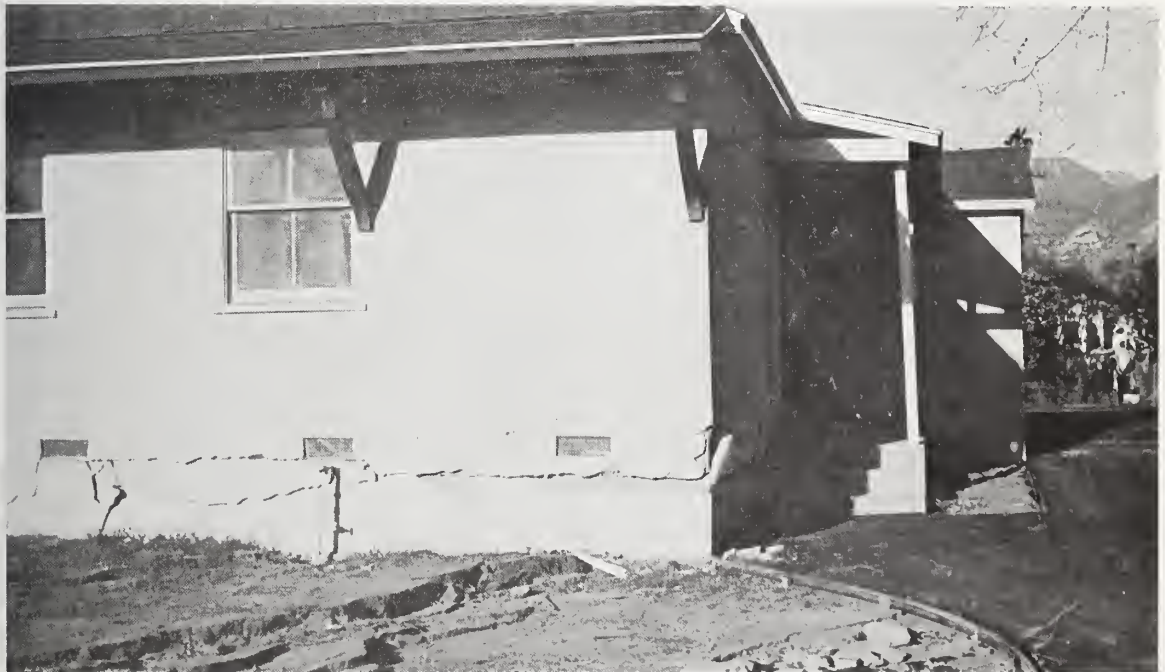
Figure 5.165 Wood-frame and stucco house on 8th Street, San Fernando. Horizontal cracking occurred along the top of the foundation wall. Note ground cracking in left foreground.
