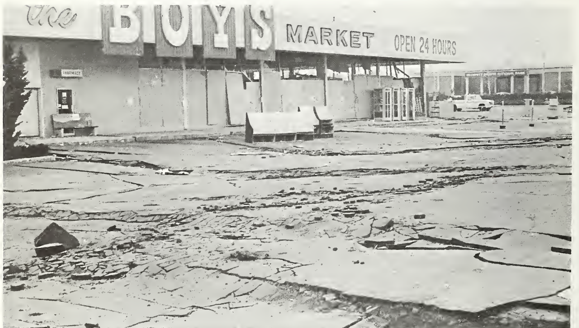
Figure 7.40 Considerable ground movement is evident in the parking lot of the shopping center at the corner of Hubbard Avenue and Glenoaks Boulevard.
