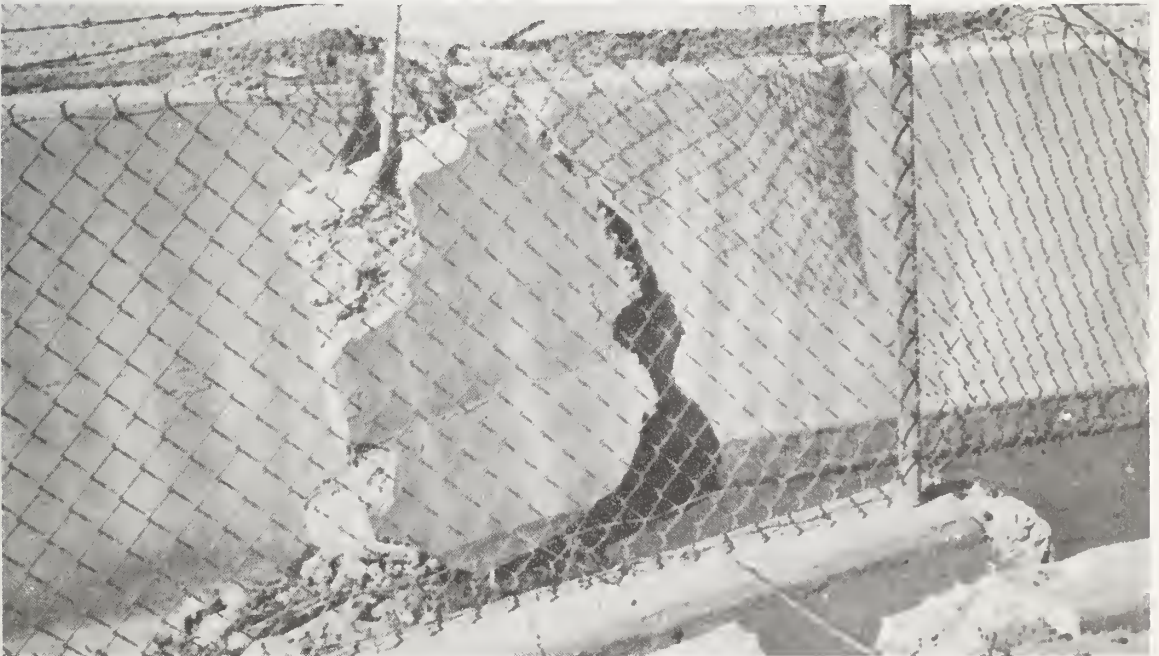
Figure 8.35 Lopez Canyon Channel. A 2-foot displacement of the channel had caused complete failure of the walls and invert, with the upstream portion moving over the downstream portion.
