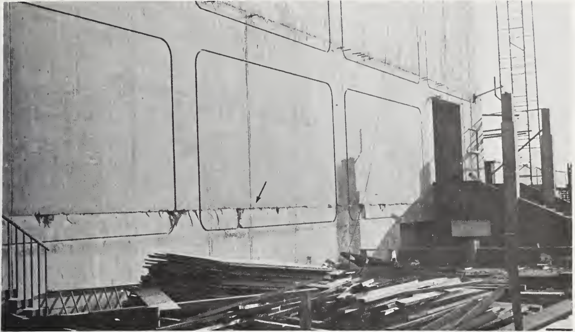
Figure 5.176 Horizontal crack along the construction joint at the base of the structure.
