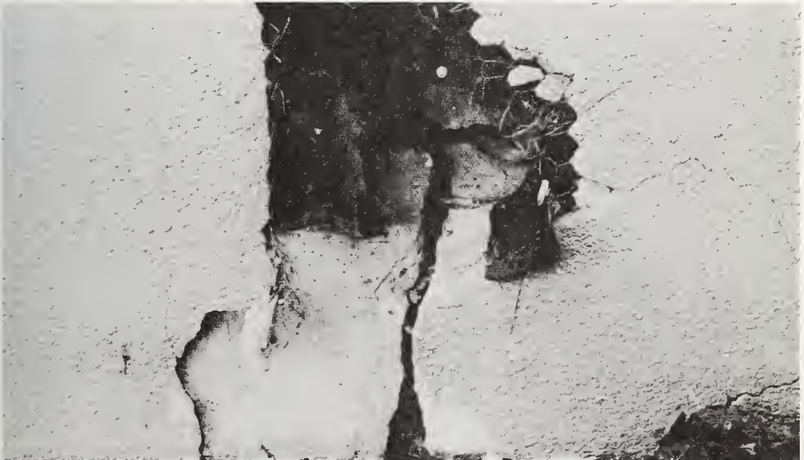
Figure 6.11 Fractured concrete foundation wall, Van Gogh Street School.
