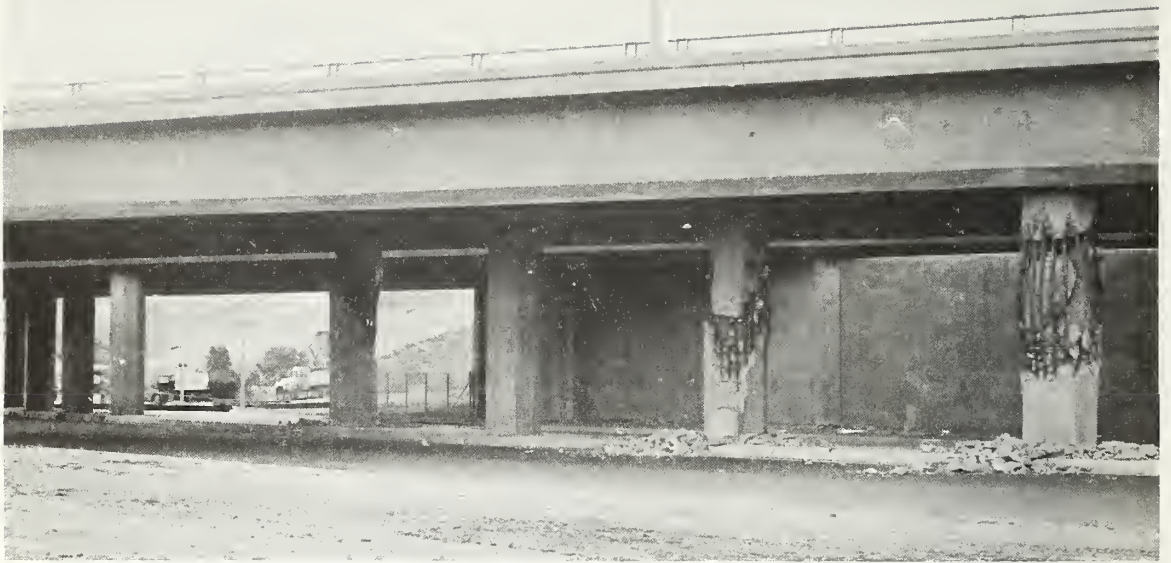
Figure 7.26 Column failures in bent 3 of Foothill Boulevard Undercrossing.
