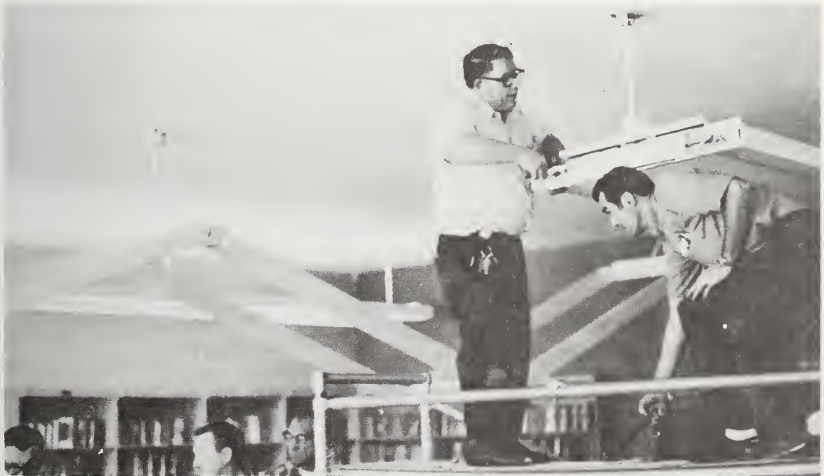
Figure 6.35 Damage to lighting fixtures at Clark Junior High School.
