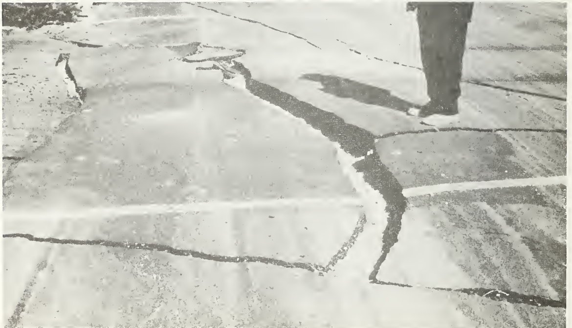
Figure 6.54 Extensive cracking of parking lot pavement, Camp Karl Holton.
