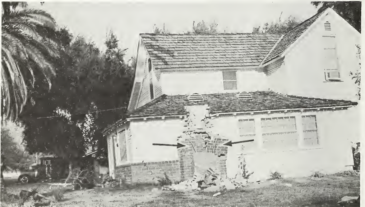
Figure 5.163 Damaged reinforced brick masonry chimney (arrows indicate reinforcement).
