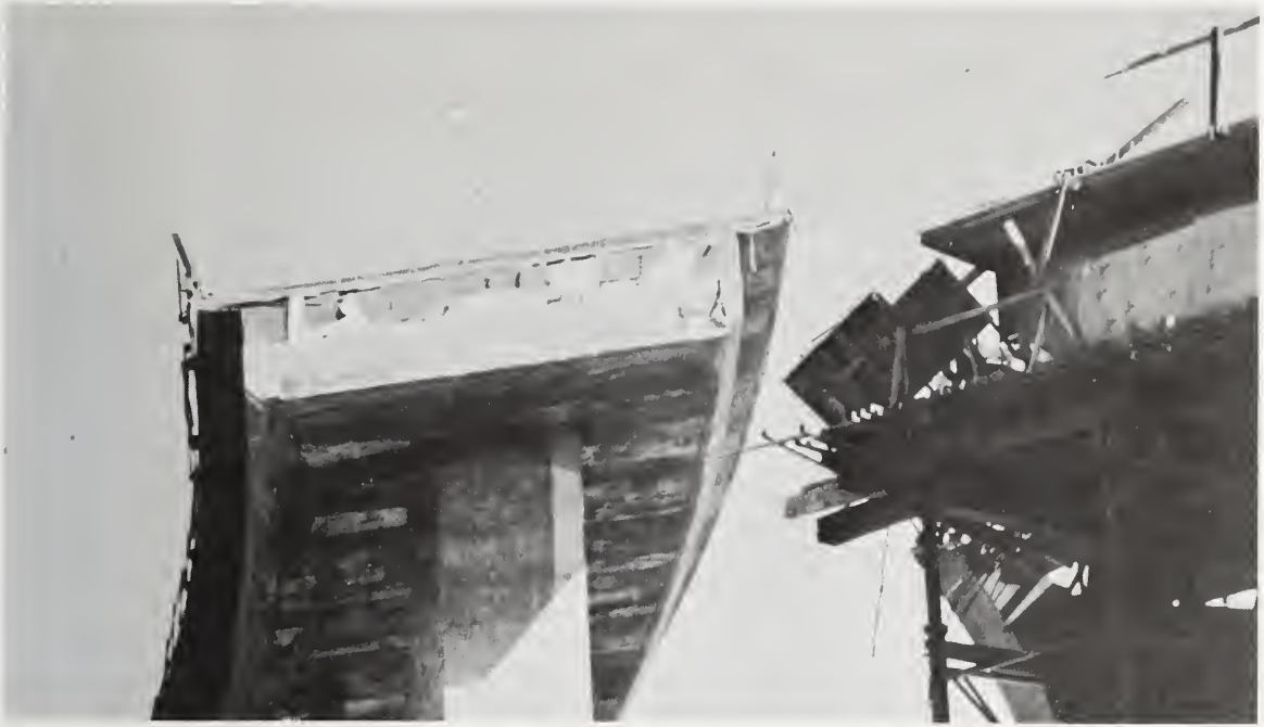
Figure 7.6 Post-failure view of Pier 3 and hinge seat with shear key.
