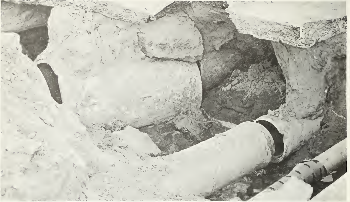
Figure 8.21 Close-up view of ruptured sewer, water, and gas lines.
