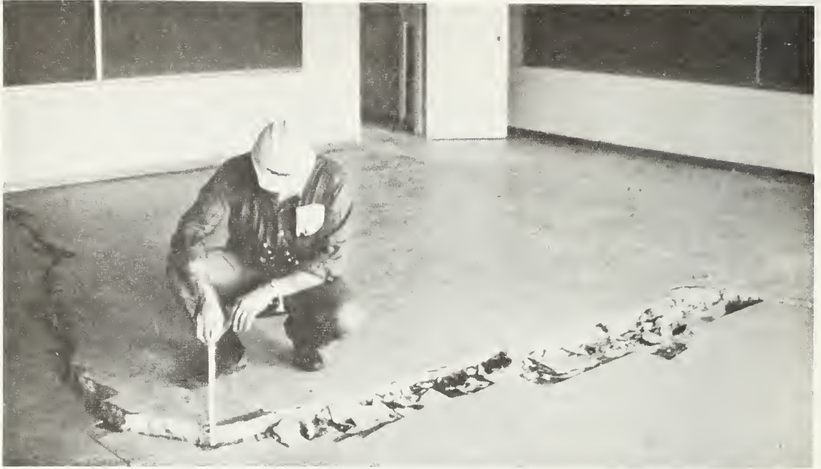
Figure 6.8 Cracked slab with a vertical displacement of approximately 3 1/2 inches, Harding Street School.
