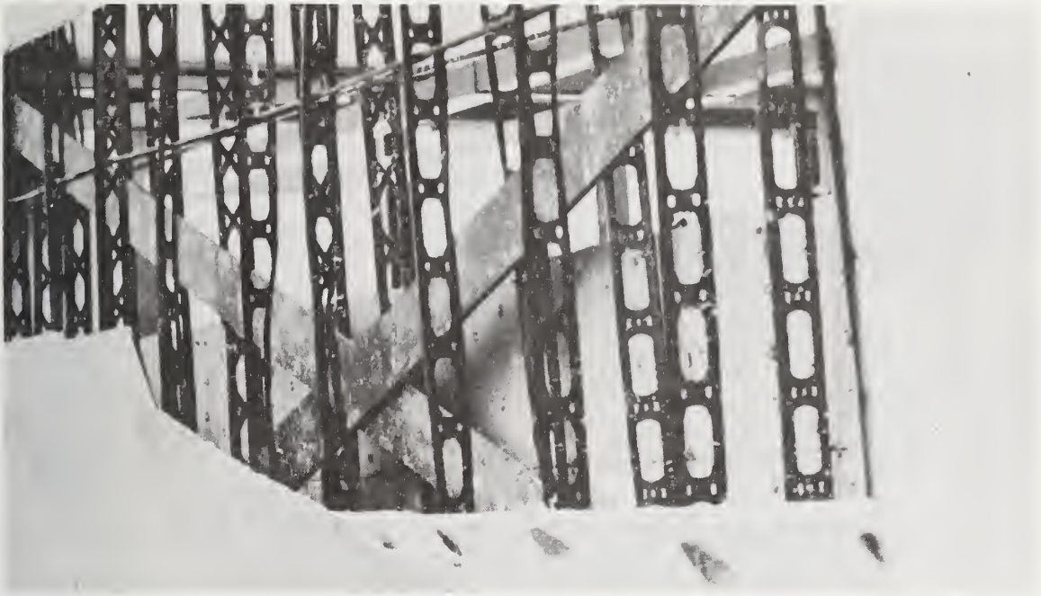
Figure 6.34 Flat steel bar braces concealed in transverse partitions, Clark Junior High School. Damage to partition caused by buckling of brace and striking the studs.
