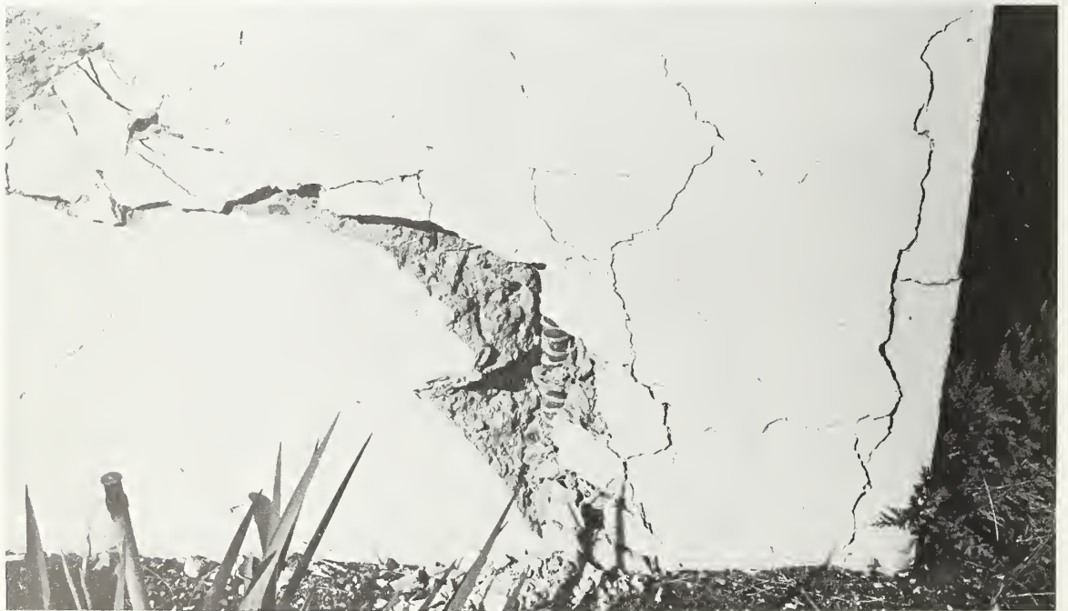
Figure 5.105 Cracking at the base of the southeast corner shear wall. Note the exposed reinforcing bar.
