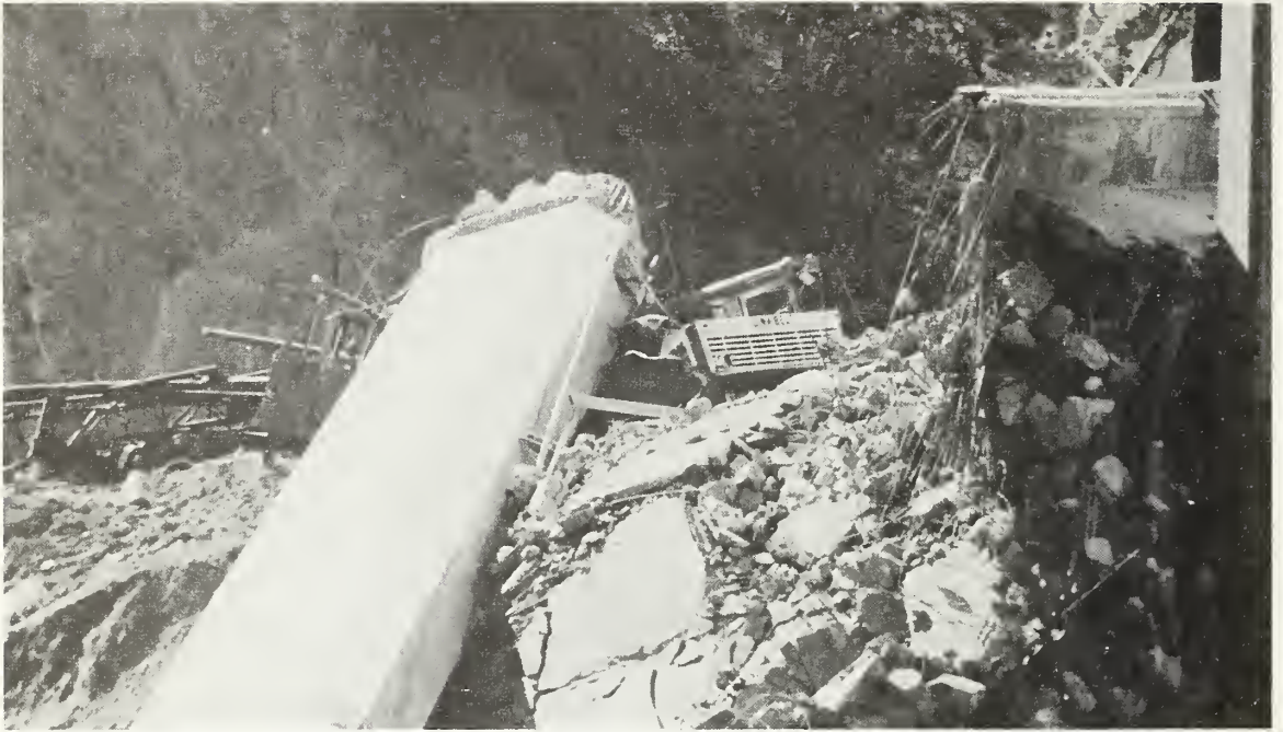
Figure 7.8 The top of Pier 5 and girder debris from the South Connector Overcrossing.
