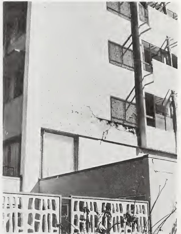
Figure 5.63 Failure at third-story construction joint at the west end of the tower.
