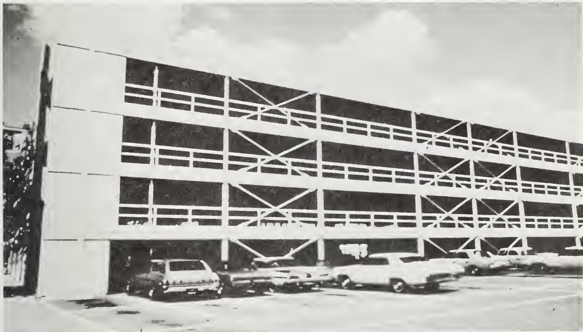
Figure 5.184 General view of parking structure, located at 2215 Purdue Avenue in west Los Angeles.
