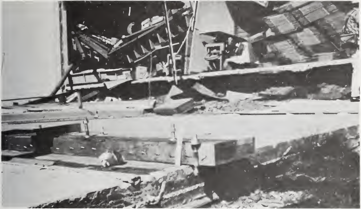
Figure 5.182 The roof collapsed when the exterior wall pulled away.
