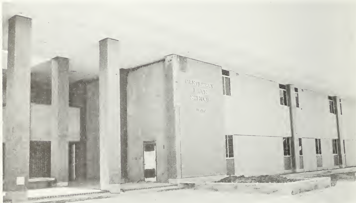
Figure 6.27 Ceramic tile fell from wall, Castlebay Lane School.
