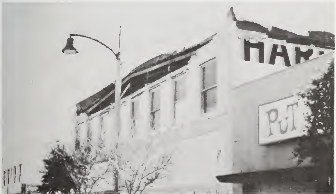
Figure 5.141 Damaged parapet and wall.
