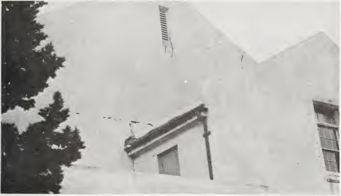
Figure 6.6 Brick wall was displaced at the gable end, Morningside School Building #2.
