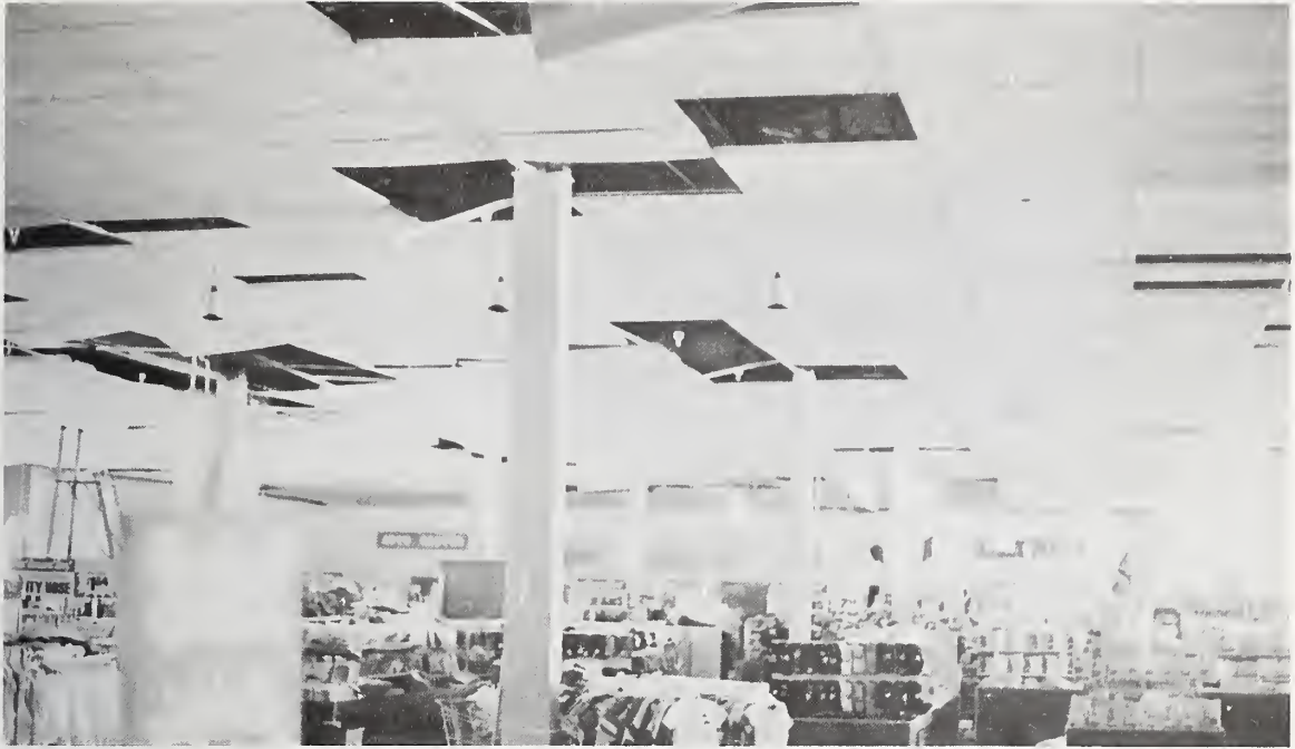
Figure 5.130 Interior view of Grants Department Store showing missing portions of suspended ceiling. Most of the merchandise which had been thrown to the floor had been picked up when this photograph was taken.
