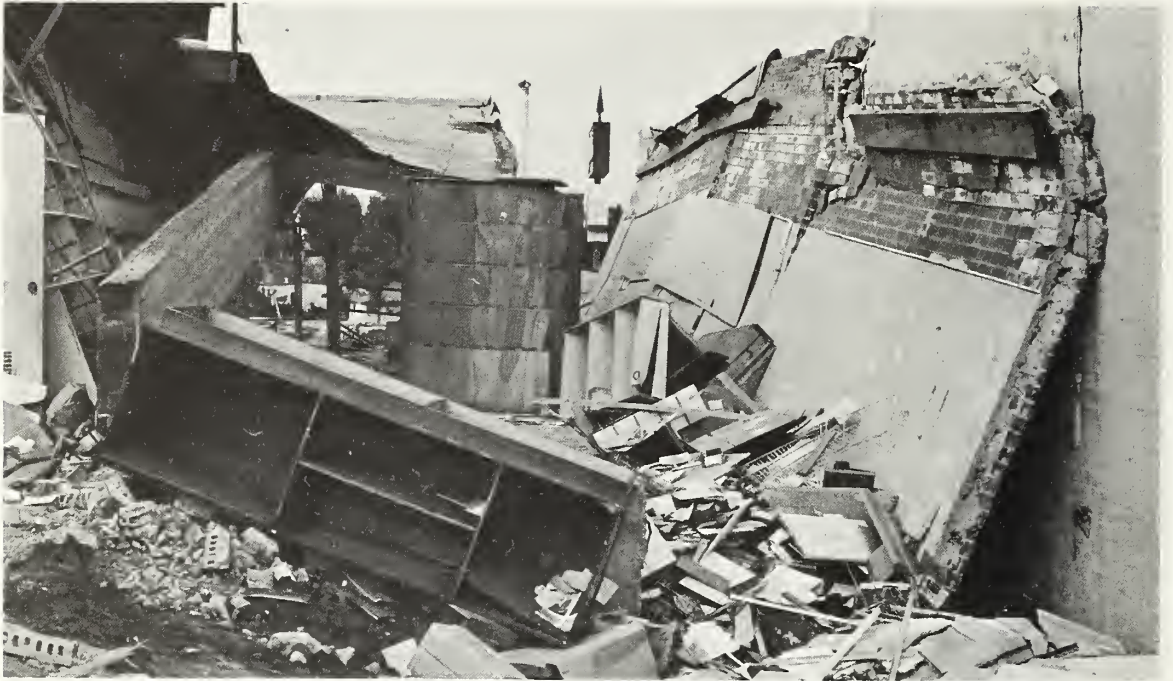
Figure 5.134 Collapsed side wall shown in figure 5.133 as viewed from the rear of the store.
