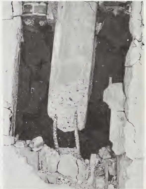
Figure 5.50 Close-up view of one of many damaged columns in Building 6. Note a lack of ties around the exposed square reinforcing bars.
