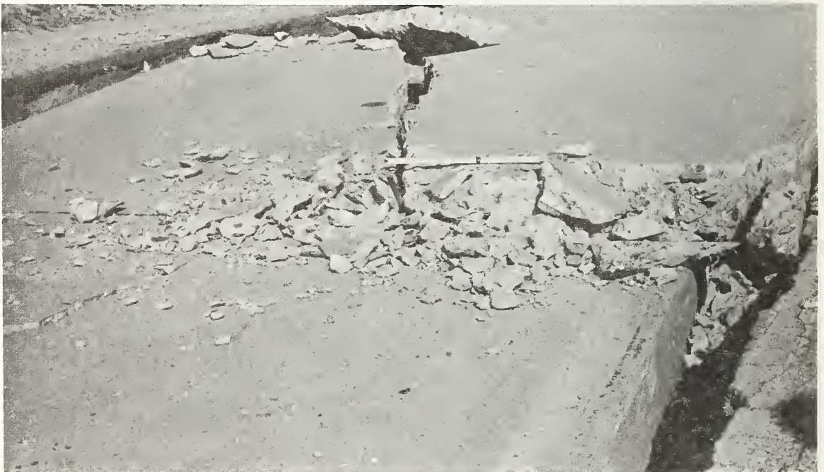
Figure 7.36 Concrete road slabs were crushed by the ground motion in this location.
