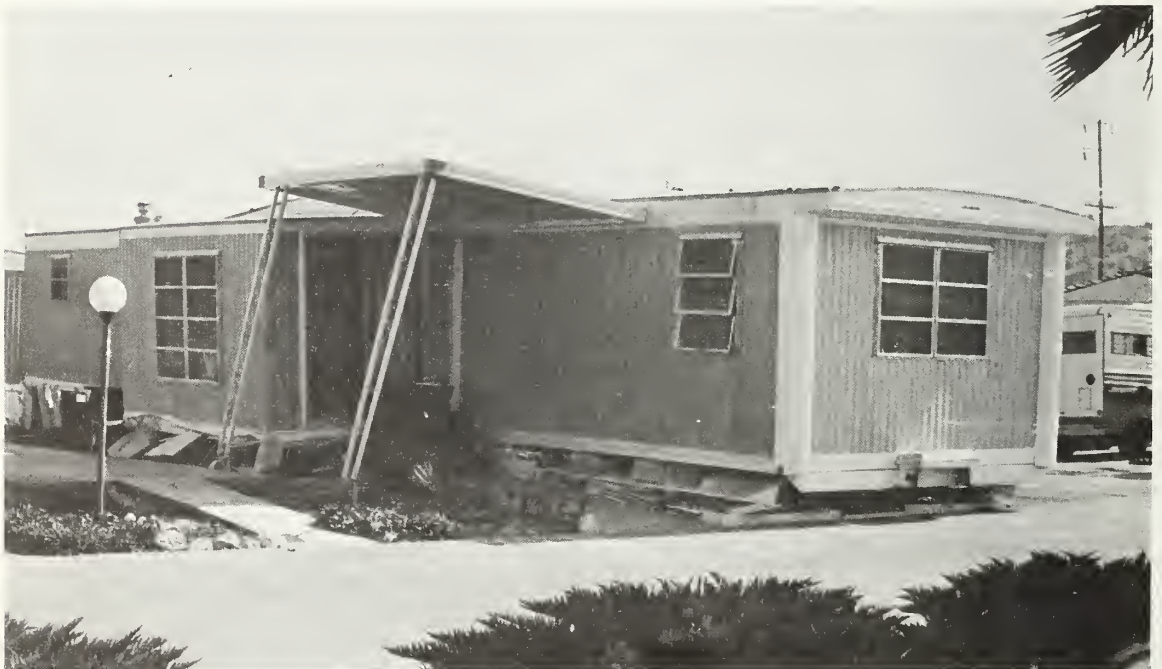
Figure 5.173 Mobile home (Soledad Canyon Road, Newhall) which was damaged when it fell off its small concrete and metal base supports.
