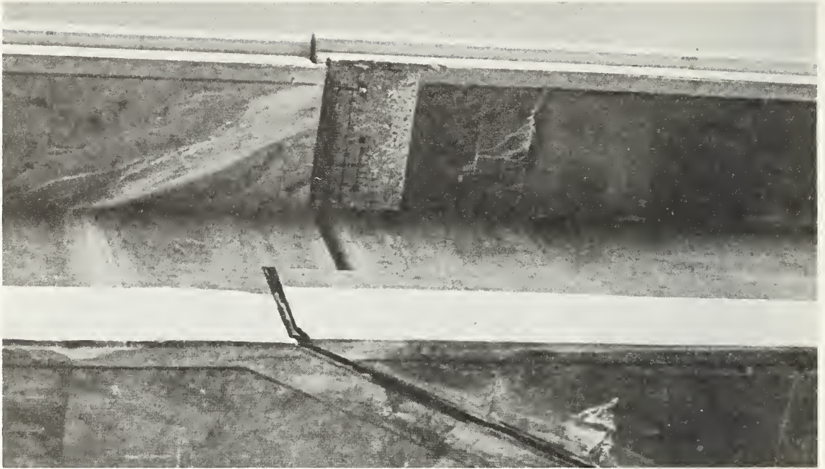
Figure 7.32 Typical movement and spalling at a joint in an elevated box girder bridge, caused by battering at the joints.
