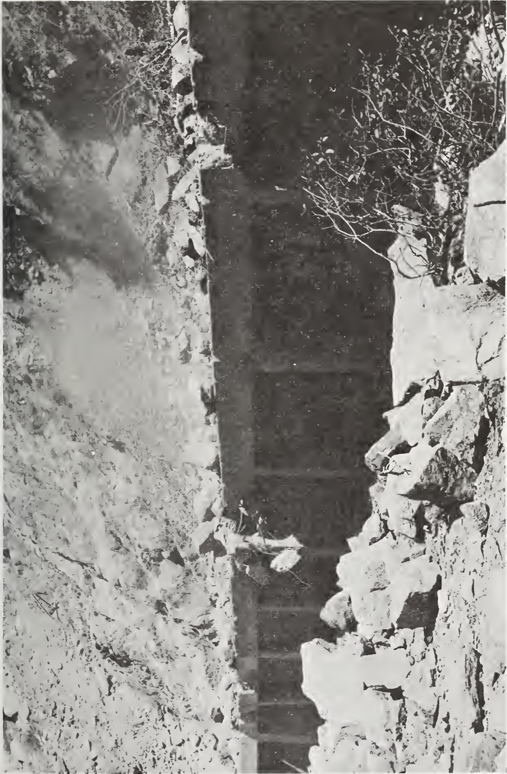
Figure 8.29 Slides on access road along covered walkway, Pacoima Dam.
