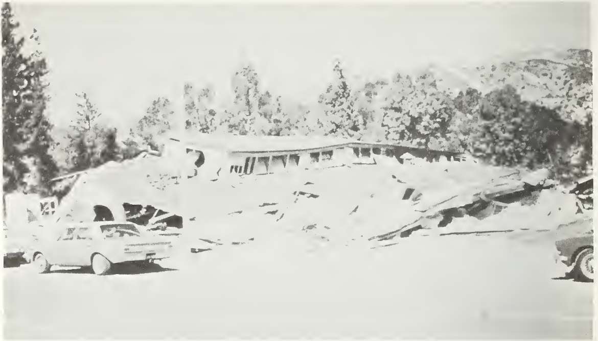
Figure 5.40a Totally collapsed old brick building at the old section of the Olive View Medical Center. The building was not designed to resist earthquake forces.
