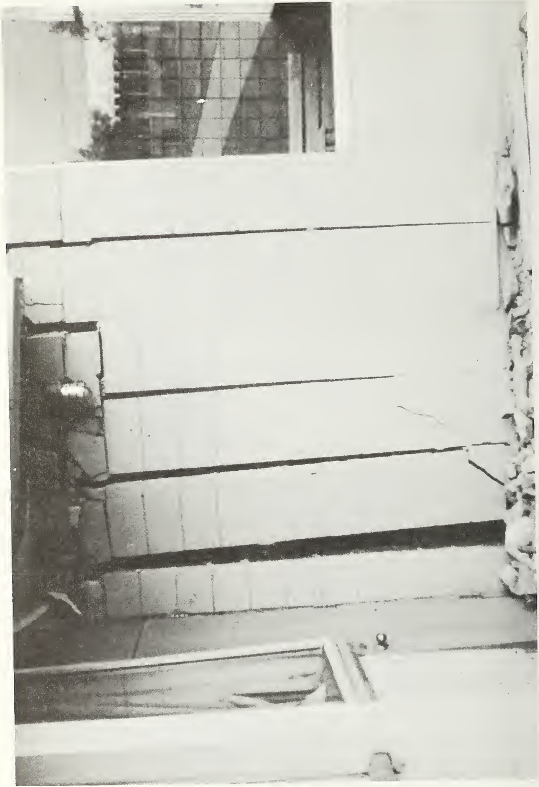
Figure 6.51 Damage to concrete block wall, Los Angeles County Juvenile Facility. Note absence of horizontal reinforcement. Only reinforced vertical cells are filled with grout.
