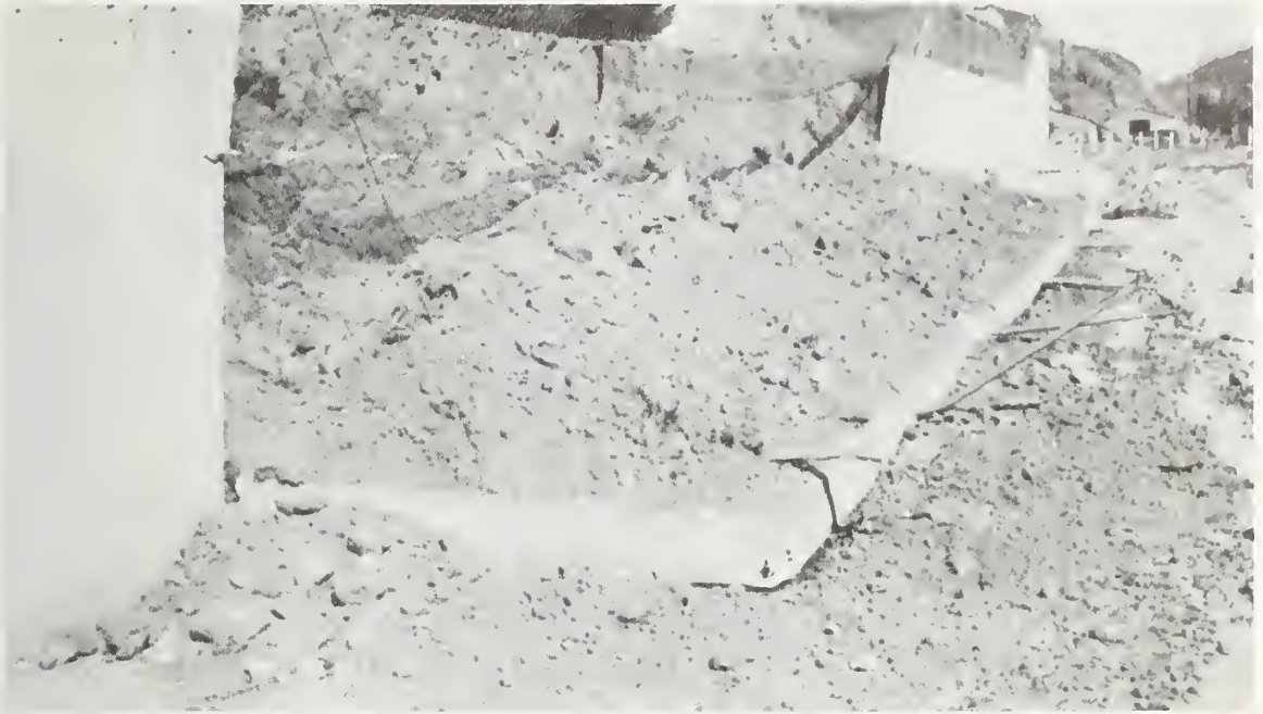
Figure 8.34 Lopez Canyon Channel. A 50-foot section of the wall has failed on the right bank. The 50-foot section adjacent upstream also shows severe structural damage.
