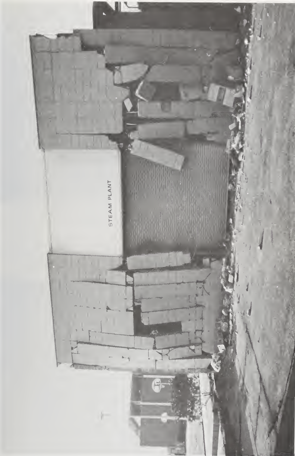
Figure 6.52 Damage to concrete block wall, Los Angeles County Juvenile Facility. Note absence of horizontal reinforcement. Only reinforced vertical cells are filled with grout.
