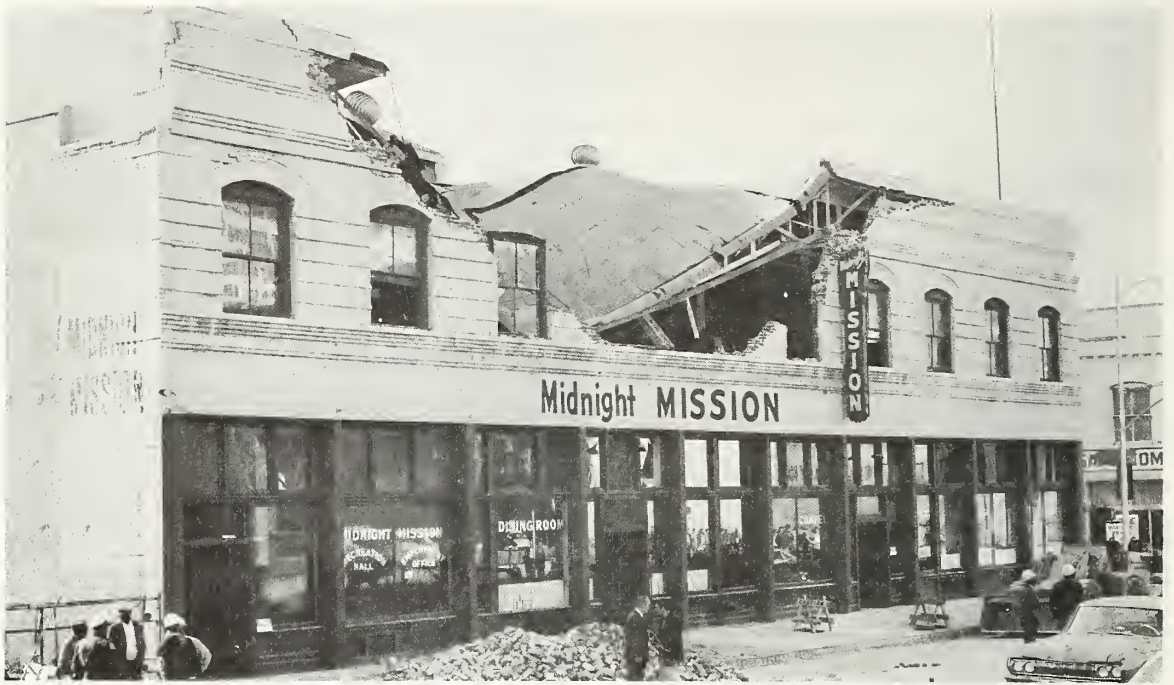
Figure 5.148 Midnight Mission, 396 South Los Angeles Street, in downtown Los Angeles. This building, erected in 1896, provided shelter for about 200 men. One man was killed when he ran out of the front door and was struck by falling masonry. (Los Angeles Times Photo).
