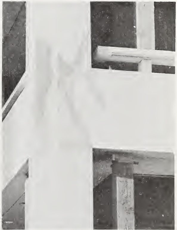
Figure 5.115 Cracked beam-column connections at the first floor were repaired with epoxy.
