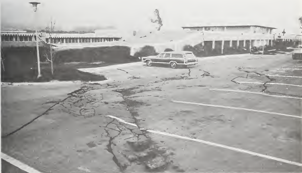
Figure 6.37 A portion of the Administration Wing collapsed at the Los Angeles County Juvenile Facility. Note the distortion of the ground surface.
