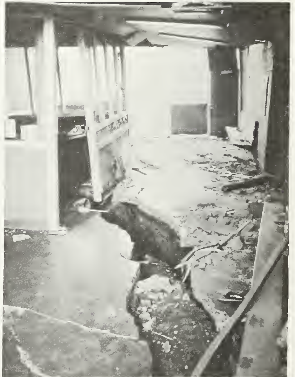
Figure 6.39 Large displacement in floor of girls' living unit, Los Angeles County Juvenile Facility. Structure did not collapse.
