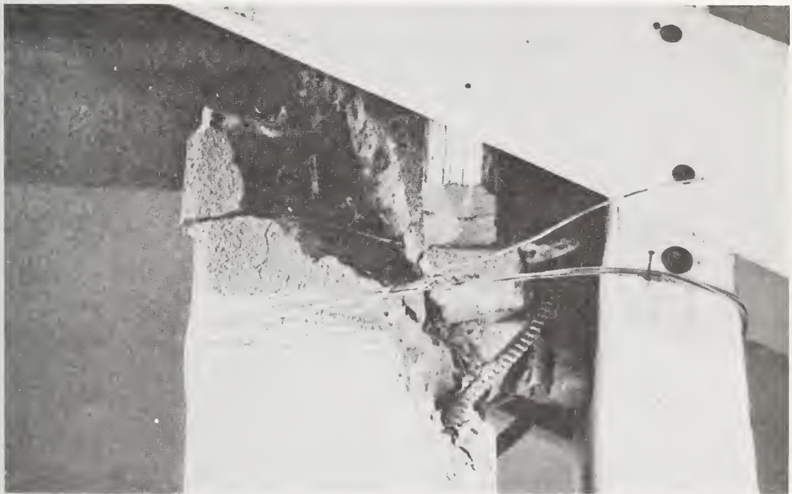
Figure 6.23 Close up of fractured concrete second-story covered arcade column, Patrick Henry Jr. High School.
