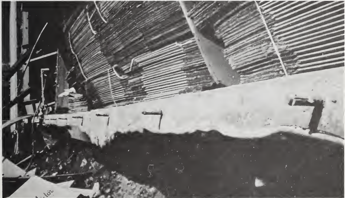
Figure 5.183 Typical failure of drilled-in anchors.
