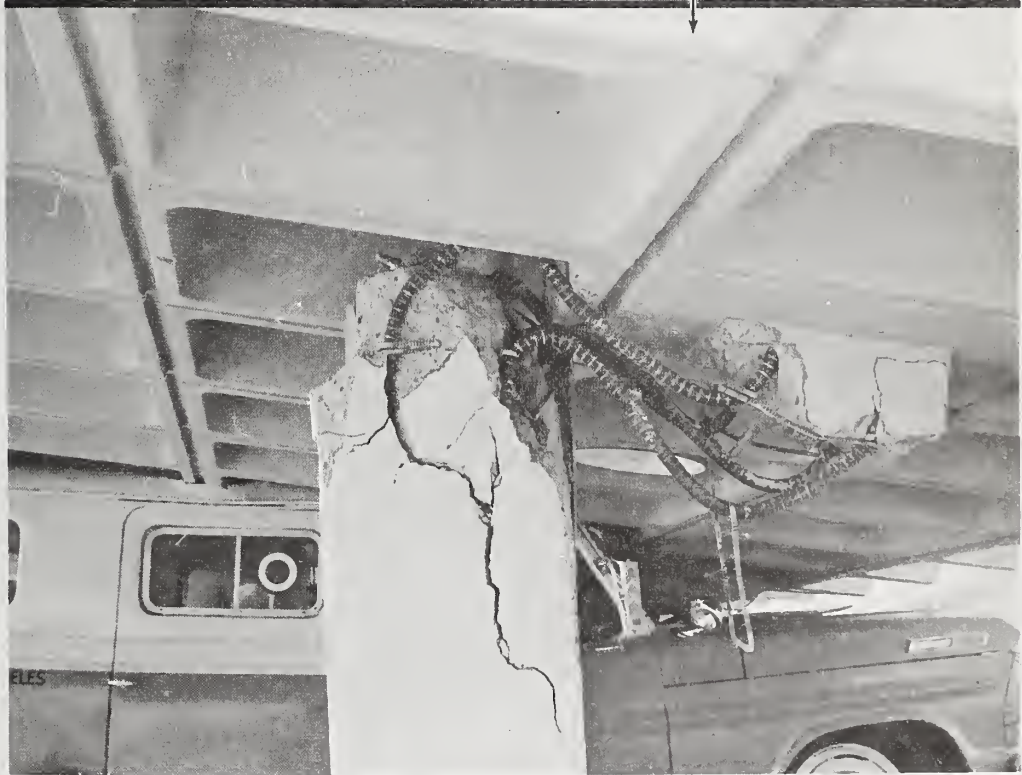
Figure 5.39 Damaged reinforced concrete ambulance port south of Wing D.
