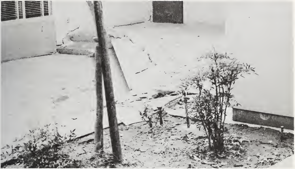
Figure 6.10 Buckled slab on grade at Van Gogh Street School.
