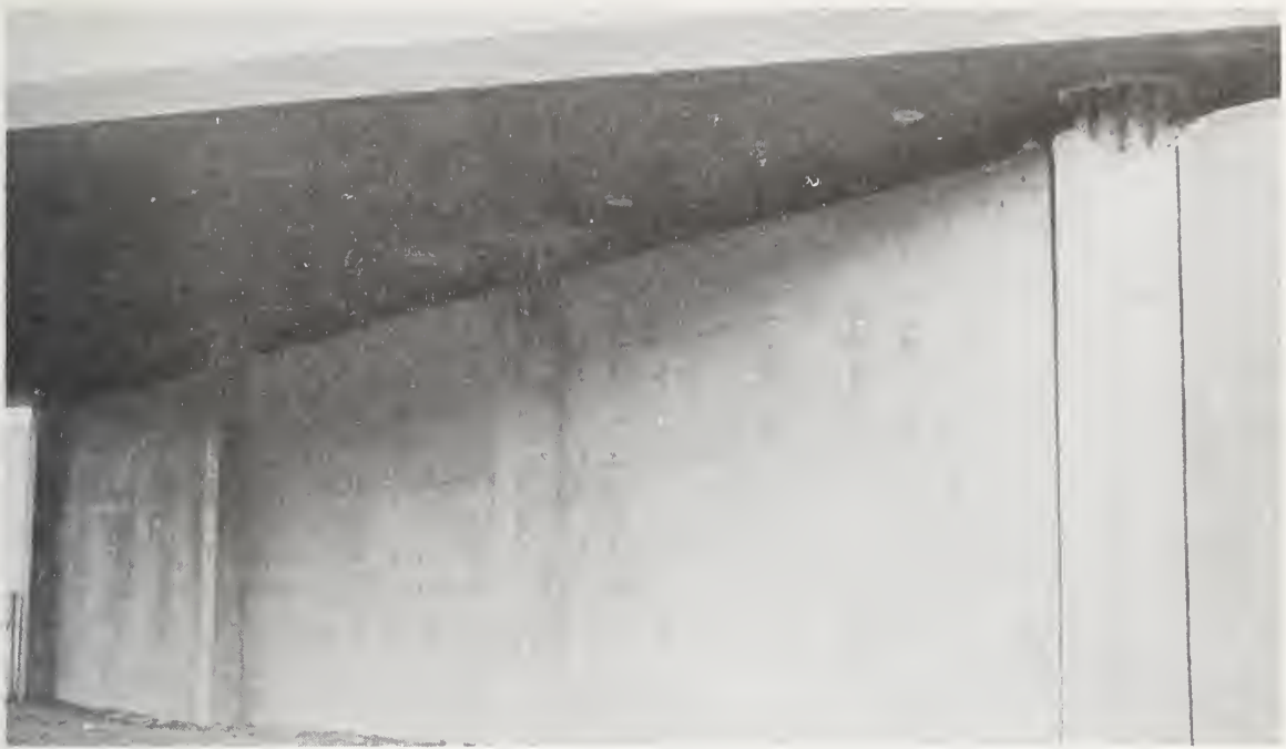
Figure 7.28 Damaged columns in bent 4 with 10-in closure wall which was separated from the columns by 1/2-in filled expansion joints.
