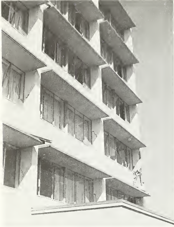
Figure 5.58 View of the failed column at the southeast corner of the fourth story.
