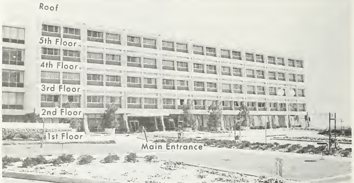
Figure 5.18 West face of Wing A. Note the extensive damage at the first floor and the lateral displacement of the building to the north. Most glass was intact in windows above the third floor.
