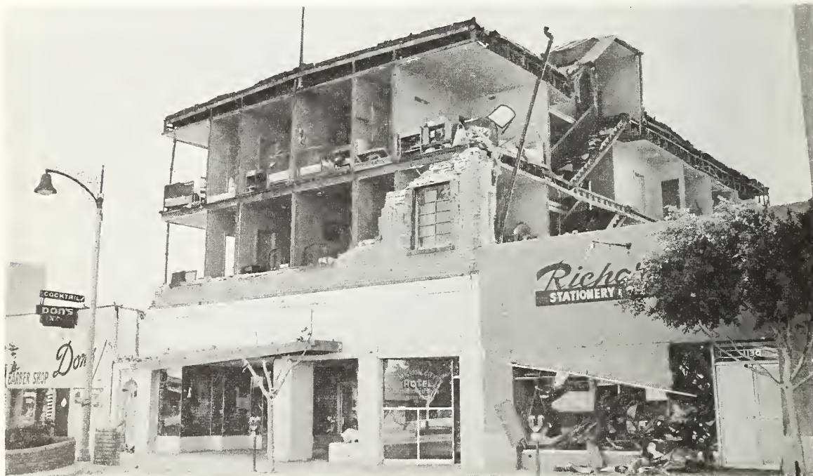
Figure 5.139 Total collapse of brick masonry wall surrounding three-story wood frame building (Mission City Hotel).
