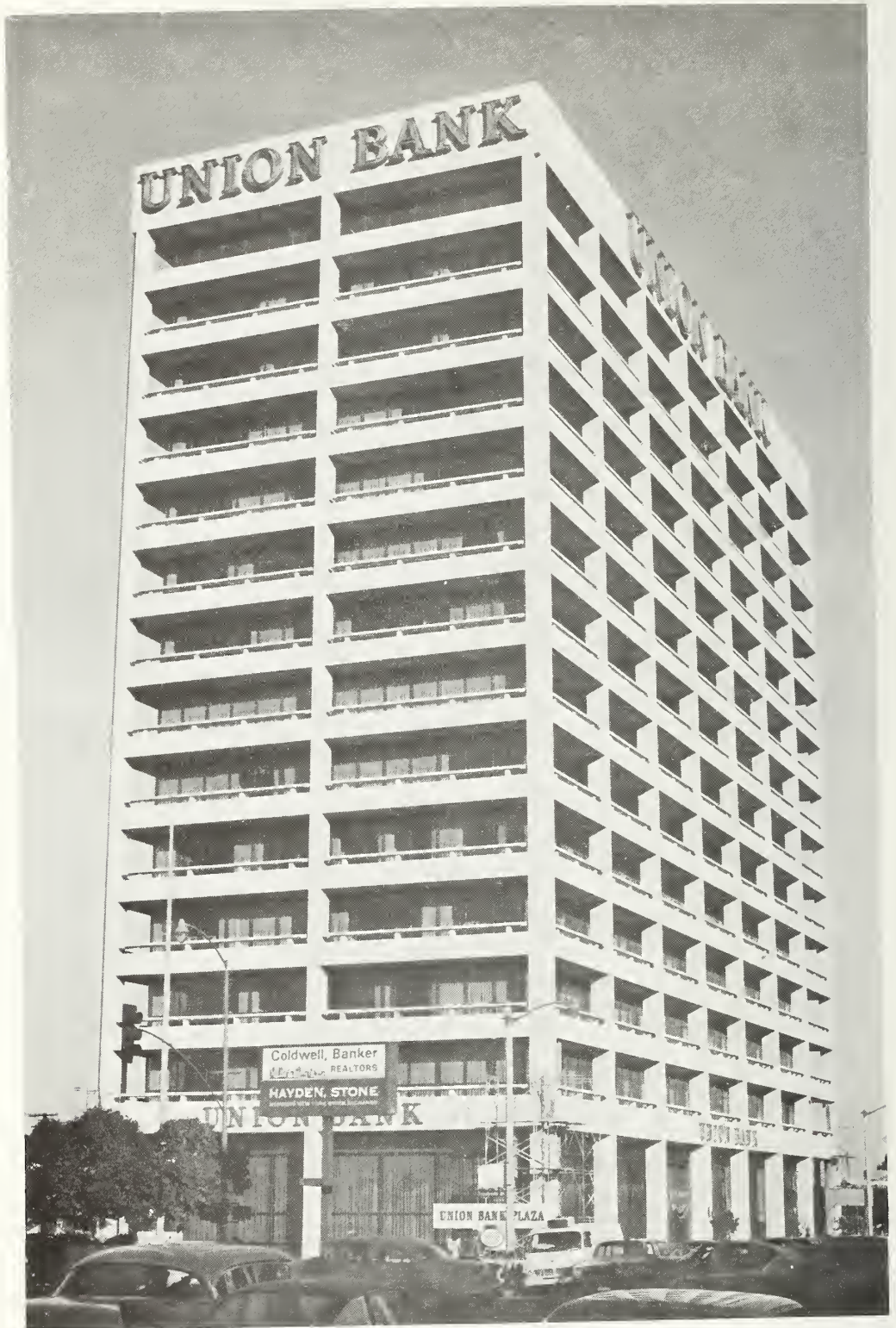
Figure 5.113 The south and west elevations of the thirteen-story Union Bank building. All four exterior corner columns in this reinforced concrete structure were cracked at the second floor level.
