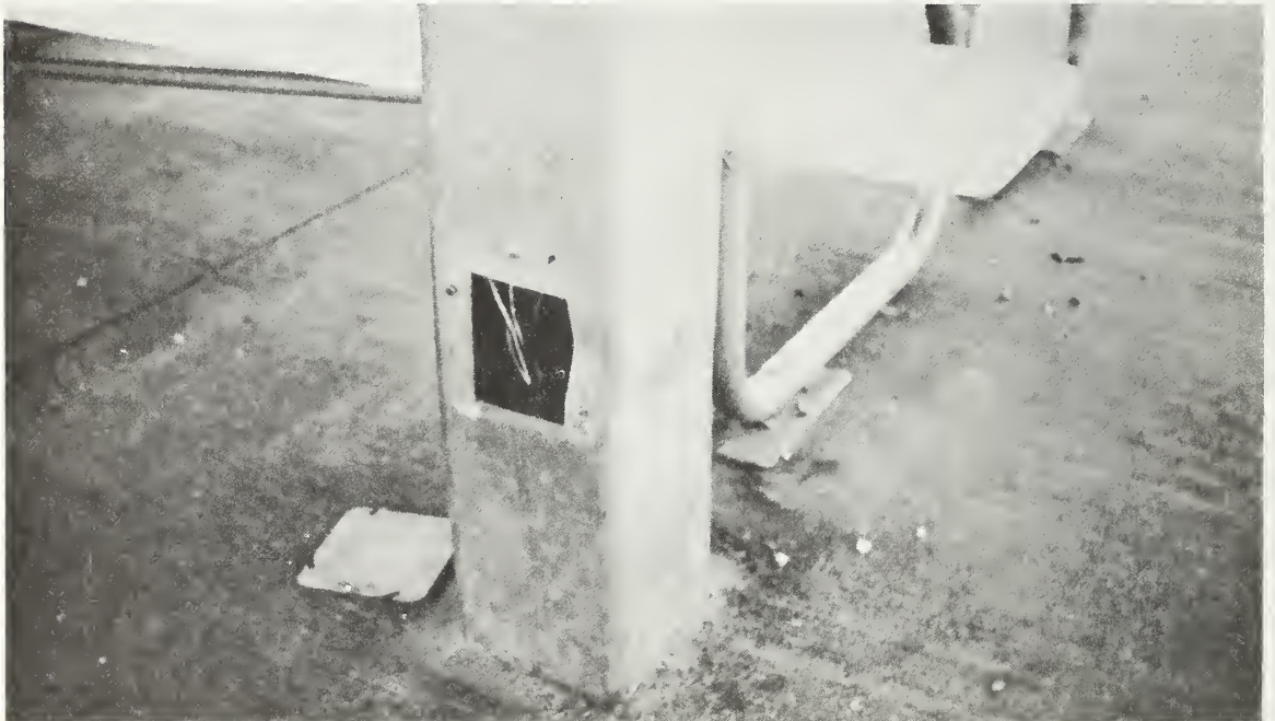
Figure 6.13 Lunch shelter columns were permanently bent at opening for electrical outlet box, Van Gogh Street School.
