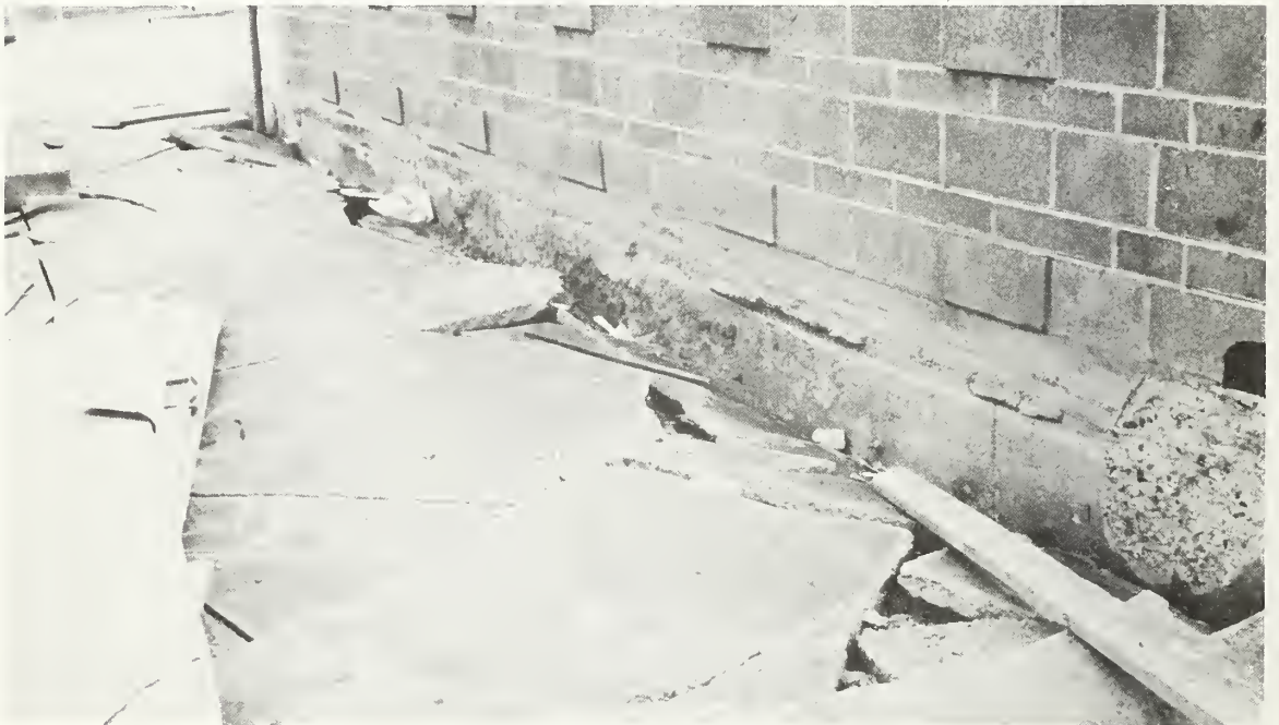
Figure 6.58 Approximately 6 inches of vertical displacement between masonry classroom building and the portable classroom building, Camp Karl Holton.
