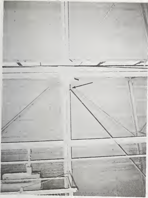
Figure 6.20 Horizontal bracing rod pulled out of clevis, San Fernando High School.
