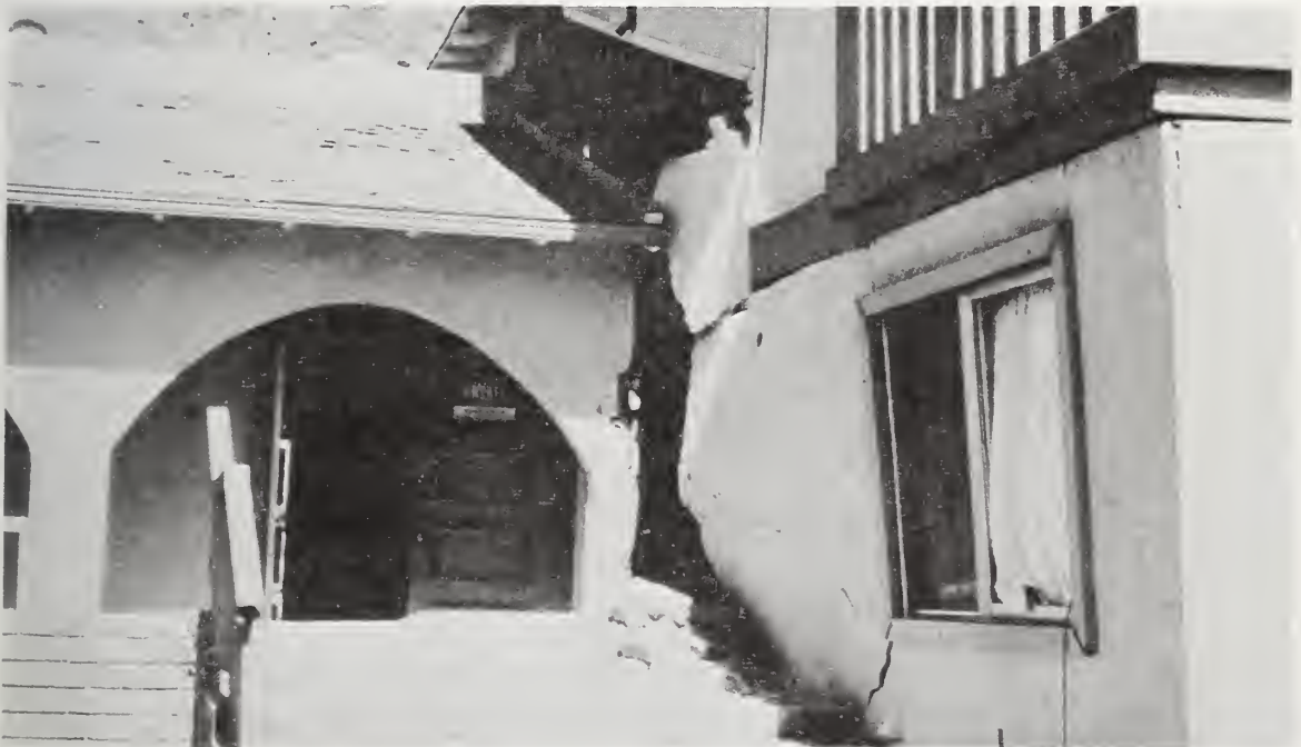
Figure 5.161 Closeup of damaged split-level residence shown in figure 5.160.
