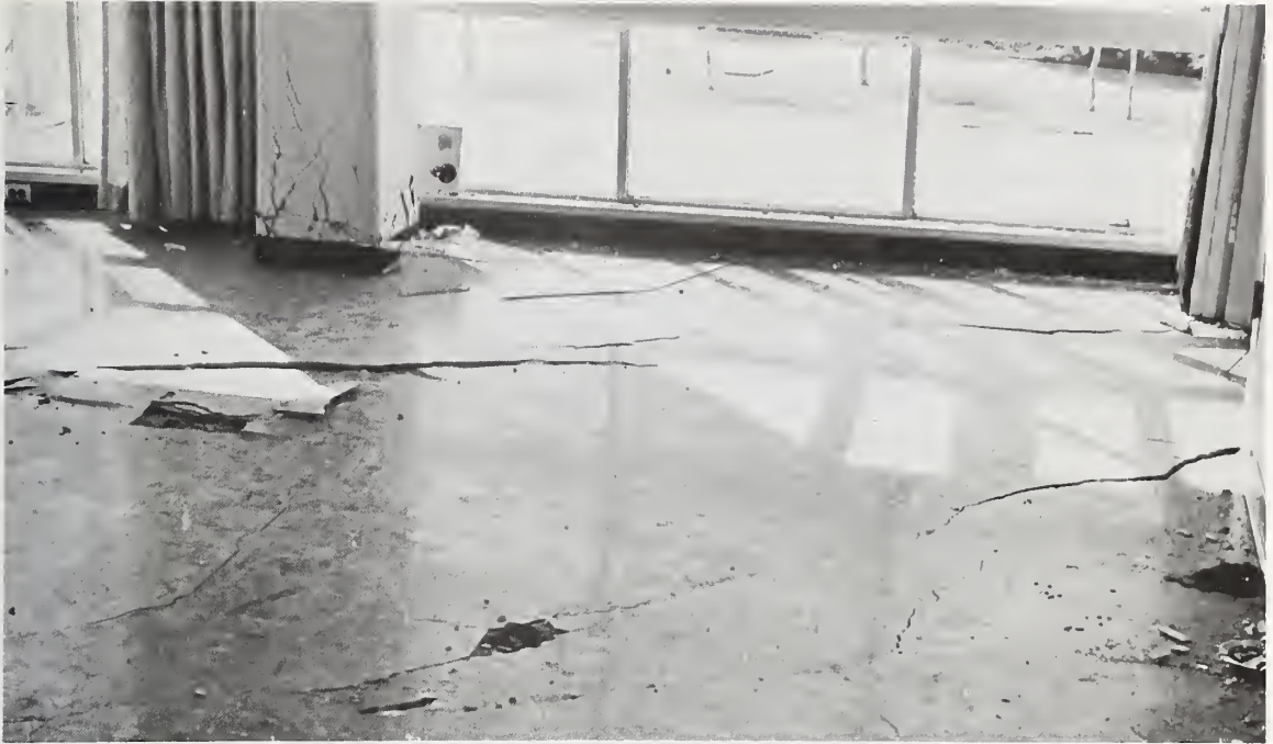
Figure 5.65 Floor damage at the west end of the third floor.
