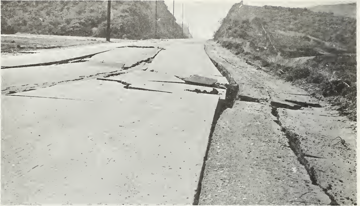
Figure 7.35 Road cave-in and ground cracks along Blucher Avenue along the eastern edge of the lower Van Norman Reservoir.
