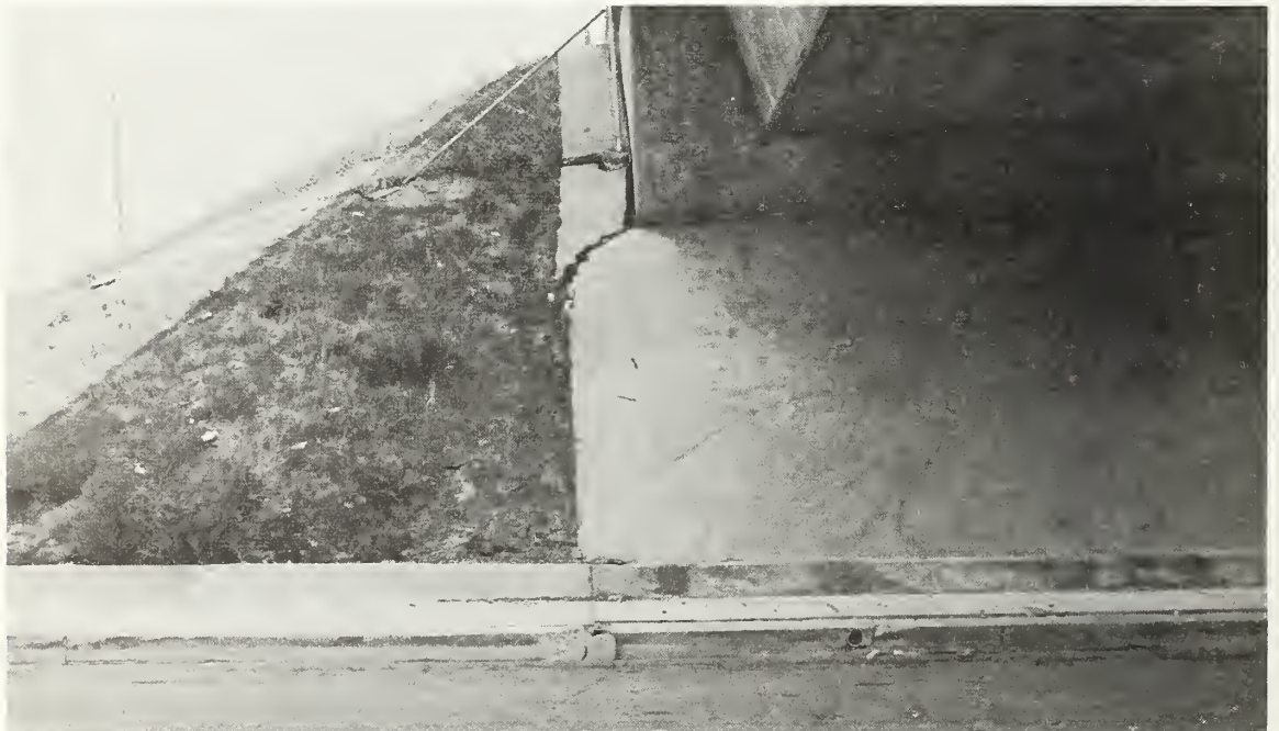
Figure 7.33 Typical damage to wing walls and sloped paving on a single span prestressed concrete box girder bridge.
