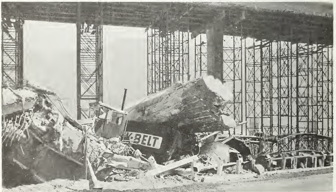
Figure 7.9 The top of Pier 5, which was embedded in the girder diaphragm, resting on the construction crane after collapse.
