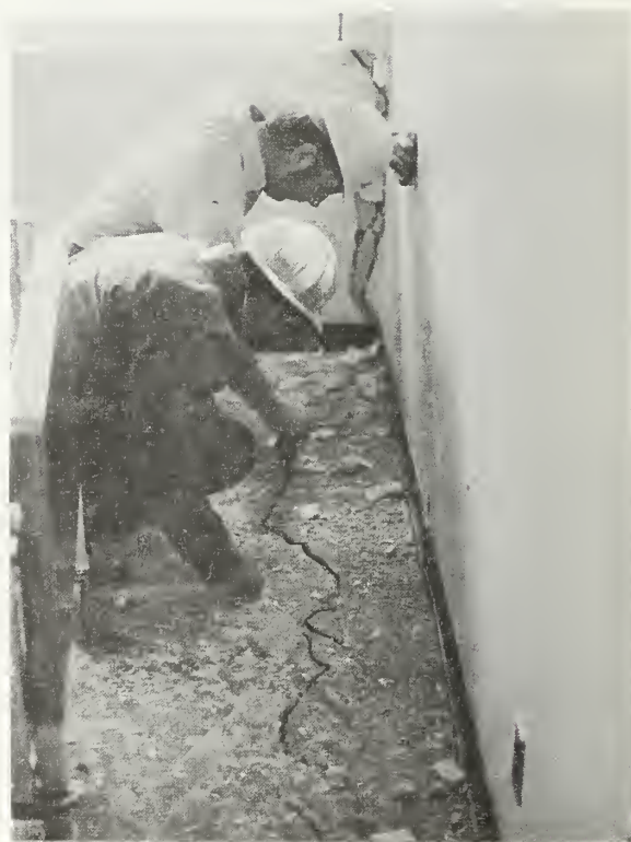
Figure 5.68 Damaged southwest corner room on the third floor. Note floor and spandrel cracking.
