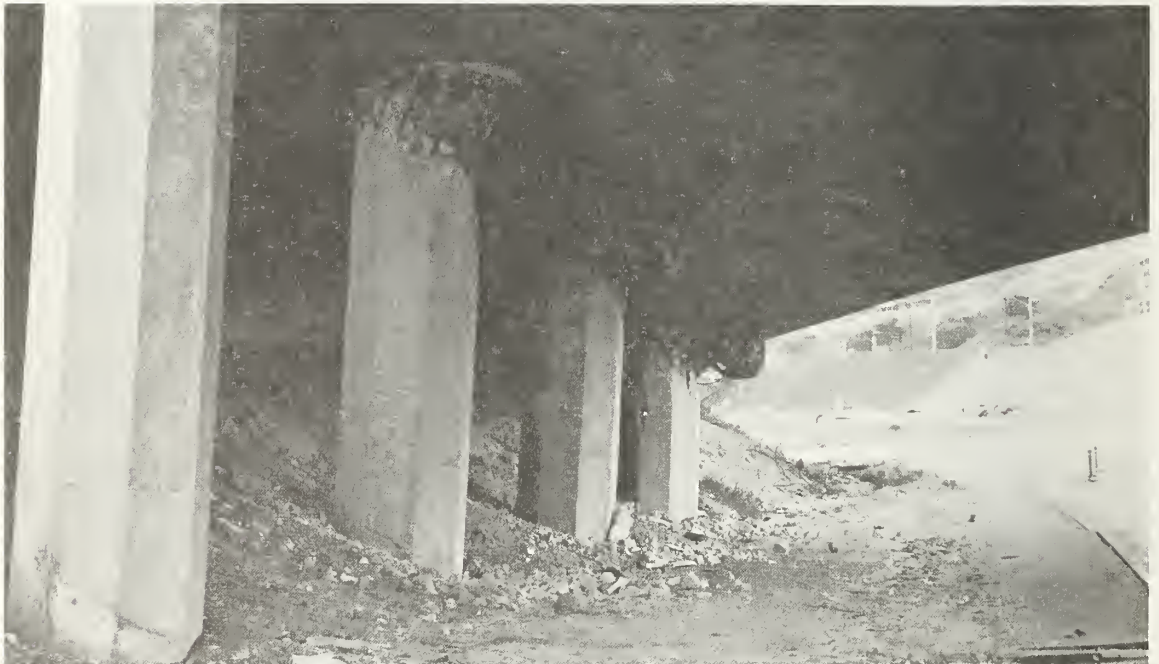
Figure 7.23 Spiral column failures in bent 2 at the west end of the Northwest Connector Overcrossing.
