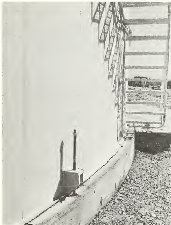
Figure 8.6 Vertical Movement of tank pulled one-inch diameter anchor bolt out of concrete base.
