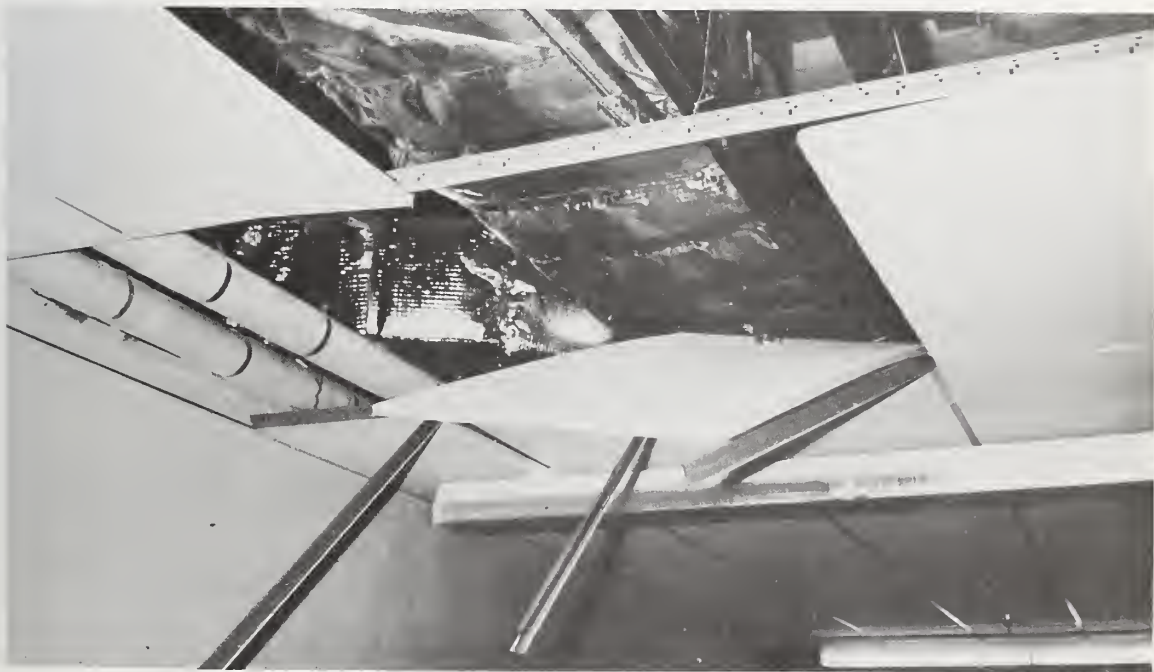
Figure 6.29 "T" bar ceilings were damaged, Castlebay Lane School.
