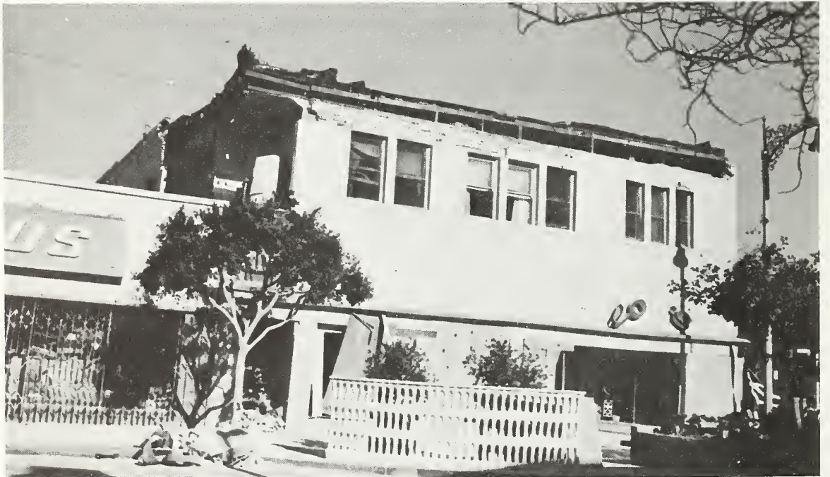
Figure 5.143 Collapsed wall and parapet.
