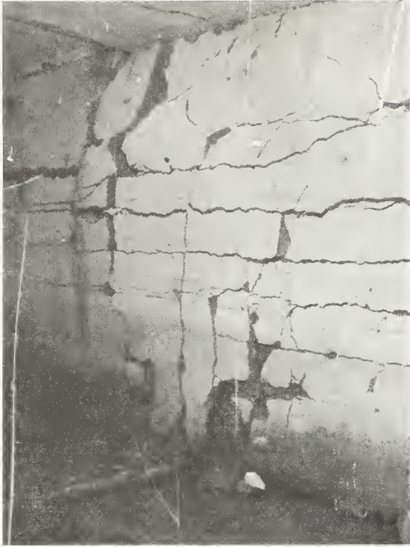
Figure 8.32 Left wall buckled inward at station 45+10. Wilson Canyon Channel.
