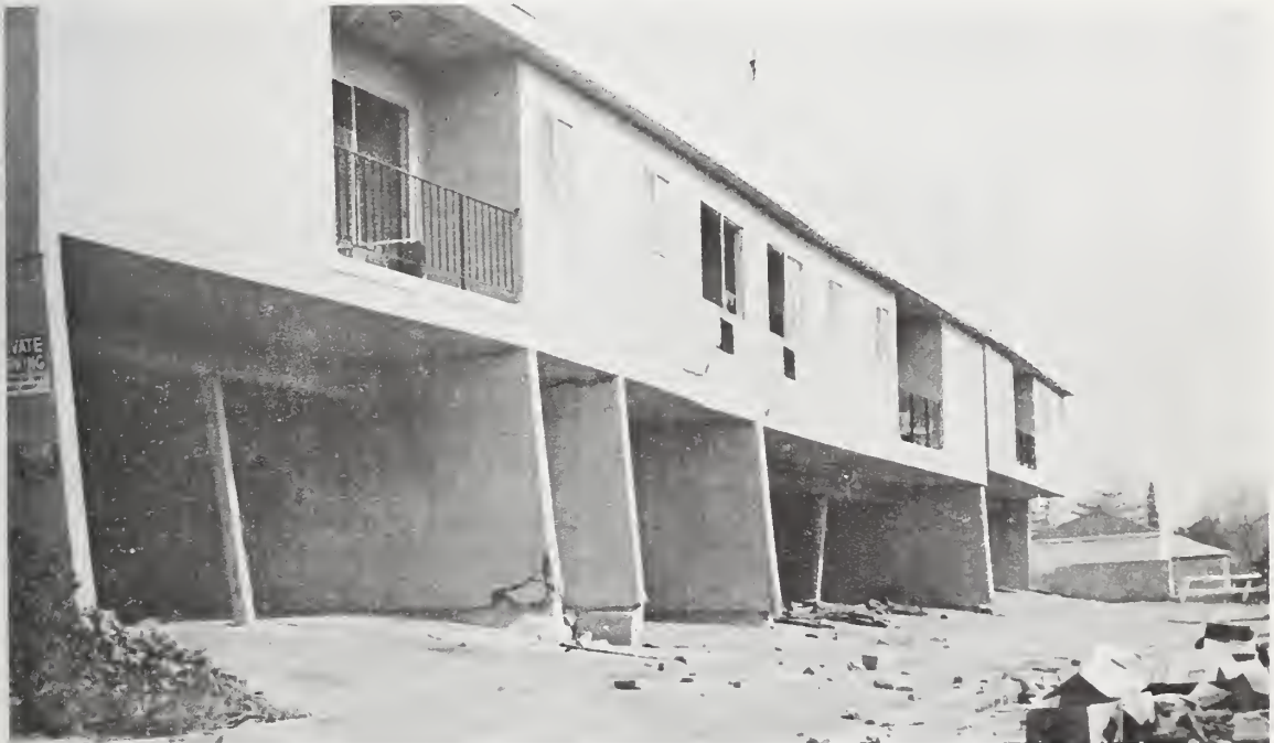
Figure 5.171 Rear view of damaged two-story Mardette apartment building.
