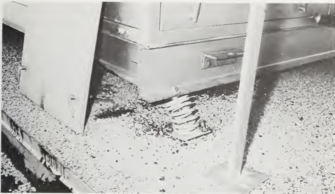
Figure 6.28 Mechanical equipment moved off the isolation mounts, Castlebay Lane School.
