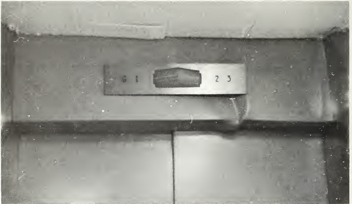
Figure 5.84 Buckled steel elevator door frame in the Pacoima Hospital.
