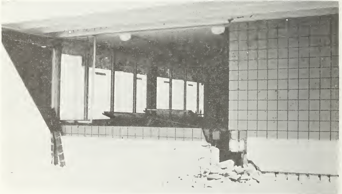
Figure 6.43 Damage to west wall of boys' school, Los Angeles County Juvenile Facility. Window fell inward.
