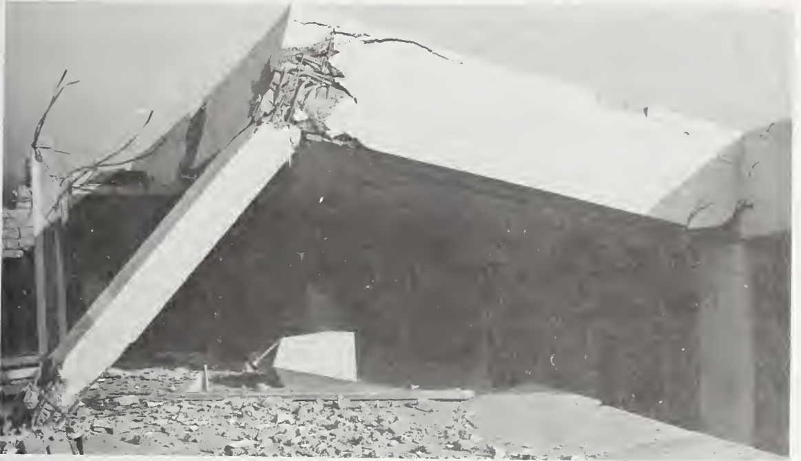
Figure 5.13 Damage to the canopy at the front (north) entrance to the Psychiatric Unit.
