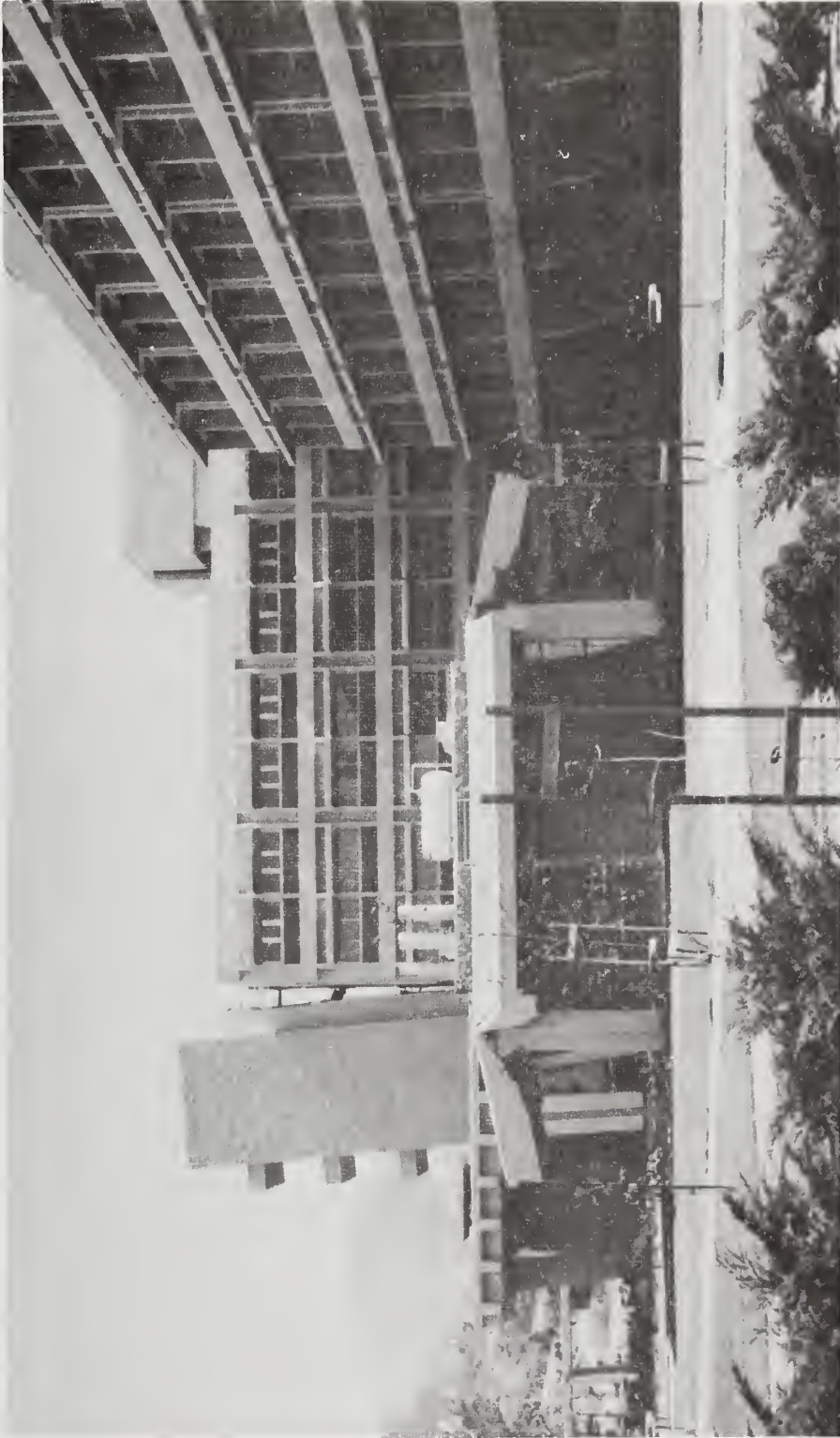
Figure 5.37 The damage to the overhanging canopy of the exhaust pavilion possibly indicates large vertical accelerations.
