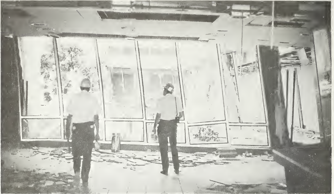
Figure 5.28 Damaged main lobby in Wing A. Note the window mullion distortion. The planted area seen through the window is a court enclosed by the four wings.
