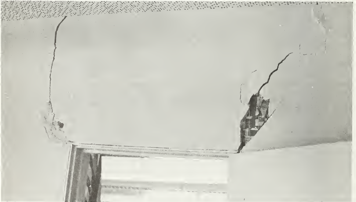
Figure 6.9 Plaster cracks over door at Harding Street School. Racking of wall caused doors to bind in the steel frames.
