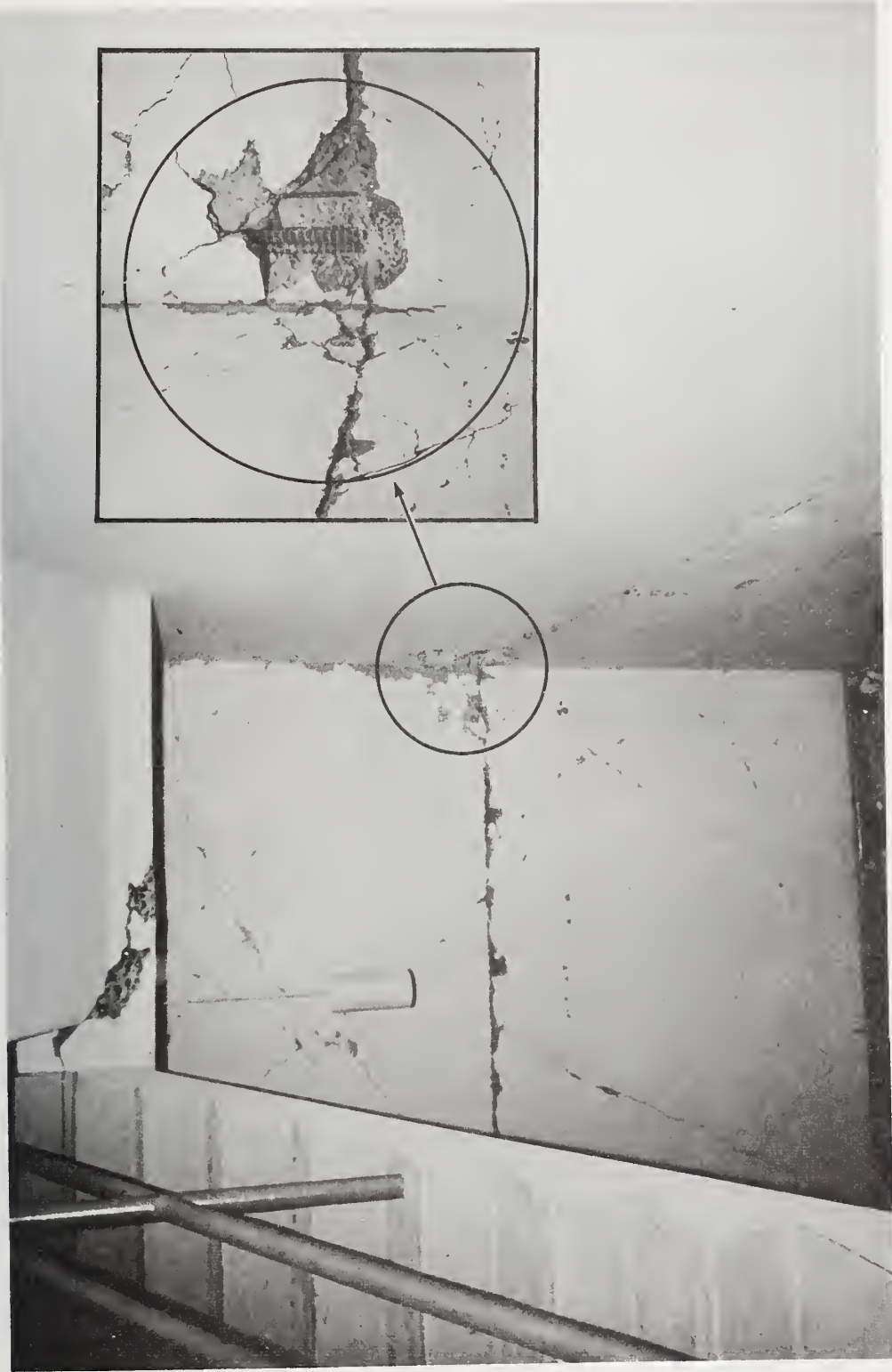
Figure 5.69 Diagonal and horizontal cracking in stairwell near the west end of the building. The horizontal crack is at the third floor.
