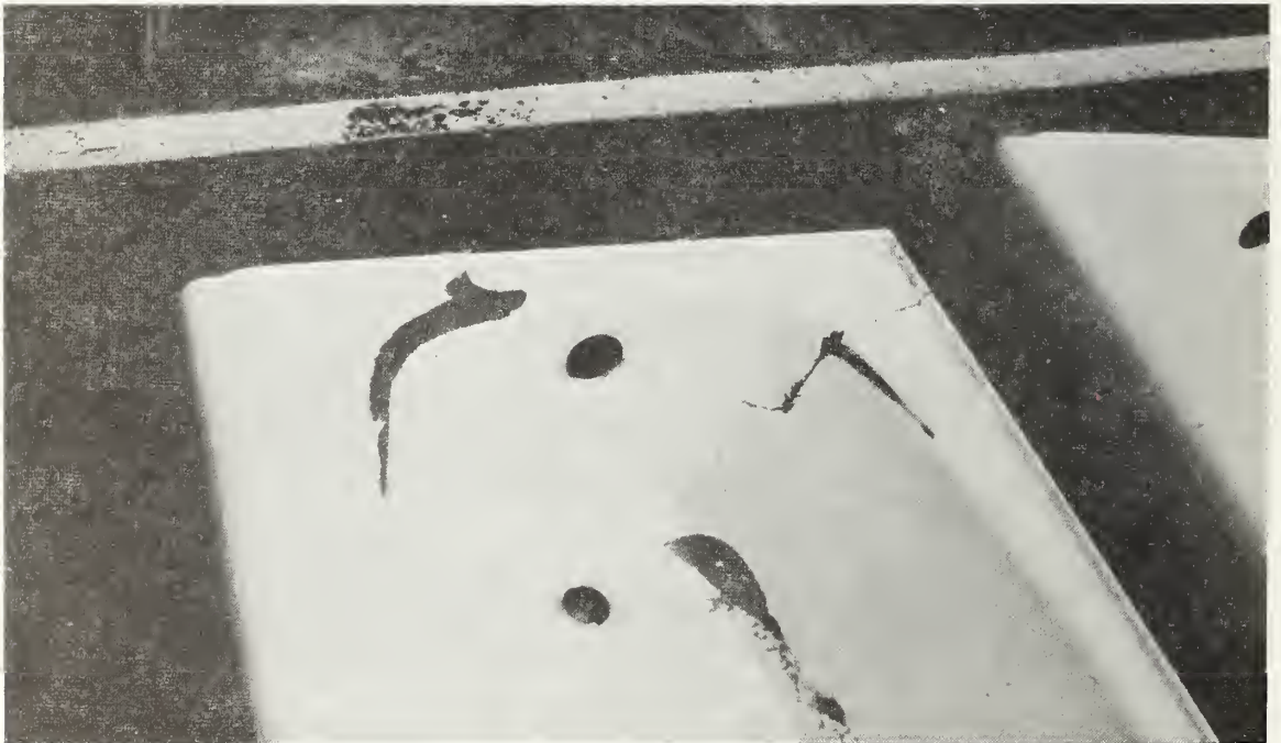
Figure 5.110 Cracked and chipped bathtub.
