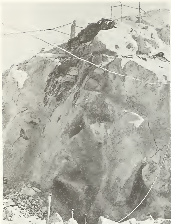
Figure 8.27 Damage to gunite left abutment, Pacoima Dam.
