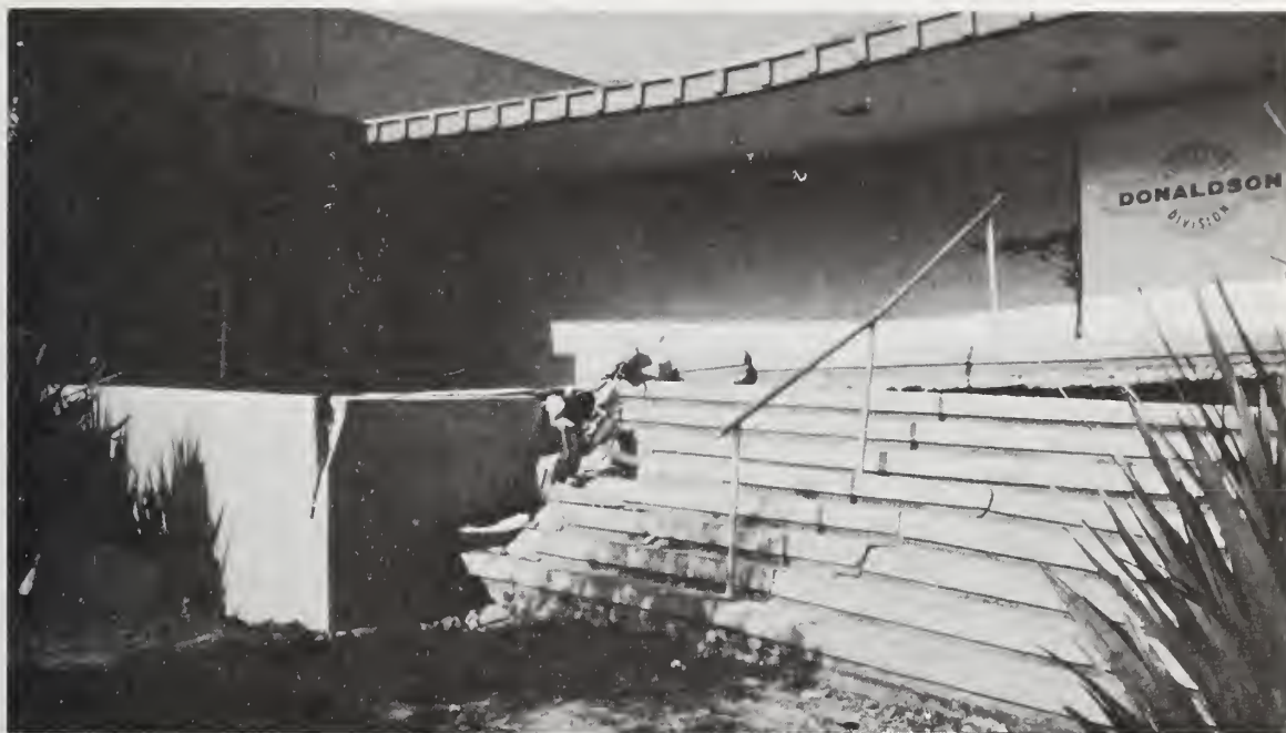
Figure 5.180 Ground faulting caused separation of the concrete slab and steps.
