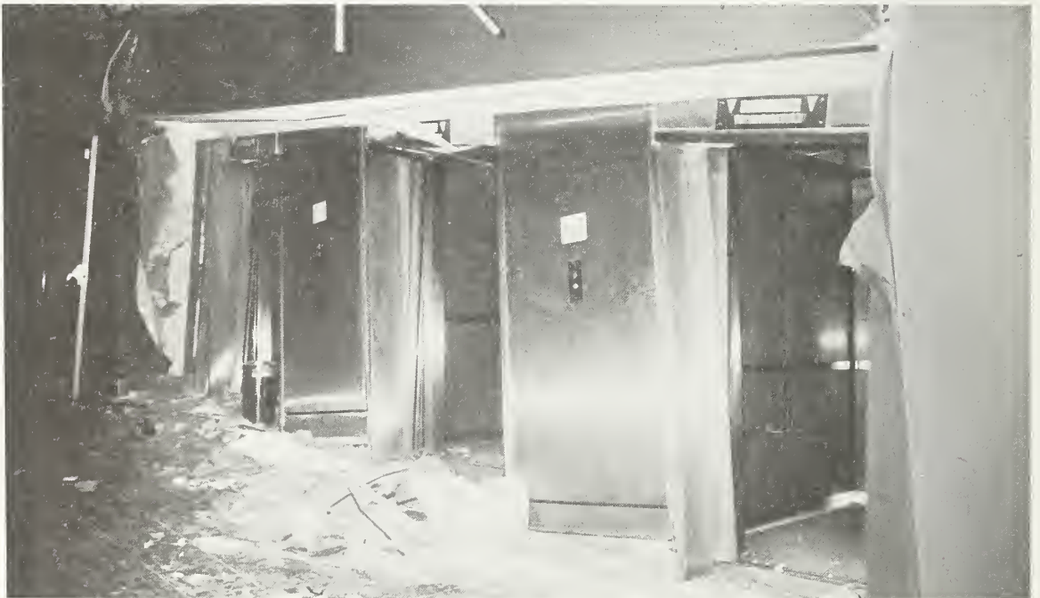
Figure 5.29 Damaged elevators in the Wing A lobby.
