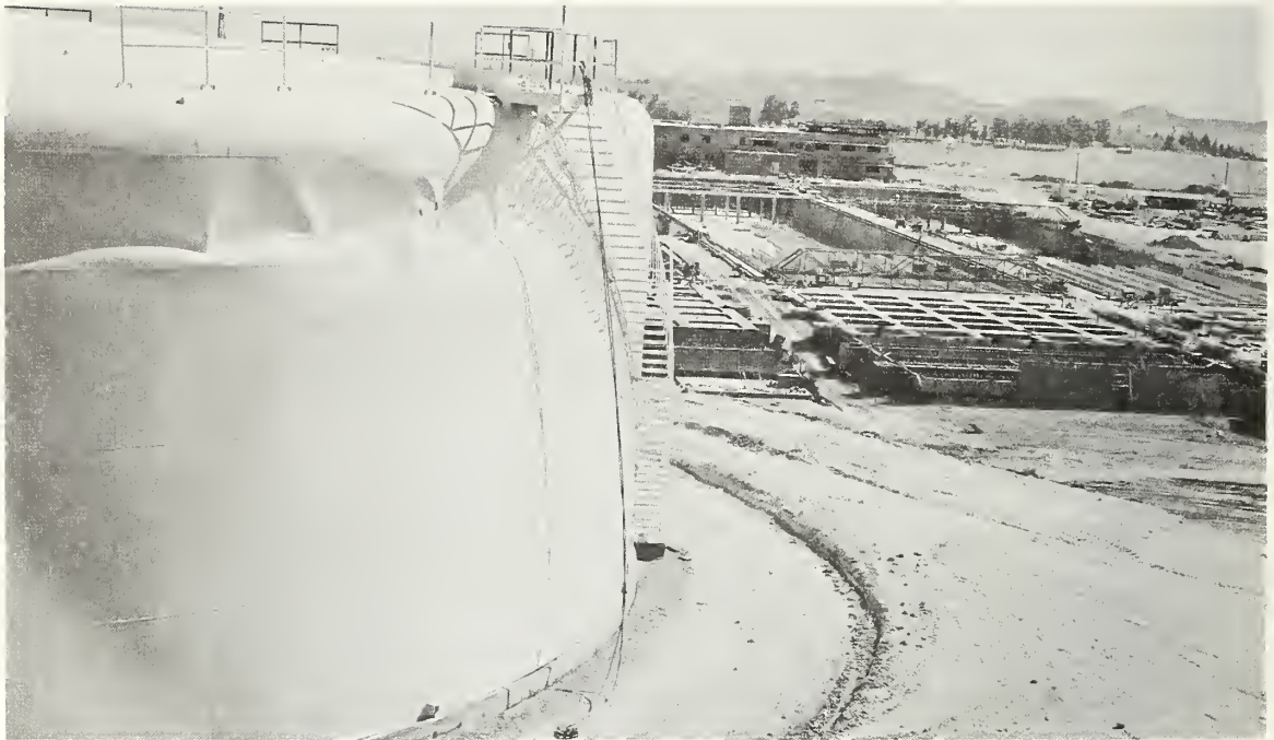
Figure 8.5 Buckled steel (3/8 in. thick) backwash tank at Joseph Jensen Filtration Plant.
