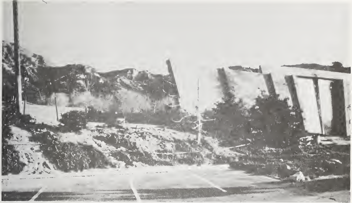
Figure 6.55 A portion of perimeter security wall has fallen; some is severely tilted, Camp Karl Holton.
