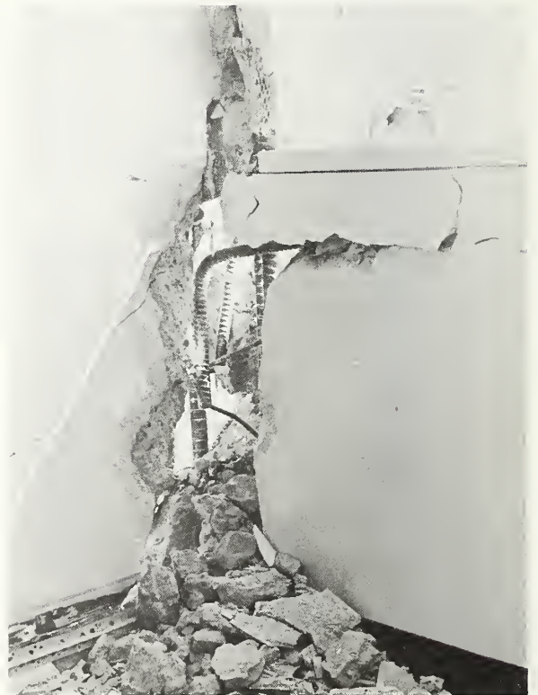
Figure 5.59 Damaged connection between the spandrel and shear wall on the southeast corner of the fourth floor.
