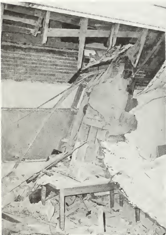
Figure 6.3 A portion of the parapet wall fell through the roof and came to rest on a table, Los Angeles High School.
