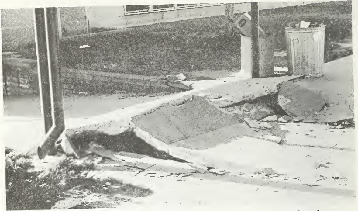
Figure 6.18 Slabs on grade were extensively cracked and buckled, Sylmar High School.
