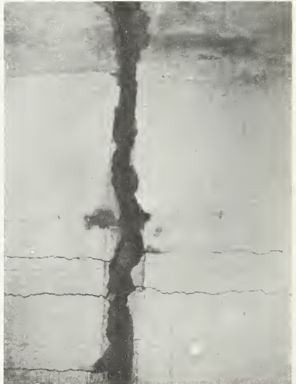
Figure 8.33 Reinforced concrete box has completely separated (4 to 12 inches) at several locations between stations 44+00 and 49+93; Wilson Canyon Channel.
