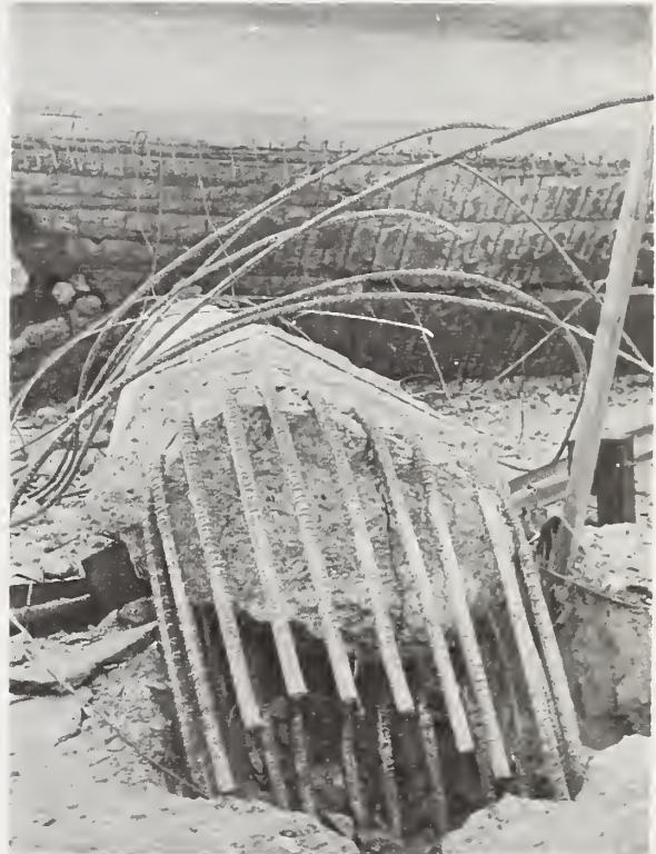
Figure 7.20 Base of the column which pulled out from the 6-ft diameter cast-in-place drilled shaft. Note the stripping of the reinforcement of the bottom of the girder in the background of the picture.
