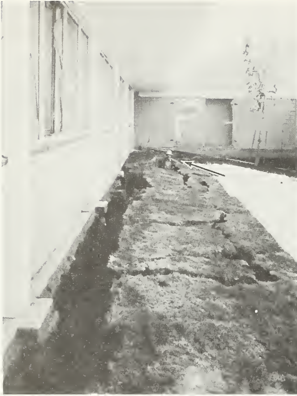
Figure 6.38 Ground crack adjacent to girls' living unit, Los Angeles County Juvenile Facility. Man standing in the crack is 6 ft 0 in tall.
