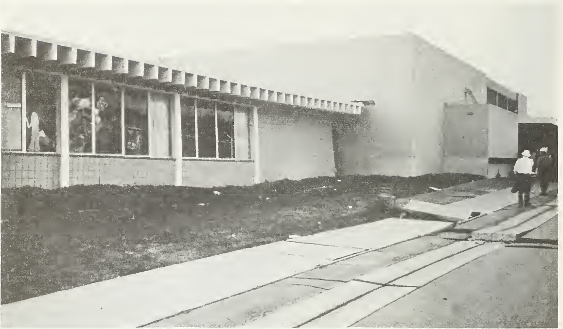
Figure 6.42 East wall of girls' school, Los Angeles County Juvenile Facility. Note distress at right (north) end adjacent to taller (cafeteria) building and ground rupture.
