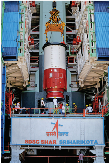
Hoisting of the nozzle end segment of PSLV-C46 first stage over the launch pedestal
