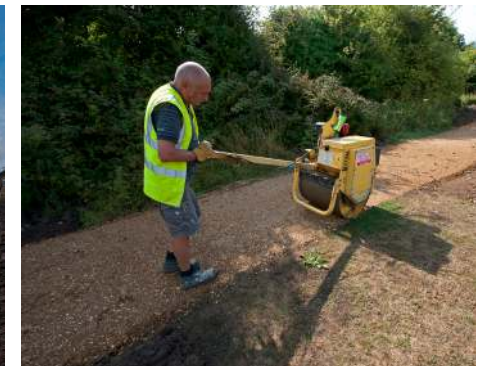
Footpath raising, realignment and resurfacing improve accessibility and limit erosion of surrounding habitats. Images: Dennis Bright
