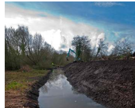
At Mansbridge Fen, an excavator clears a silted-up ditch to encourage the spread of fen vegetation
