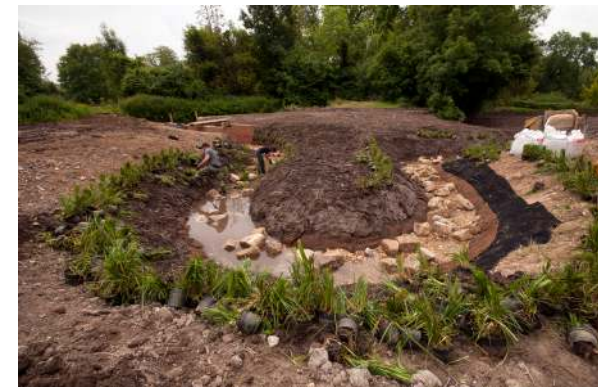
The channel being constructed bypasses Malm Lock, enabling fish to reach the habitat upstream. Image: Dennis Bright
