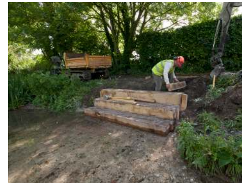
A 'Dog Dip' being constructed, to allow access to the water whilst preventing bank erosion
