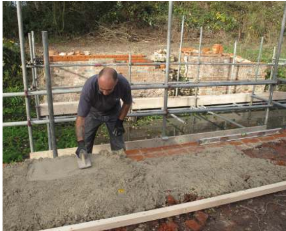
Contractors lay a bead of lime mortar to protect the restored brickwork below. Image: Dennis Bright
