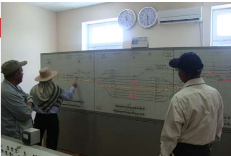
Signalling panel in Hairatan station
