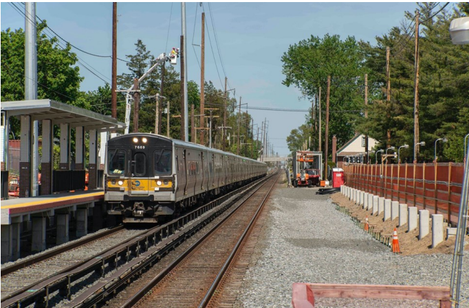
M-7 7669 (Bombardier Transportation, 6/2006) is heading Train #8055 from Ronkonkoma to Penn Station through the Carle Place station on May 17, 2020 at 3:22 in the afternoon. The ballasted area to the right is where the new third track will be laid. The platform supports for the new eastbound platform are to the right of that. On the extreme right is the temporary walkway from the existing eastbound platform to Carle Road. The temporary pedestrian access from Garden Avenue on the south side of the station to the eastbound platform is now closed due to the construction of the new overpass.
