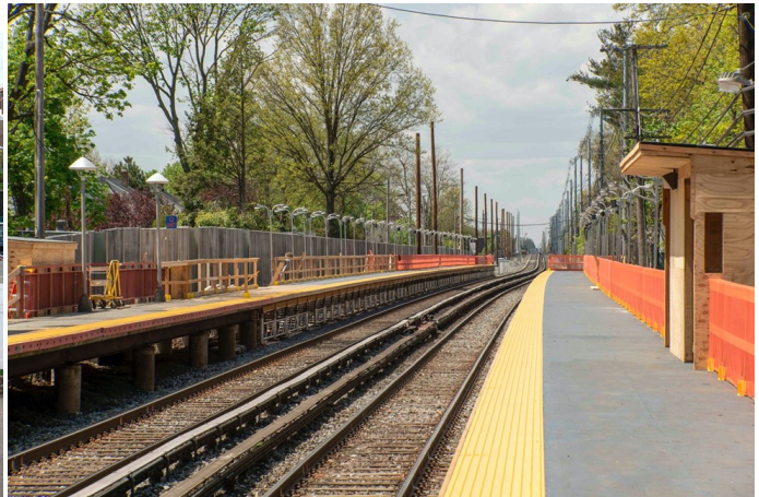
Construction is nearly complete in this view west of the temporary platform extensions at Mineola station on May 4, 2020. Note the shift in the track alignment in the distance. This was done during the Herricks Road grade crossing elimination project back in 1998.
