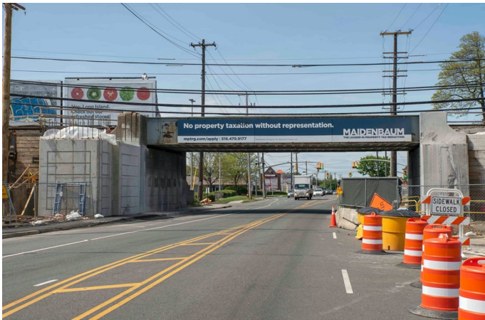
Looking north on Glen Cove Road on May 17, 2020. The west bridge abutment has already been extended while the east abutment is still being worked on.
