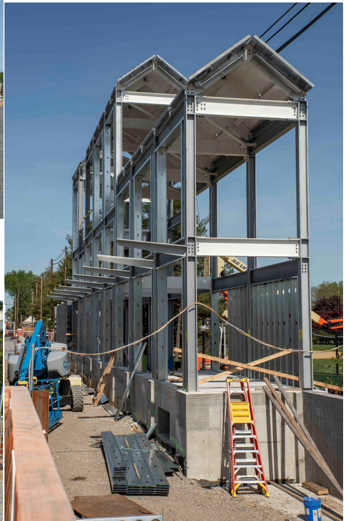
The steelwork for the south side of the future overpass, with elevator shafts, is nearing completion. Those are the canopy supports for the future eastbound platform extending out from this structure. May 17, 2020.
