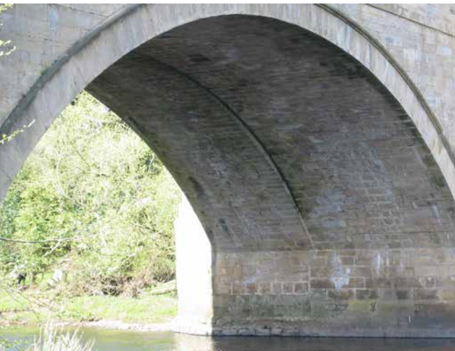
The underside of the arch and the join (left, upstream) of the single carriageway medieval bridge and the later, widened 18th century bridge, Piercebridge
