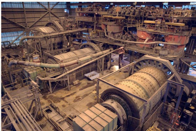
THE OK TEDI ORE PROCESSING FACILITIES COMPRISE 2 SAG MILLS AND 4 BALL MILLS
