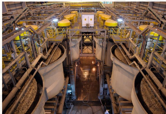
THE TAILINGS PROCESSING PLANT, PART OF THE RECENTLY COMMISSIONED MWTP
