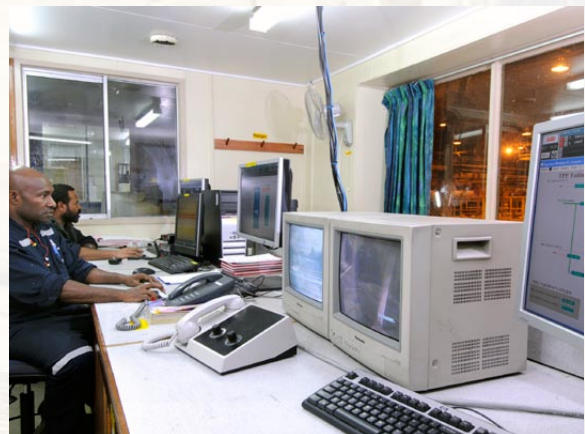
CONTROL ROOM AT THE TAILINGS PROCESSING PLANT
