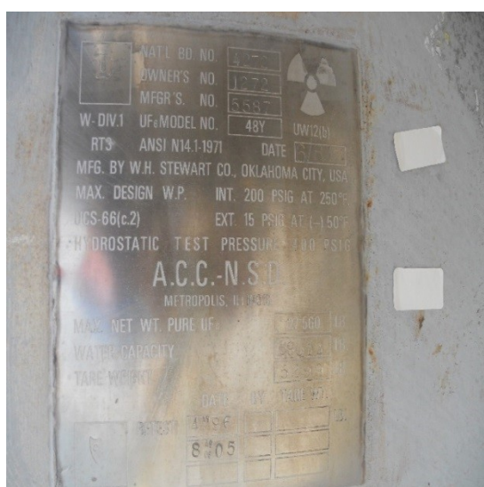
Figure B-1. Representative nameplate.
