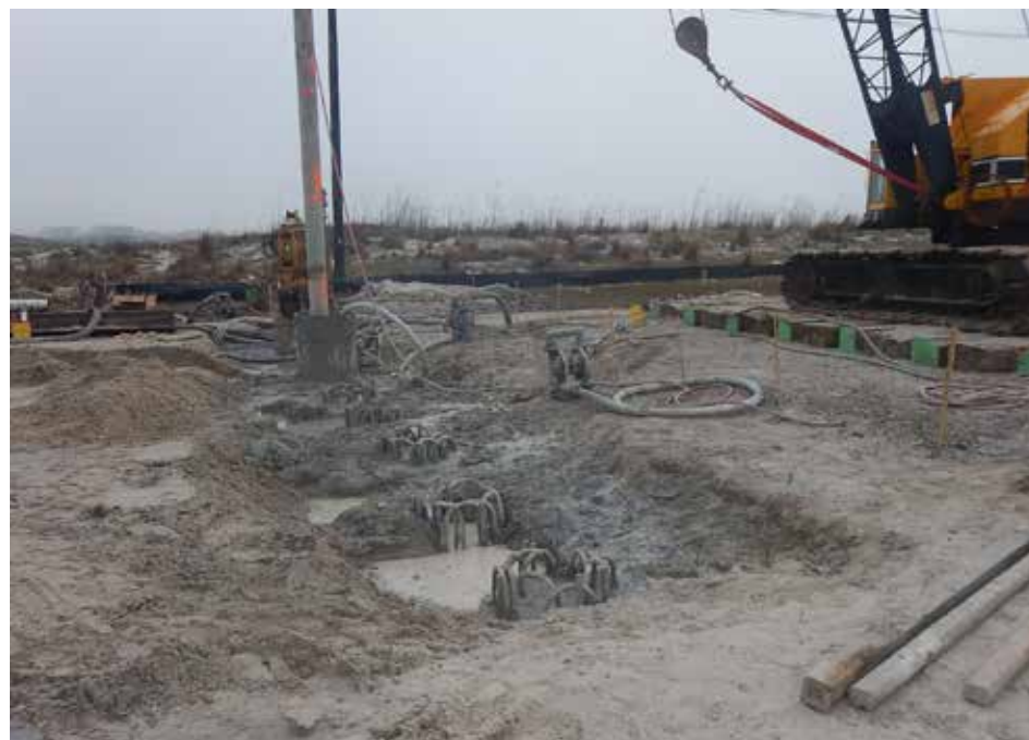
These vertical supports will be the underpinning of the bridge structure. There will be a total of 32 and several are already in place.
