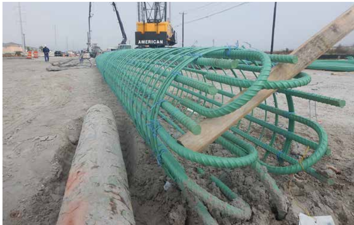
These columns of rebar will be filled with cement and support the arches that are the main portion of the bridge.
