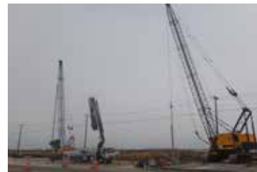
The cranes at the site are drilling the shafts for the vertical supports..
