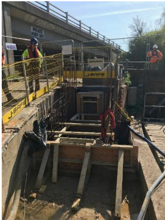
Construction underway on the Itchen counter at Gaters Mill, providing a safe side-access door as an alternative to the vertical ladder and shaft.
