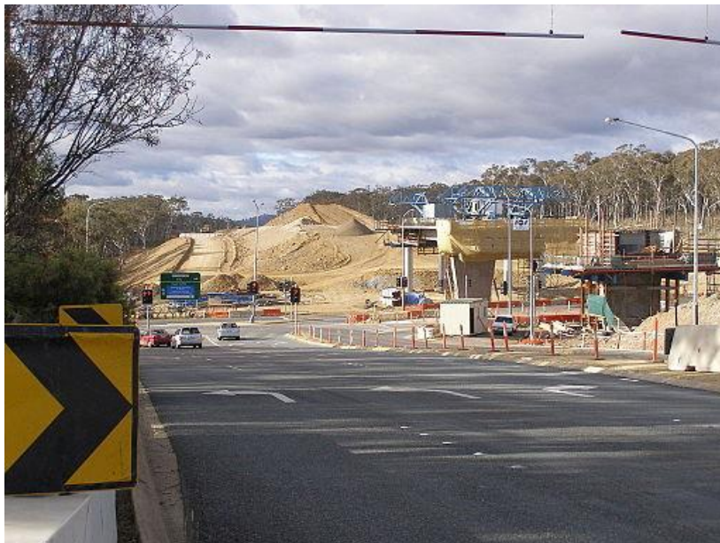
Fig. 5. Construction of the GDE at Belconnen Way and Caswell Drive. Photo: Ben McCarthy (Wikimedia Commons).
