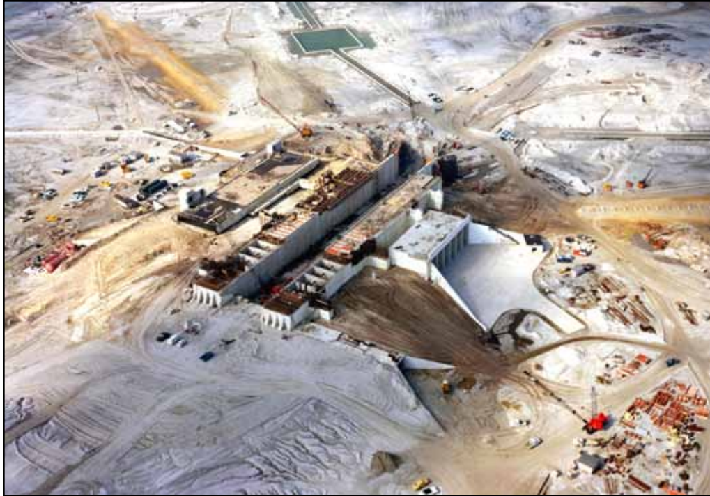
Pad A takes shape at the seaside Launch Complex 39 in December 1964. The pad hardstand contains 68,000 cubic yards of concrete.
