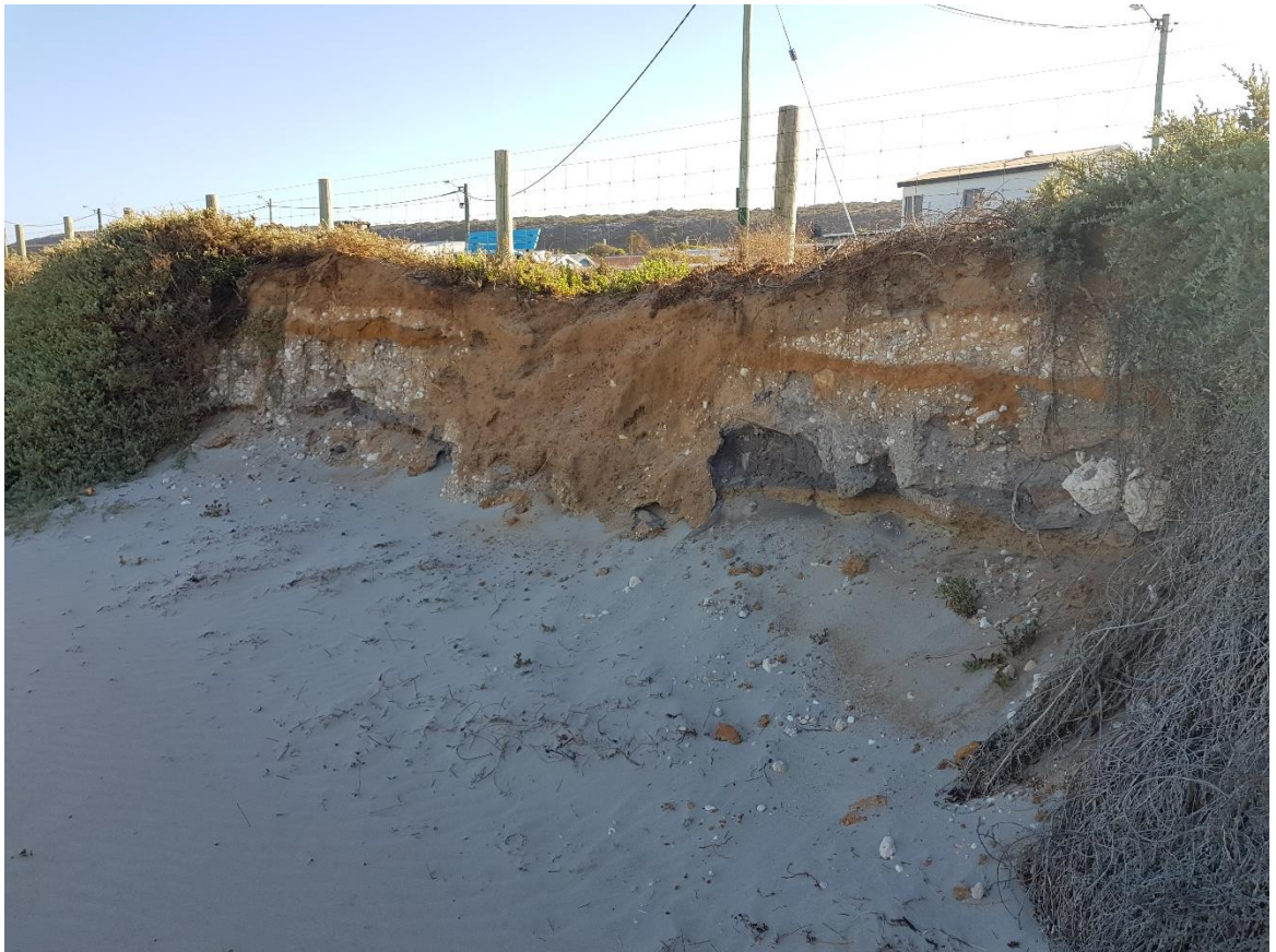
Figure 3-28 Erosion scarp threatening to undermine footpath. Northern Zone 7.
