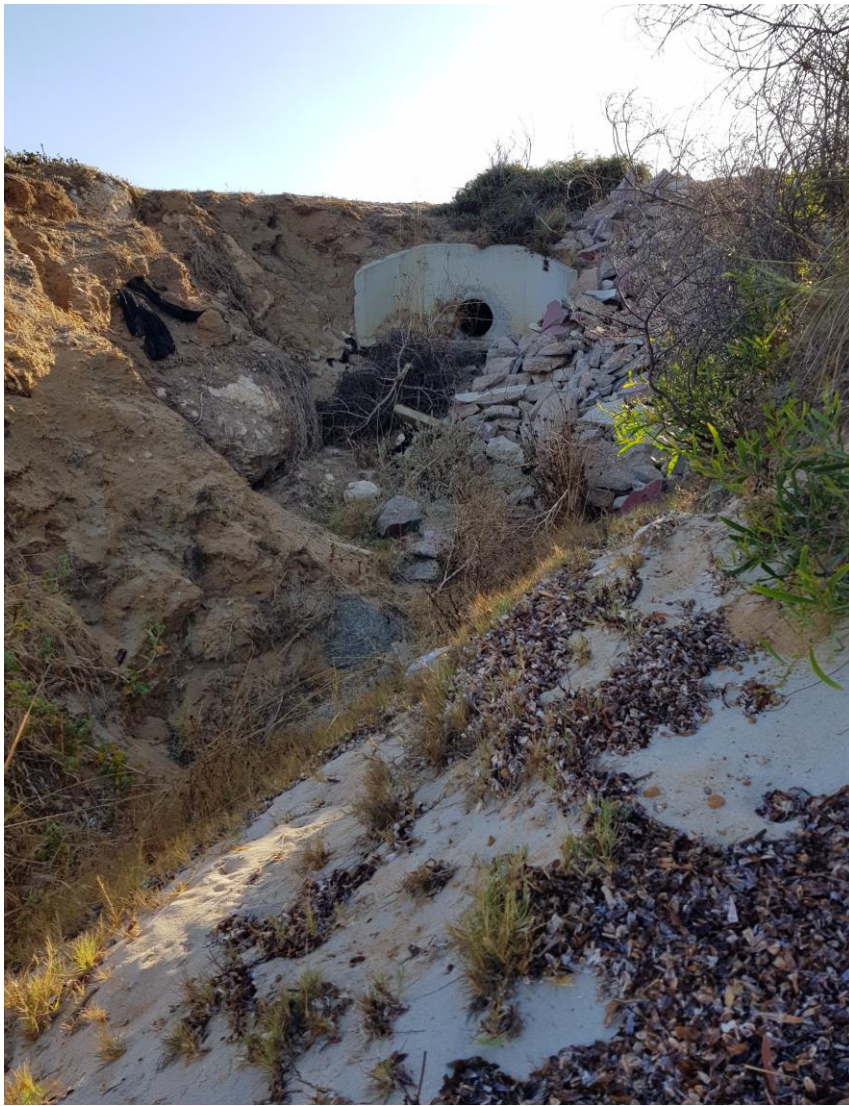
Figure 3-34 Stormwater drain in central Zone 8 causing water scour of dunes.
