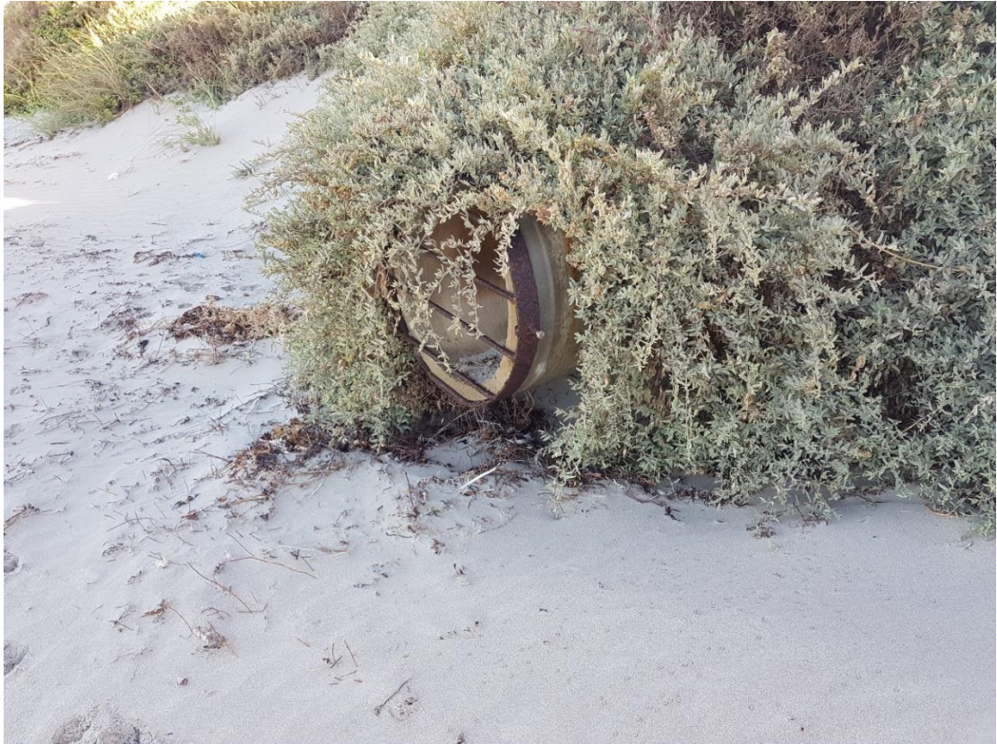
Figure 3-25 Stormwater drain obscured by vegetation near the boundary of Zone 7 and 6.
