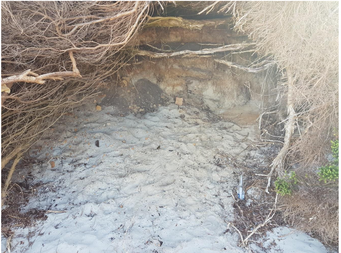
Figure 3-29 Erosion beneath vegetation, northern Zone 7.
