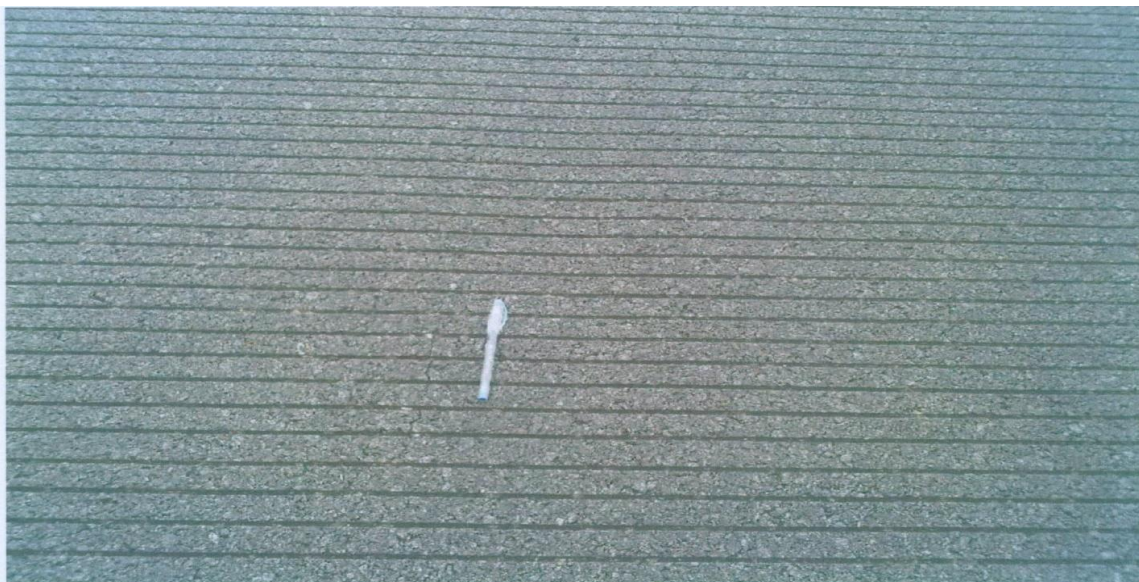
Photo No.3 Transverse grooving on the 06-24 runways (pen is to establish scale)
