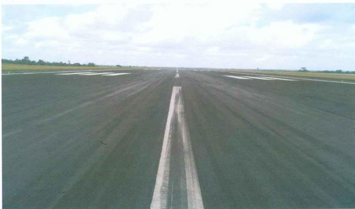
Photo No.2 shows runway 06 (Discoloration of paint markings)
