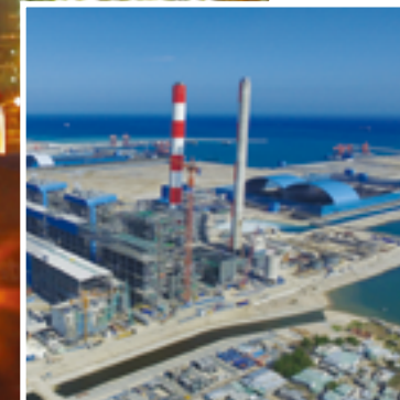
Vinh Tan 4 Coal-fired Thermal Power Plant in Vietnam
