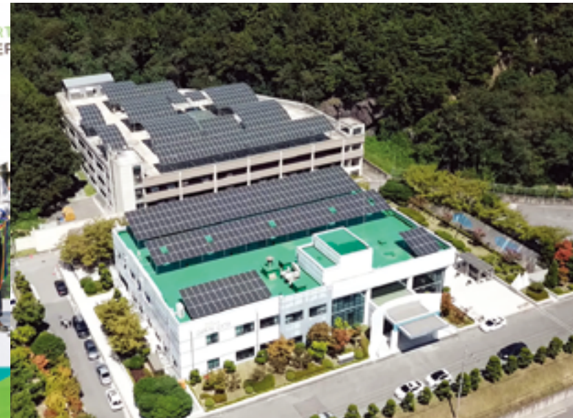
Solar ESS business
