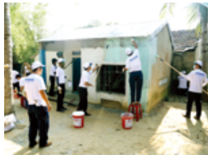
Vietnam Doosan Vina Clean houses for low-income families, House Building of Love
