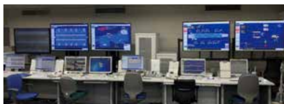
Equipment monitoring center screen
