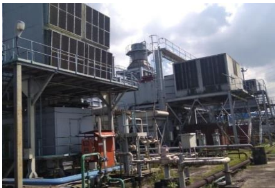
2x18.45 MW John Brown Turbines
