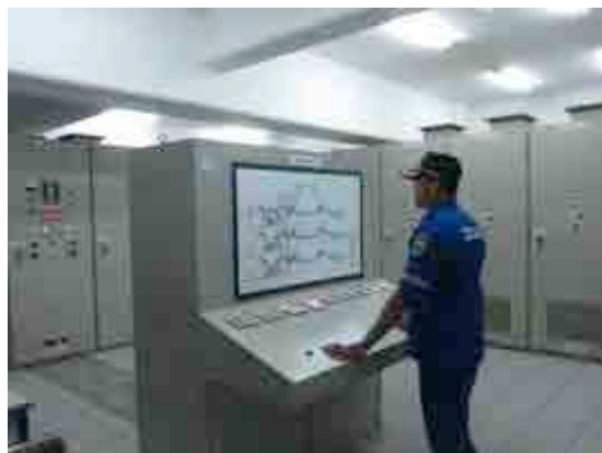
Photo 5: An operator operating the pumps at East Pump House
