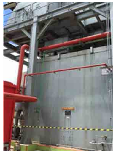
Photo 2: Generator for Gas Turbine Unit 1
