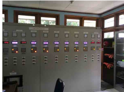
Photo 2: Water Gate Control Room of Babat Barrage
