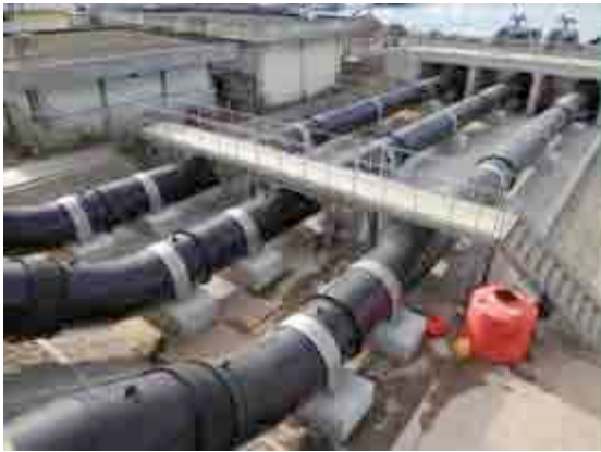
Photo 3: Pluit Pump Station Aboveground pipe line system
