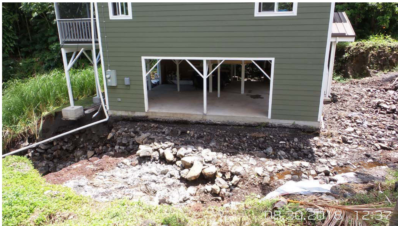
Figure 5. Flood damage to a property in Hilo on the Island of Hawaii.
