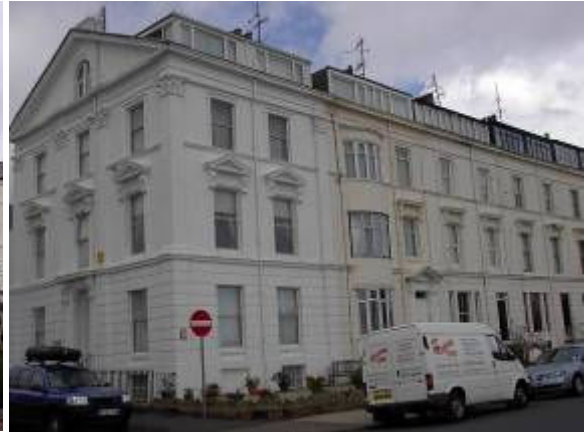
The Crescent- later dormers do not respect the architecture below and increase the dominance of the roof
