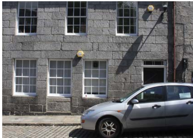
Top: Powis Lodge, 1834 south facing extension Bottom: College Bounds, blocked doorways forming new window openings
