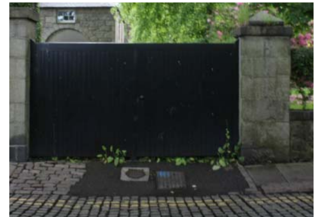
Poor condition of the granite setted roads
