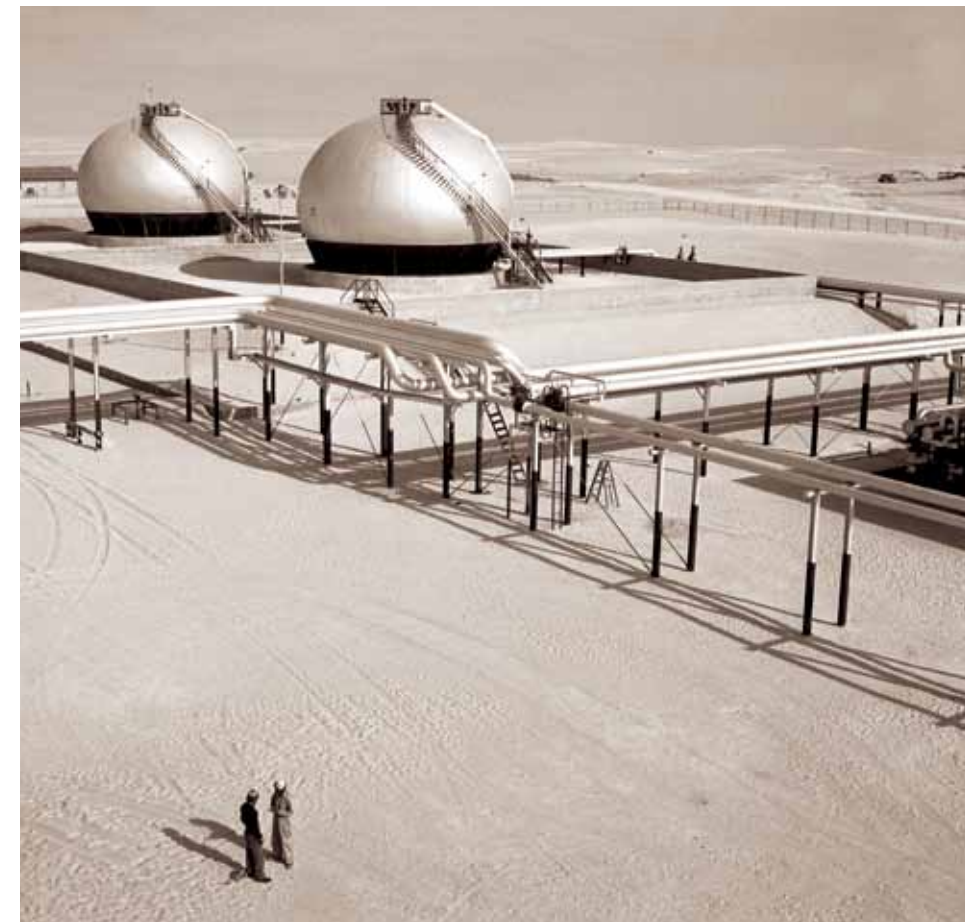
The gleaming spheroids of Abqaiq’s northern Buqqah plant, shown here in 1952, provided a key link in the process of separating natural gas from crude oil before the oil was stabilized for shipment.
