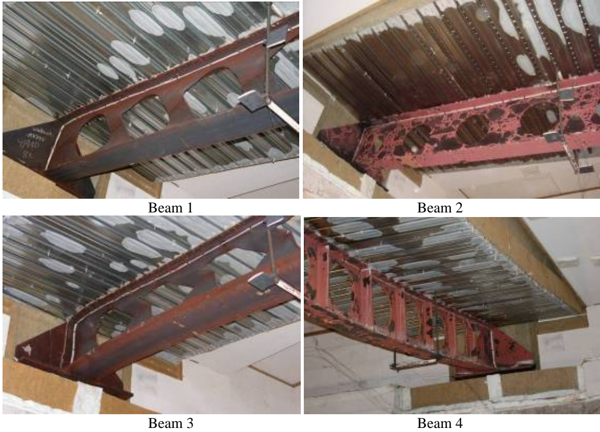
Figure 0–3 : Deformed beams in their RHS zone
