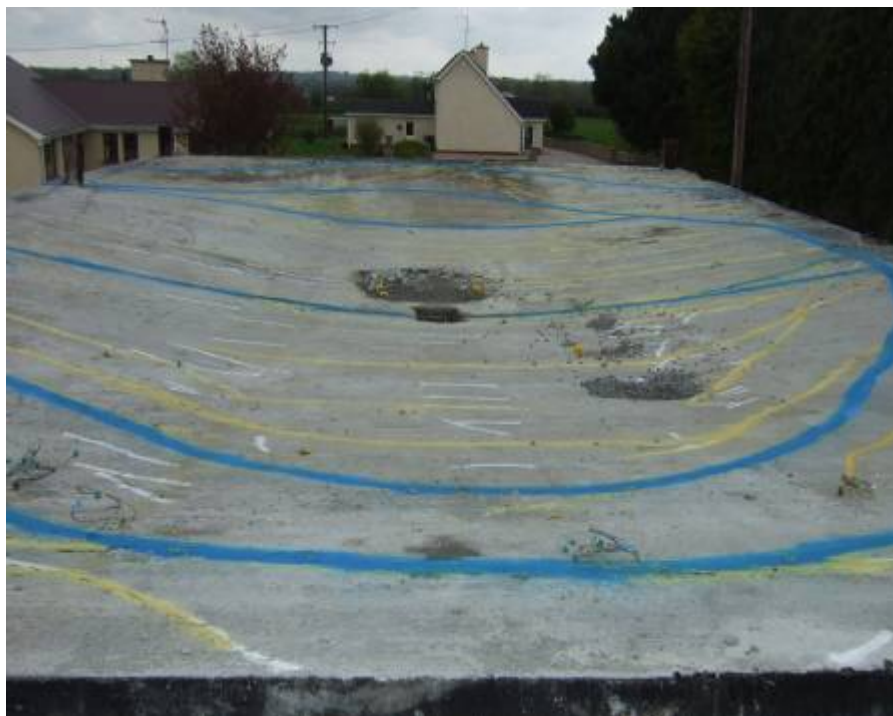
Figure 8-42 : Crack distribution on the slab
