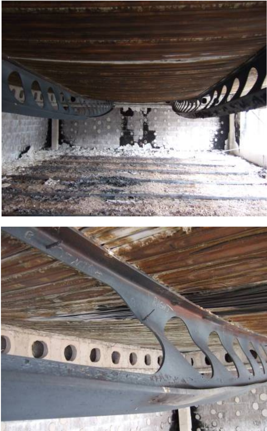
Figure 8–41 : Deflection of the slab/unprotected beam: post web buckling and lateral torsion effect.
