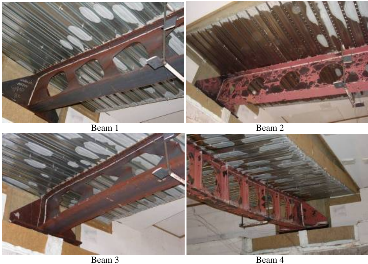
Figure 10–1 : Deformed beams in their RHS zone
