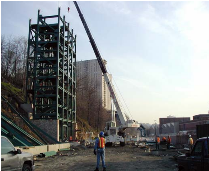
The structure that will actually join 9 th Street in Hoboken with Congress Street in Jersey City on the bluff above is taking shape. Because of the need to allow access for construction equipment, the track area has not yet received attention. The northbound platform for the station can be seen behind the crane.
