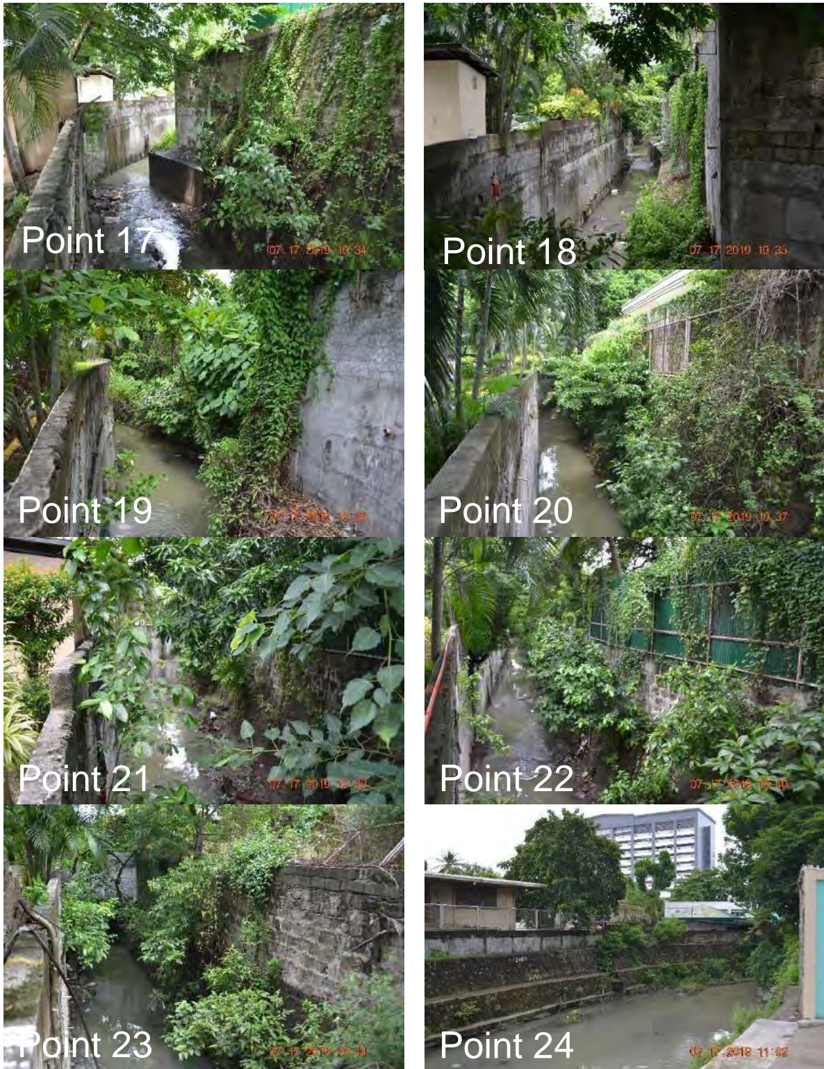
Plate 3.2-5 Site Photographs of each Survey Point Across the Channel of Maricaban Creek (Point 17 to Point 24)
