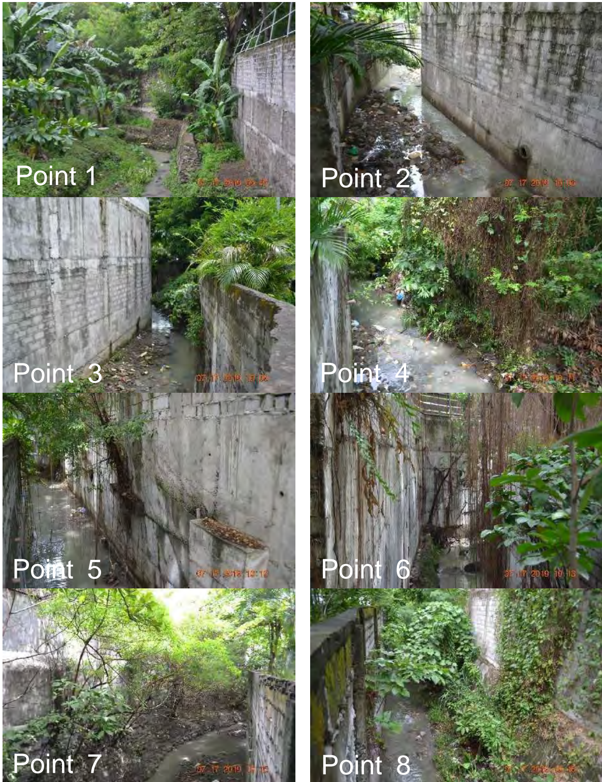
Plate 3.2-3 Site Photographs of each Survey Point Across the Channel of Maricaban Creek (Point 1 to Point 8)
