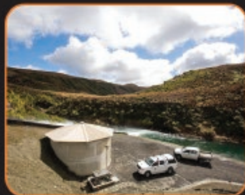
MANGAIO POWER STATION (2 MW)
