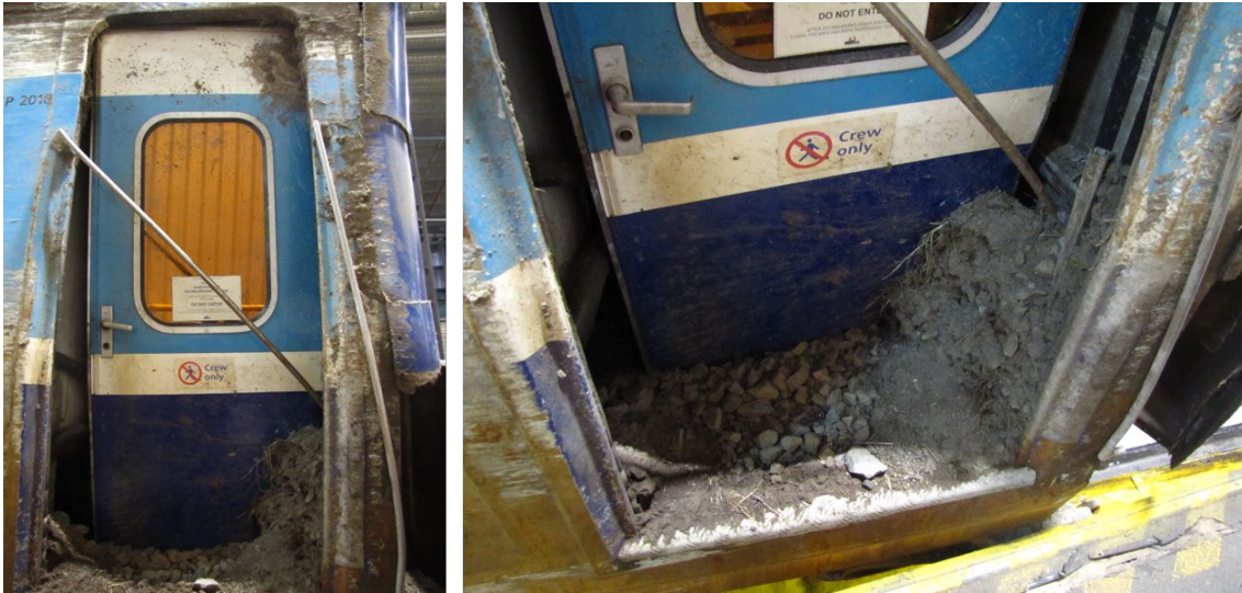
The left photograph shows a full view of the rear left-side door of XP2018, and the right photograph the base of the door pushed-in by track ballast and dirt. Source: ATSB
