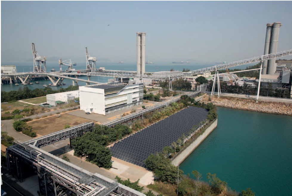
TFPV modules at the Lamma Extension
