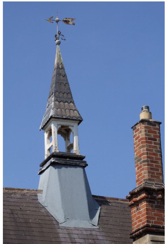
The bell tower 'fish-scale' lead-work in the form of a flèche to the roof of the former Belgrave School.
