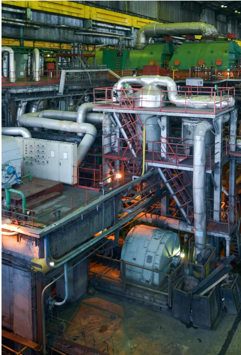
Aksu Power Plant
