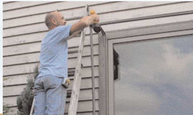
Affix the frame to the exterior of your house. The author's wooden window frames made installation easy.
