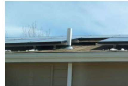
This example was rated a "2" because the array was installed too close to vent.
