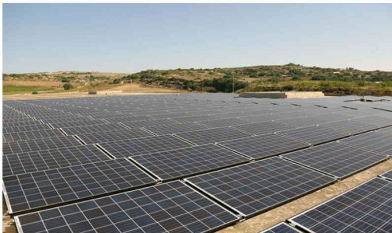
Fig. 1: More than 3,500 photovoltaic panels were installed on Tal-Fiddien Reservoir.
