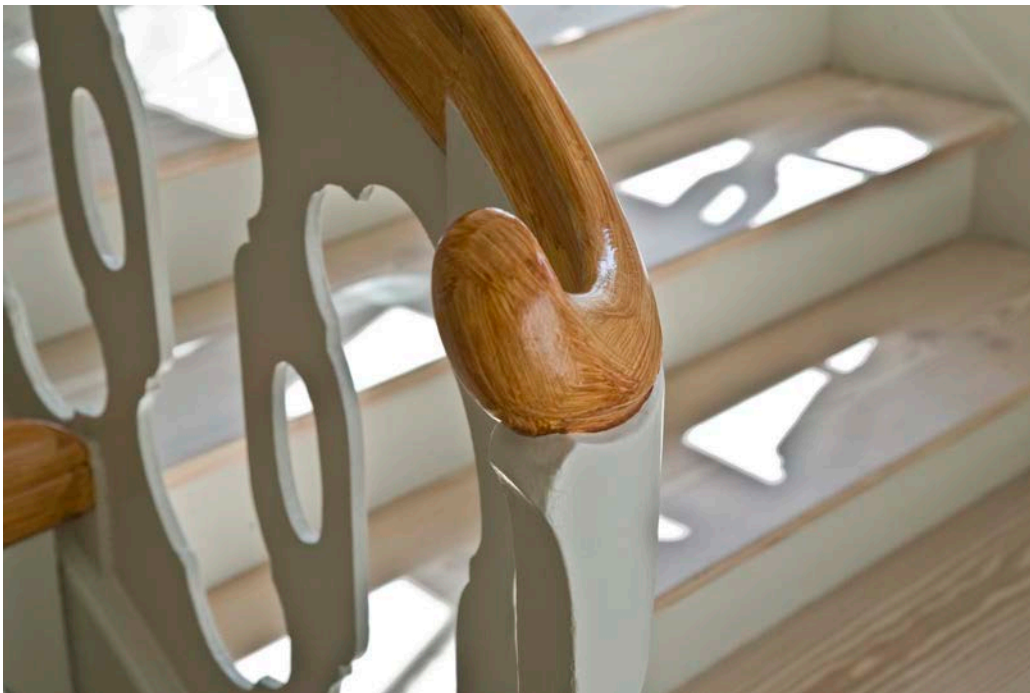
2.61 Joinery detail from the staircase in the Sisters' House, Nørregade 14 in Christiansfeld.
