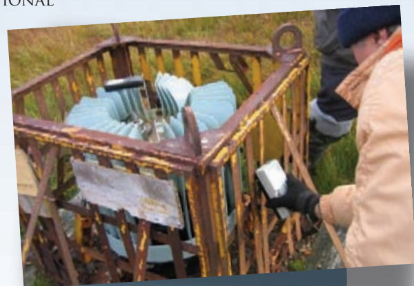
SAFETY CHECK ON A DAMAGED UNSECURE RTG, SEPTEMBER 2005
