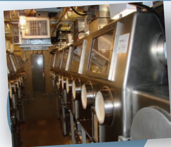
MOBILE GLOVEBOX FOR PLUTONIUM HANDLING
