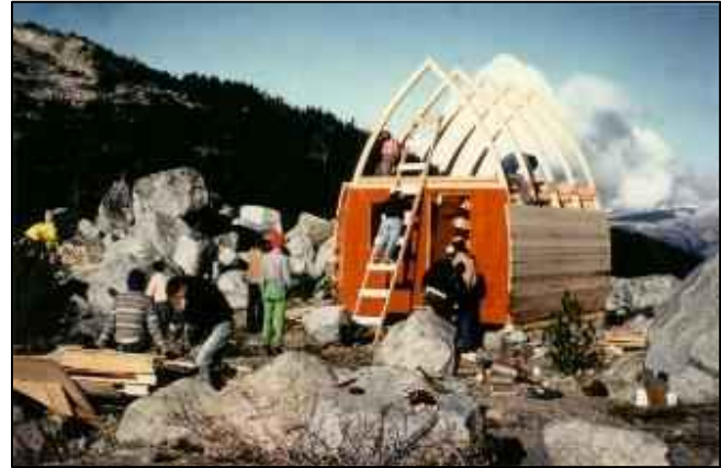
The hut under construction at its destination. Picture taken by Jay Page.
