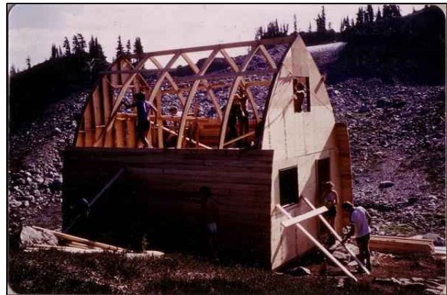
The original Brew Hut I, under construction in 1982. The Hut was destroyed by snow creep
