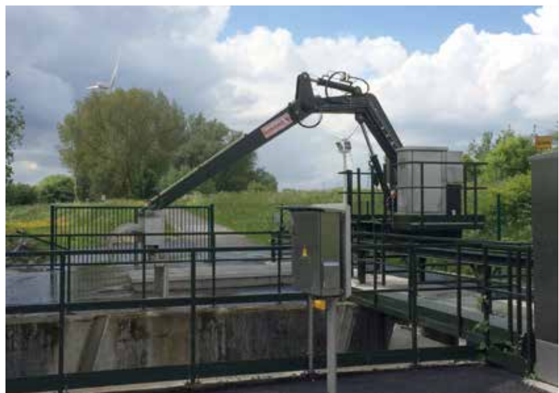
Automatic Trash Rack - Crane Type - Hemiksem (Belgium)
