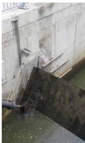
Steel construction, electromechanical and hydraulic equipment of weir at Zandbergen (Belgium)
