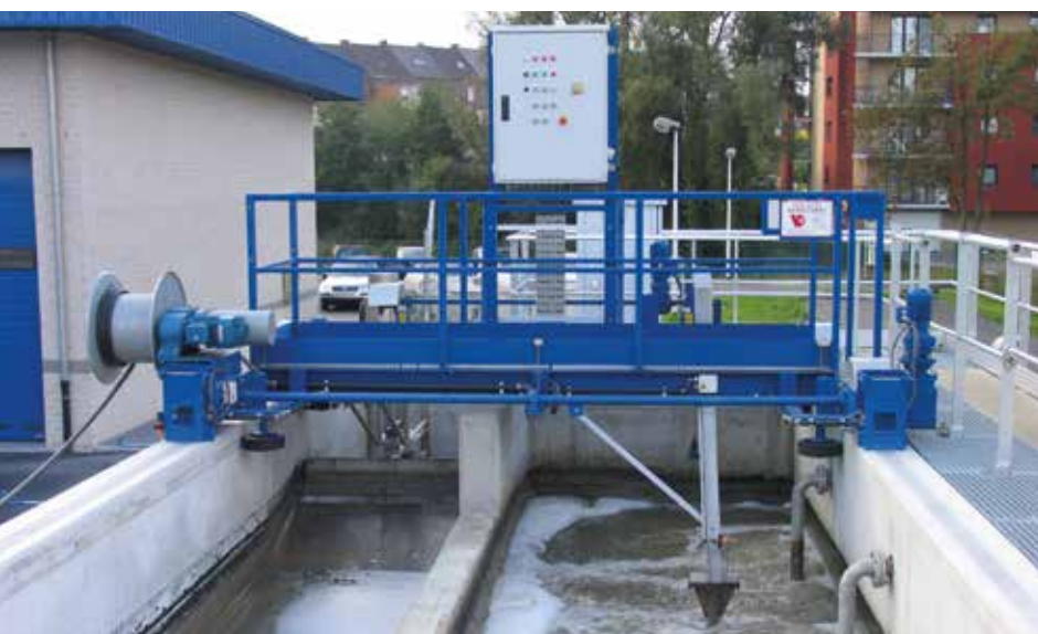
Rectangular grit and scum remover with airlift system - Step Tubize (Belgium)
