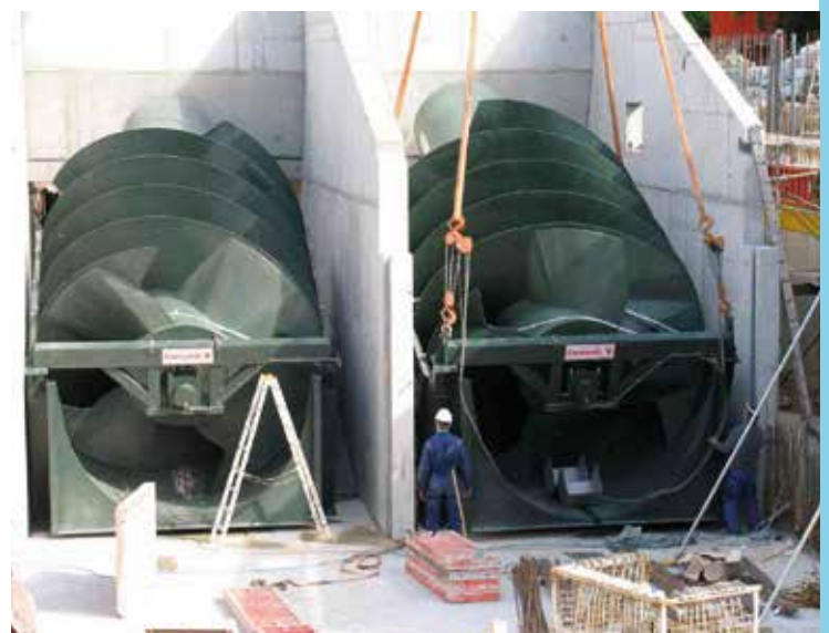
Hydro power screws with steel trough for casting at Kochehr Hofratsmühle in Künzelsau (Germany) - 2 screws - 132 kW - 8,95 m 3 /s - Screw diameter 4,1 m - Bladed length 4,8 m
