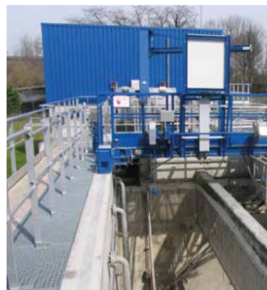
Rectangular grit and scum remover with airlift system - Step Tubize (Belgium)
