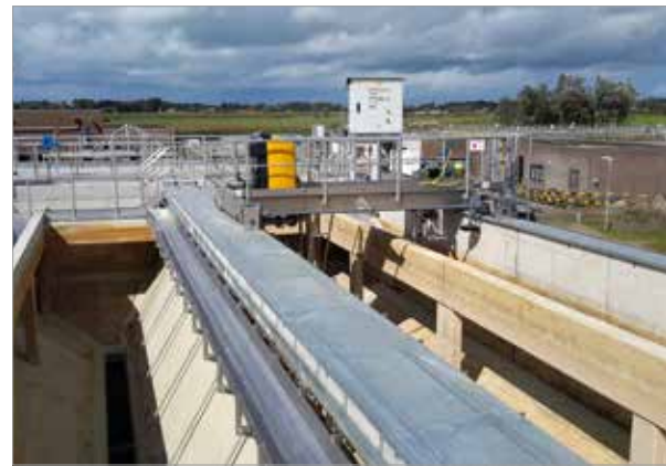
Rectangular grit and scum remover with airlift system - RWZI Wulpen (Belgium)
