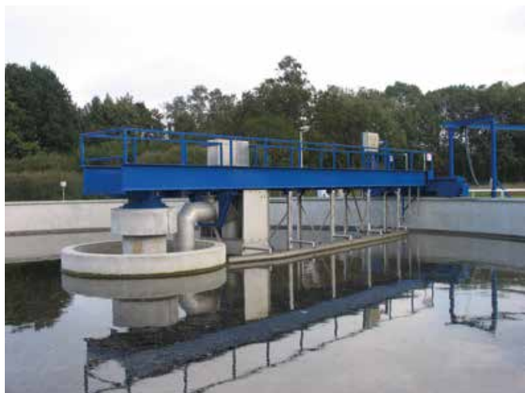
Scraper bridge Steel profile - Step Tubize (Belgium)
