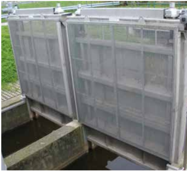
Steel construction and electromechanical equipment of shut off valve at Woumen Stenensluisvaart (Belgium)
