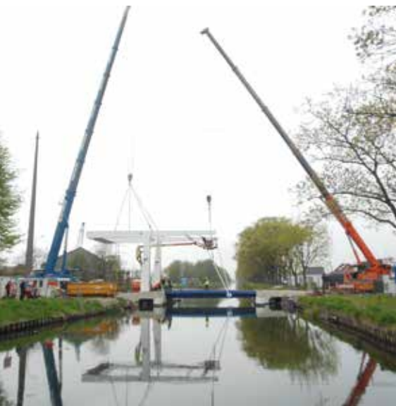
Electromechanical and Hydraulic equipment Bridge 5 in Beerse (Belgium)
