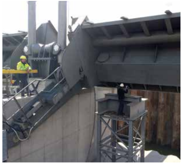
Electromechanical equipment of weir at Lock Harelbeke (Belgium)
