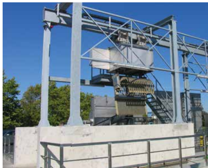
Automatic trash rack - Overhead transfer type - Woumen (Belgium)
