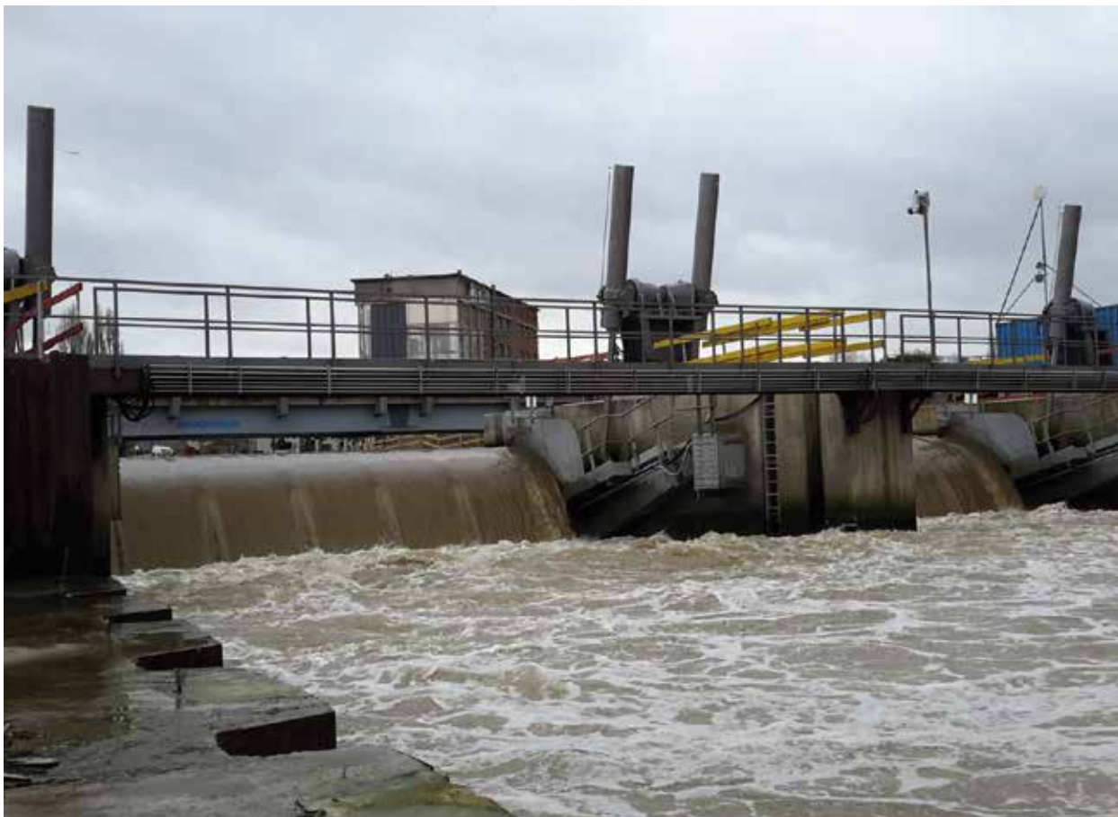
Electromechanical equipment of weir at Lock Harelbeke (Belgium)
