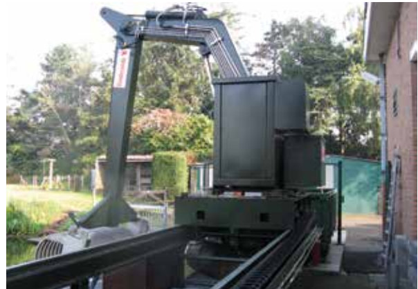
Automatic Trash Rack - Crane Type - Ertvelde (Belgium)
