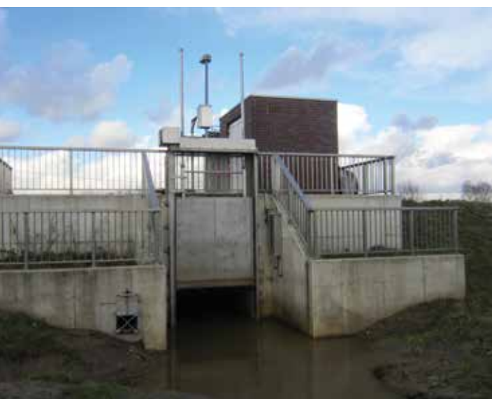
Steel construction and electromechanical equipment of shut off valve at Zandbergen (Belgium)
