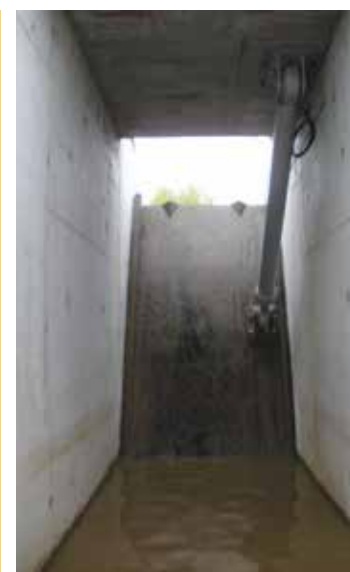
Steel construction, electromechanical and hydraulic equipment of weir at Zandvoorbrug (Belgium)
