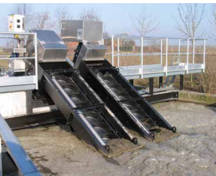
Compact screwpumps at RWZI Poperinge (Belgium)
