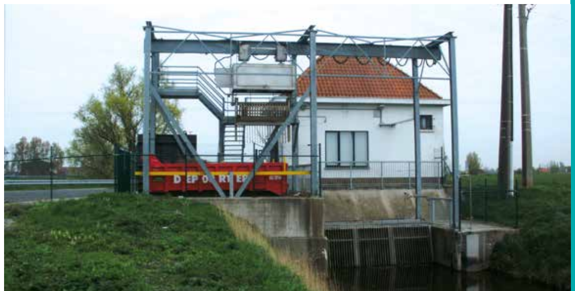
Automatic trash rack - Overhead transfer type - Woumen (Belgium)
