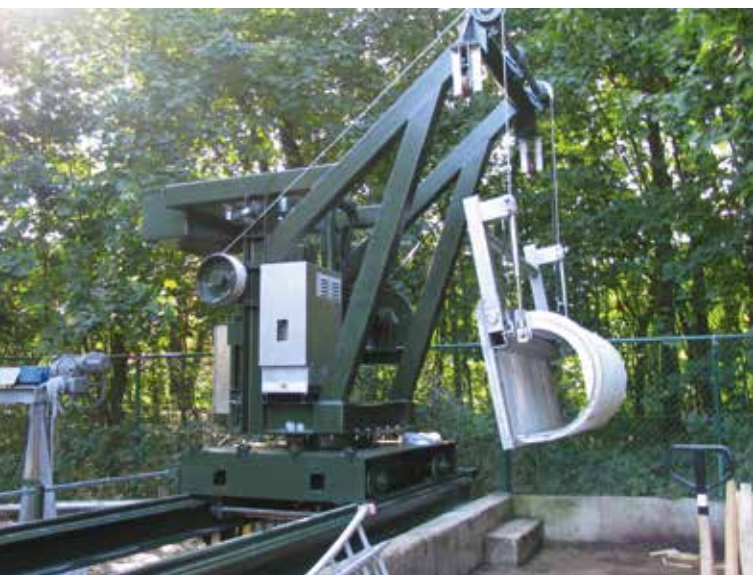
Automatic trash rack - Hybrid type - Brugge (Belgium)
