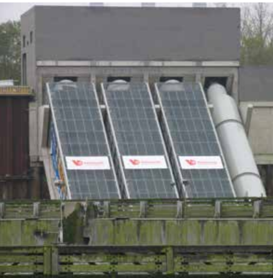
Compact screwpumps/ hydropower screws on the Albert Channel in Ham and Olen (Belgium) - 6 screws - 780 kW pumping operation - 360 kW generating operation - 5 m 3 /s - Screw diameter 4,3 m - Bladed length 21,6 m
