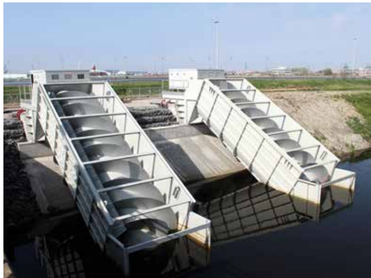
Compact screwpumps on the Leopold channel at Zeebrugge (Belgium) - 2 screws - 315 kW - 5 m 3 /s - Screw diameter 3,7 m - Bladed length 10,6 m
