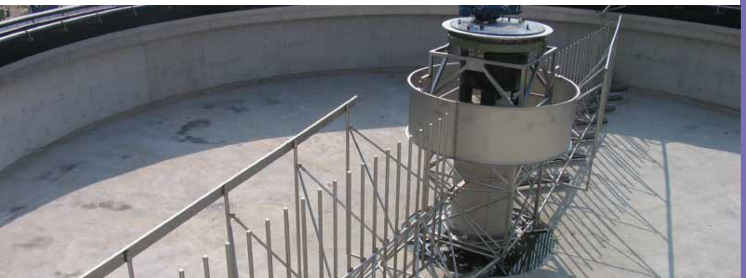
Sludge thickener RWZI Amsterdam West (Netherlands)
