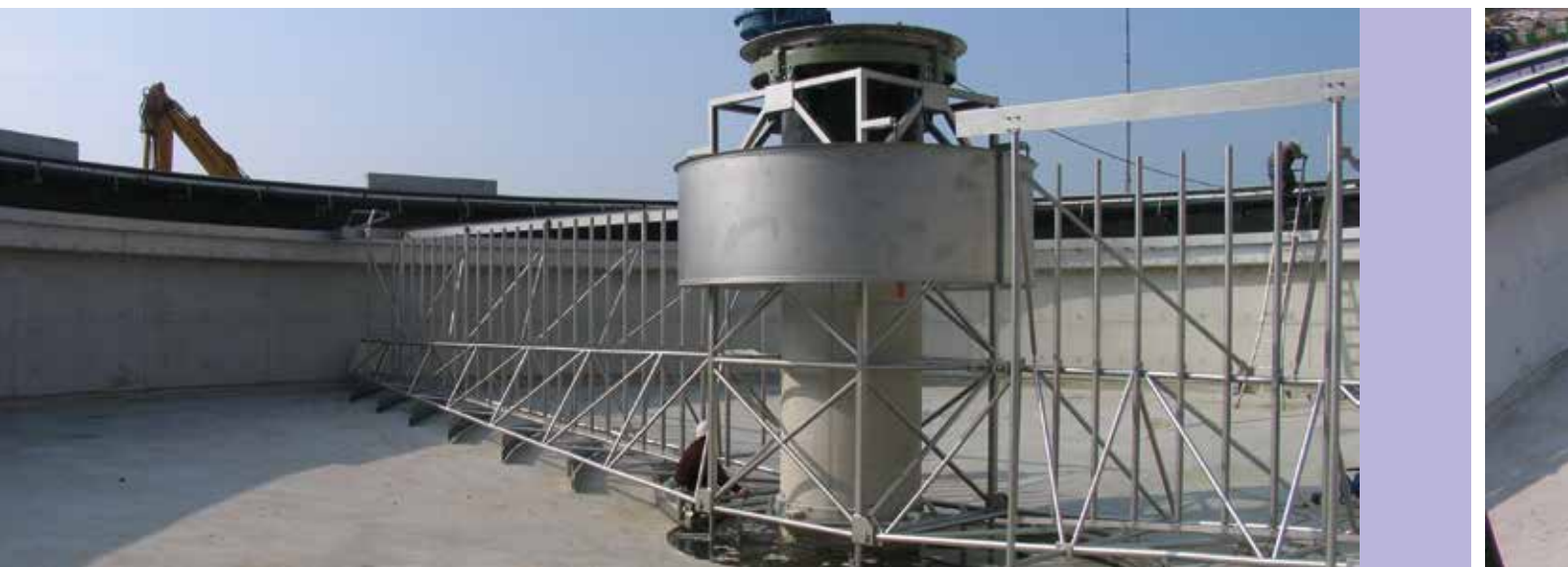
Sludge thickener RWZI Amsterdam West (Netherlands)
