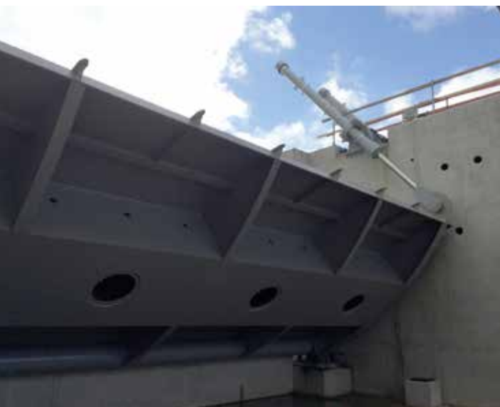
Electromechanical and Hydraulic equipment of weir at Lock Kain (Belgium)
