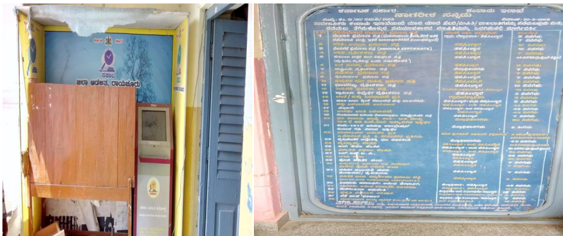
Pic. 6. Damaged Kiosk and SAKALA Board at DC office Raichur
