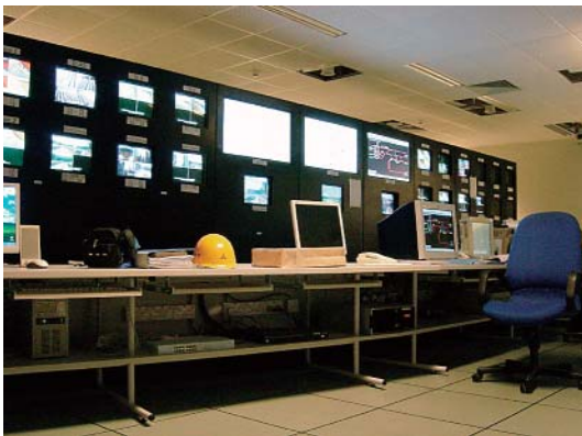
Fig. 3 Main operation control center
