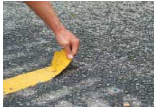
Figure 4. High Severity Wear Non-Patterned Tape Lane Marking.
