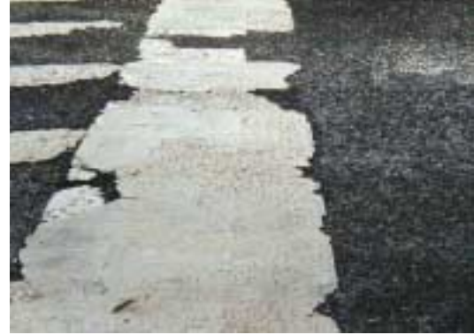
Figure 2. High Severity Wear Thermoplastic Lane Marking.
