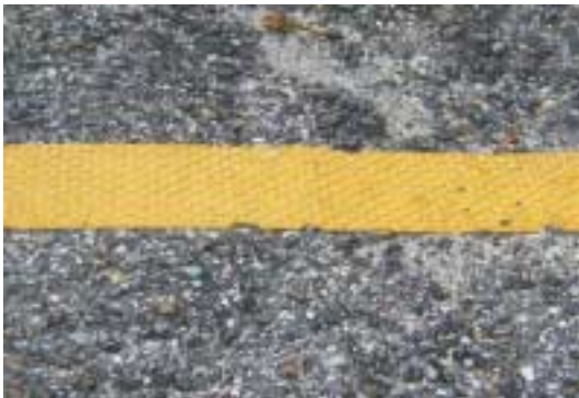
Figure 3. Medium Severity Wear Patterned Tape Lane Marking.
