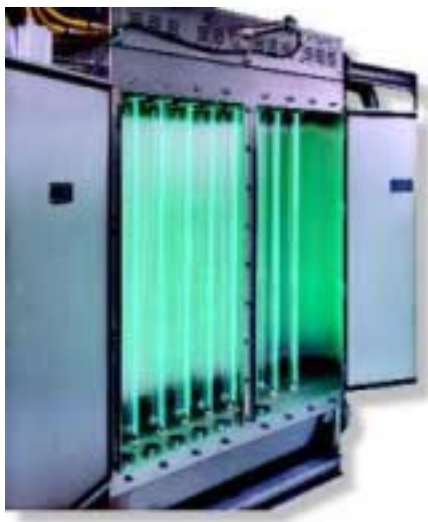
Figure 4. Interior of 650-scfm PPCU Module (Lights “On” and No “Socks”).
