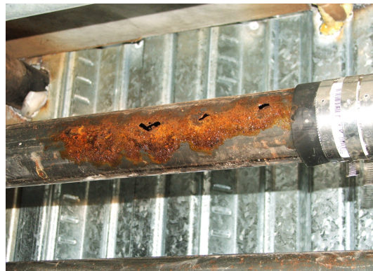
Figure 4 – Results of a Dry-Pipe Fire Sprinkler System. Photo: CDCR
