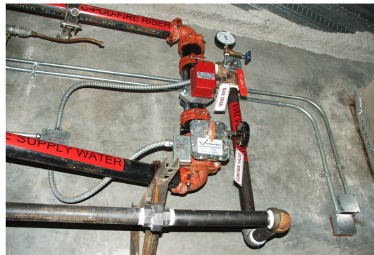
Figure 5 – After Conversion to Wet System. Photo: CDCR
