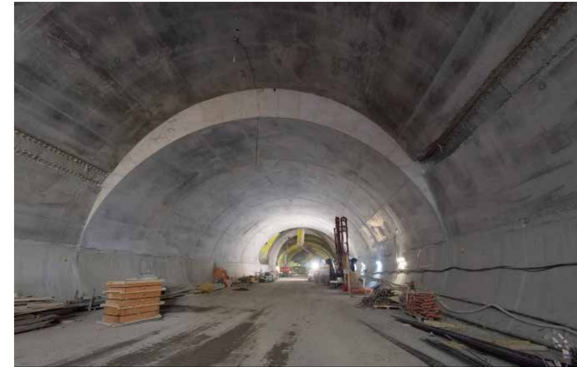
This view shows the mining at Laird Station, with completed sections of floors and roof archway.
