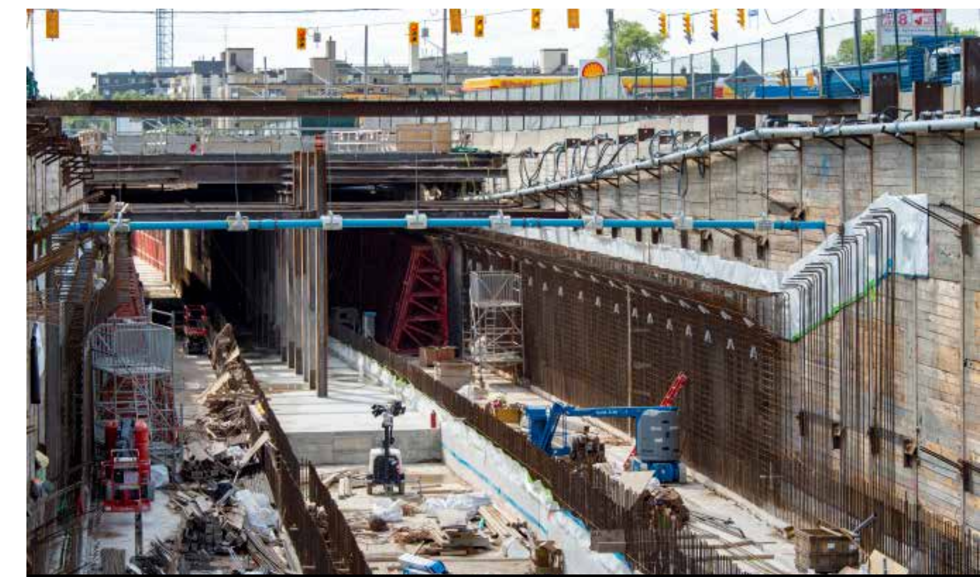
This view is looking under the Kennedy and Eglinton intersection, with formwork in place for more concrete pours.
