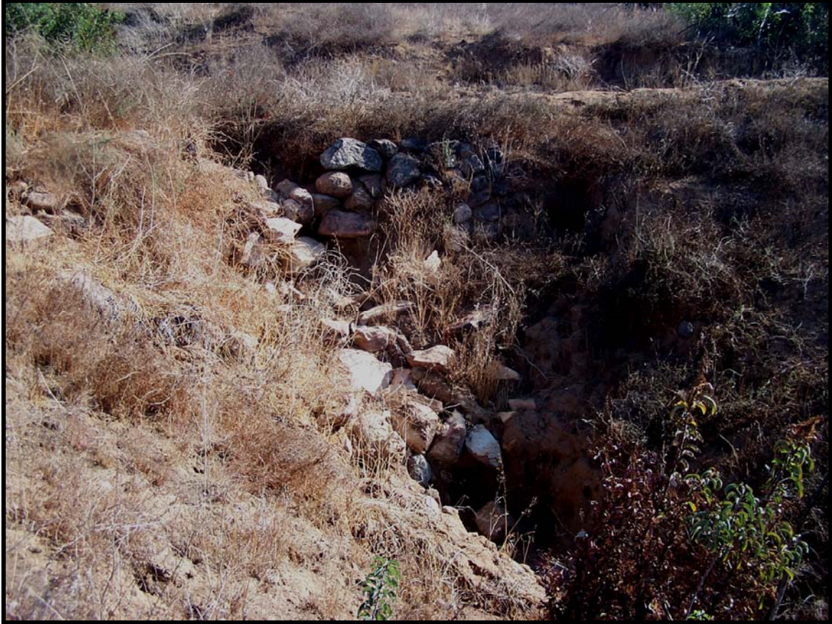
Figure 10: A dry masonry retaining wall reinforcing the old road bed where it crosses a small drainage.
