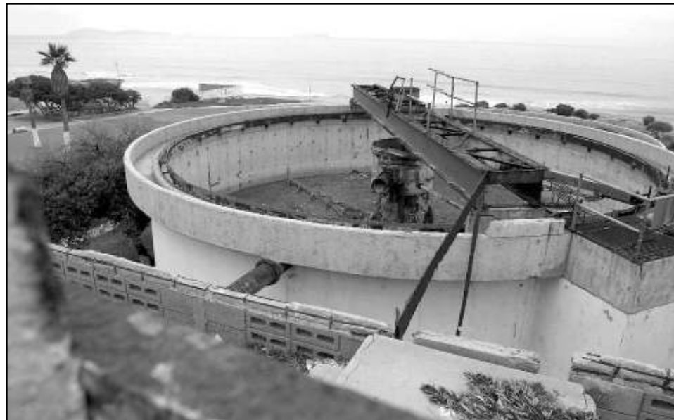
Playas de Tijuana sewer pump station
