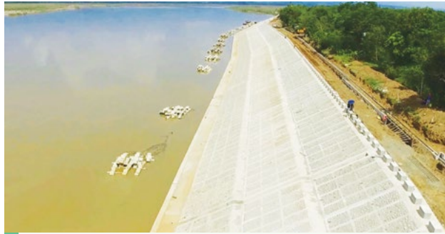
The Flood Risk Management Project for the Cagayan River to address serious bank erosion was completed in November 2019.
