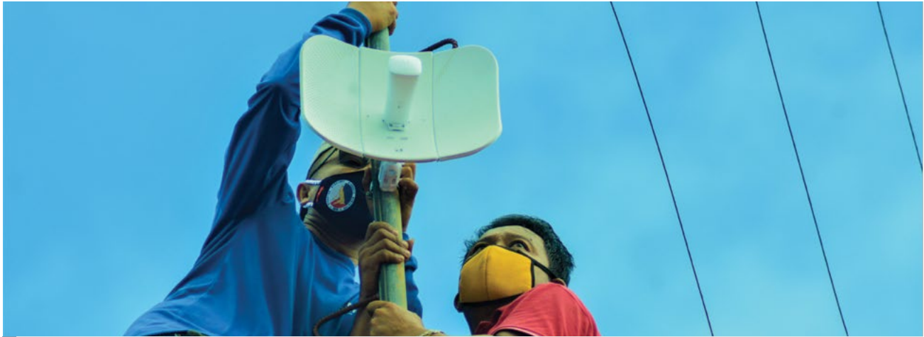
Installation of “Free Wi-Fi for All” Tower amidst the new normal
