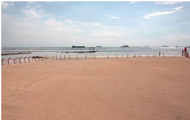
The beach nourishment project along Manila Baywalk is being undertaken to prevent coastal erosion and increase beach width.
